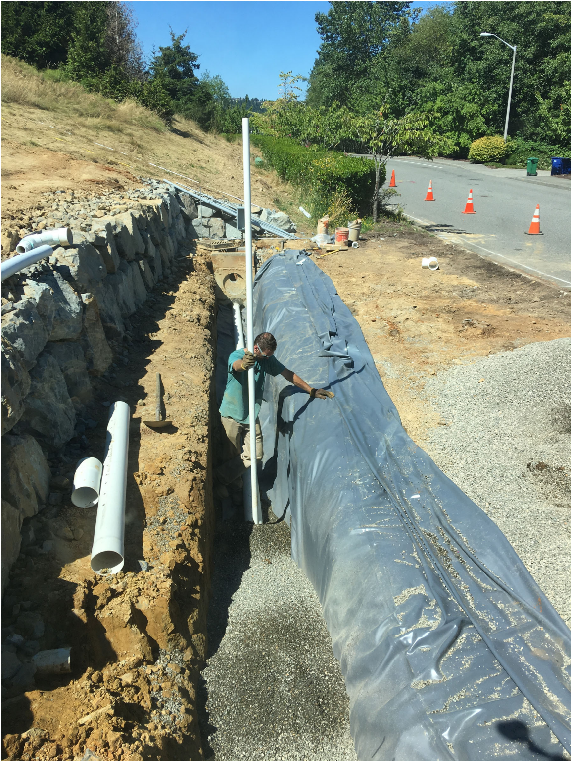
Gravel Backfill of Interception Trench (note rock wall drain pipe in lower left corner)
