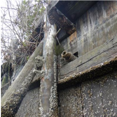
Pipe Q1 (4-inch steel) and Q2 (8-inch steel)
