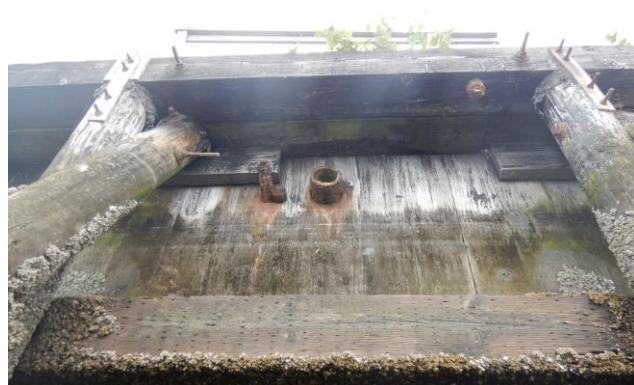
Pipes P (6-inch steel) and Q (2-inch steel)
