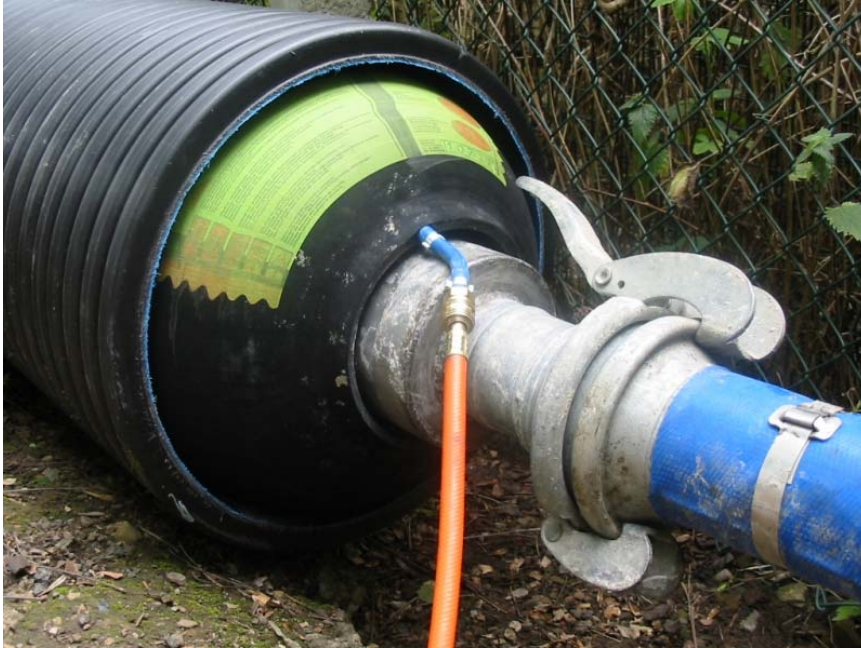
Photograph 3. Pipe Plug with Bypass
