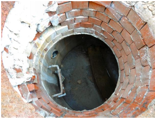
Lateral Pipe Entering City CSO Line at Easternmost Manhole on K-C Property
