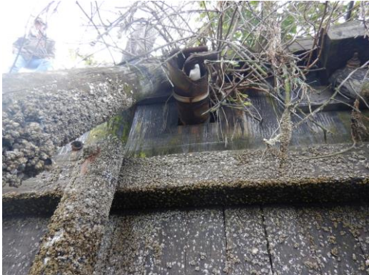
Pipe Q3 (2- and 1-inch steel, inside 12-inch casing)
