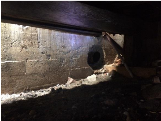
Pipe E (8-inch steel)
