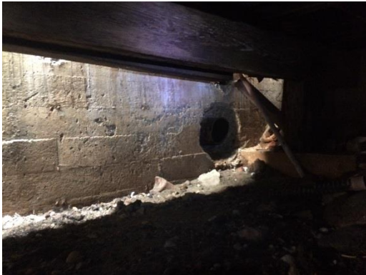
Pipe E (8-inch steel)
