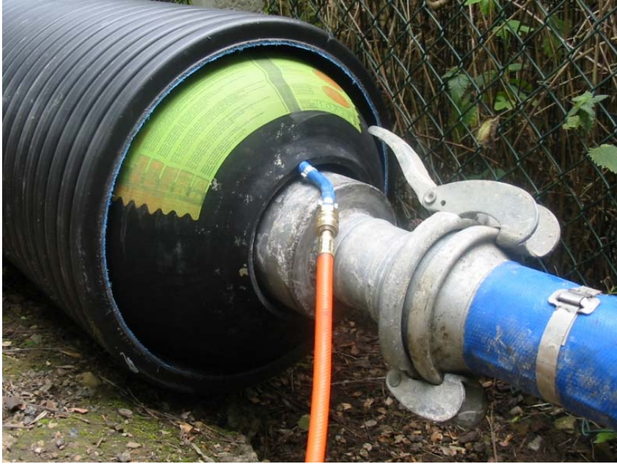
Photograph 3. Pipe Plug with Bypass
