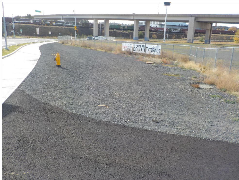
4. View of new sidewalk and east fence line, where Ben Burr Trail meets North Erie Street (looking southwest).
