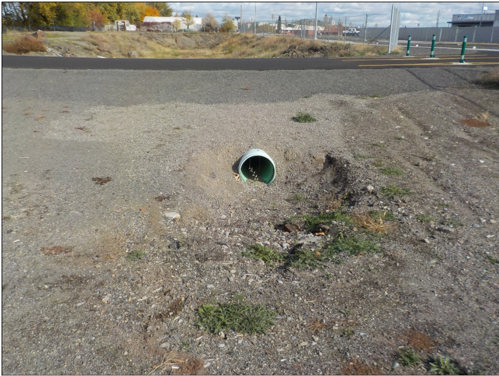
7. Culvert under new section of Ben Burr Trail, near northeast site boundary (looking northeast).
