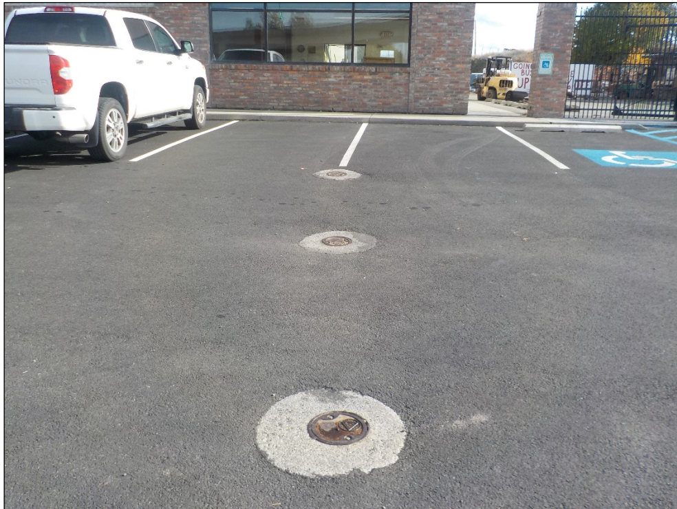
10. New asphalt pavement surrounding monitoring wells MW9-20, MW9-40, and MW9-100 (looking east).
