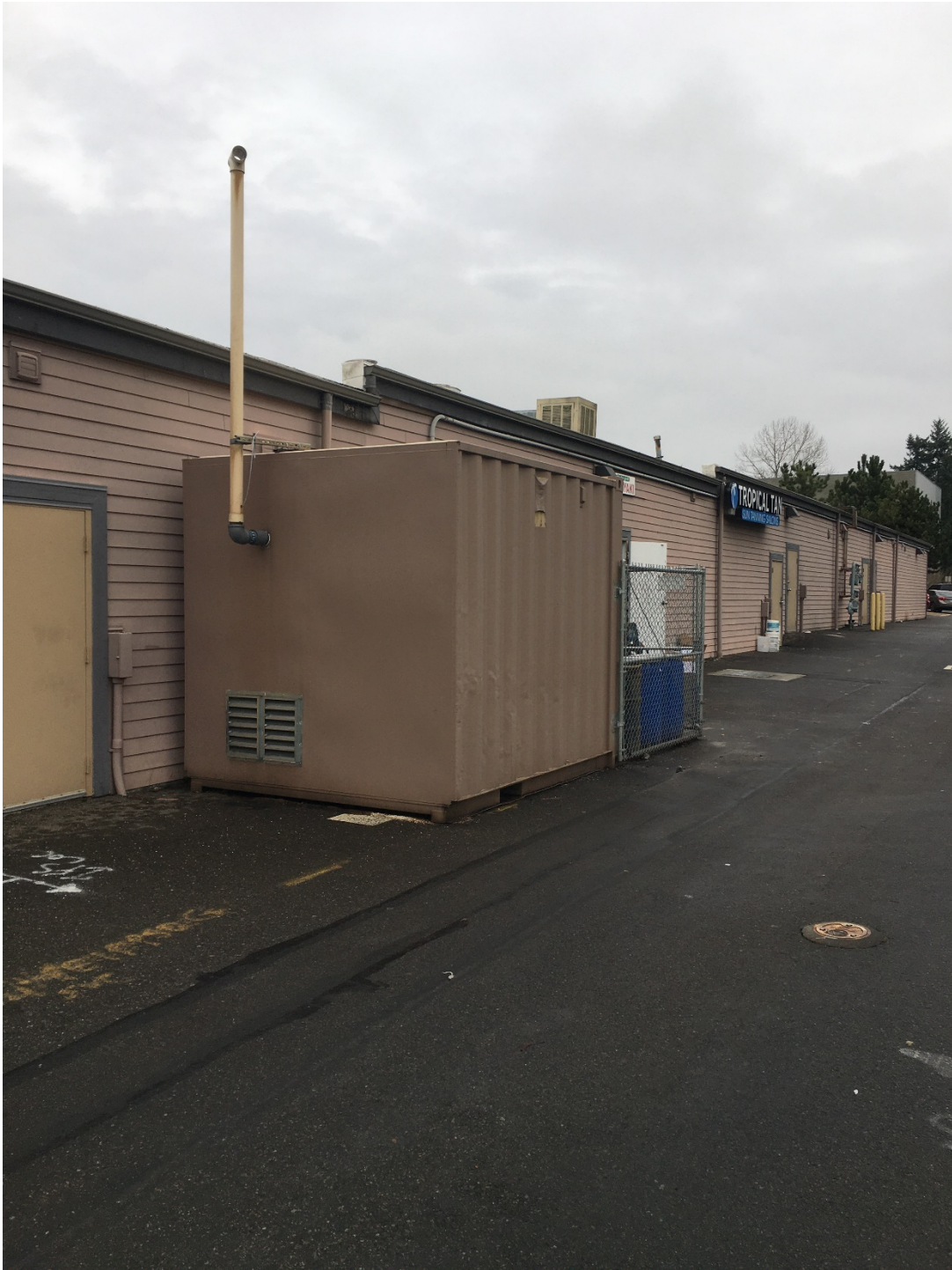
Conex box housing DPE system located on the south side of the retail building. MW-4 is visible in the bottom right portion of the photo. Photo from December 5, 2019 site visit.
