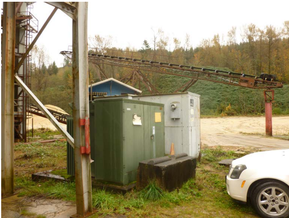
Photograph 14: Pad-mounted transformers on northeastern portion of Site, looking east.
