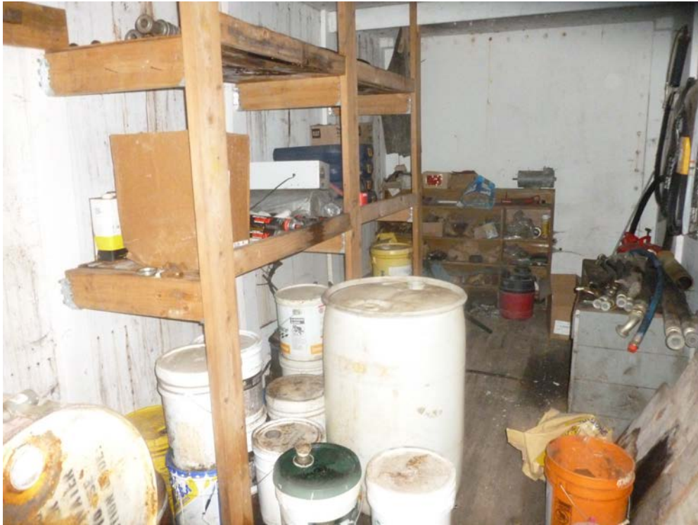
Photograph 7: Hazardous materials storage container in equipment storage area.
