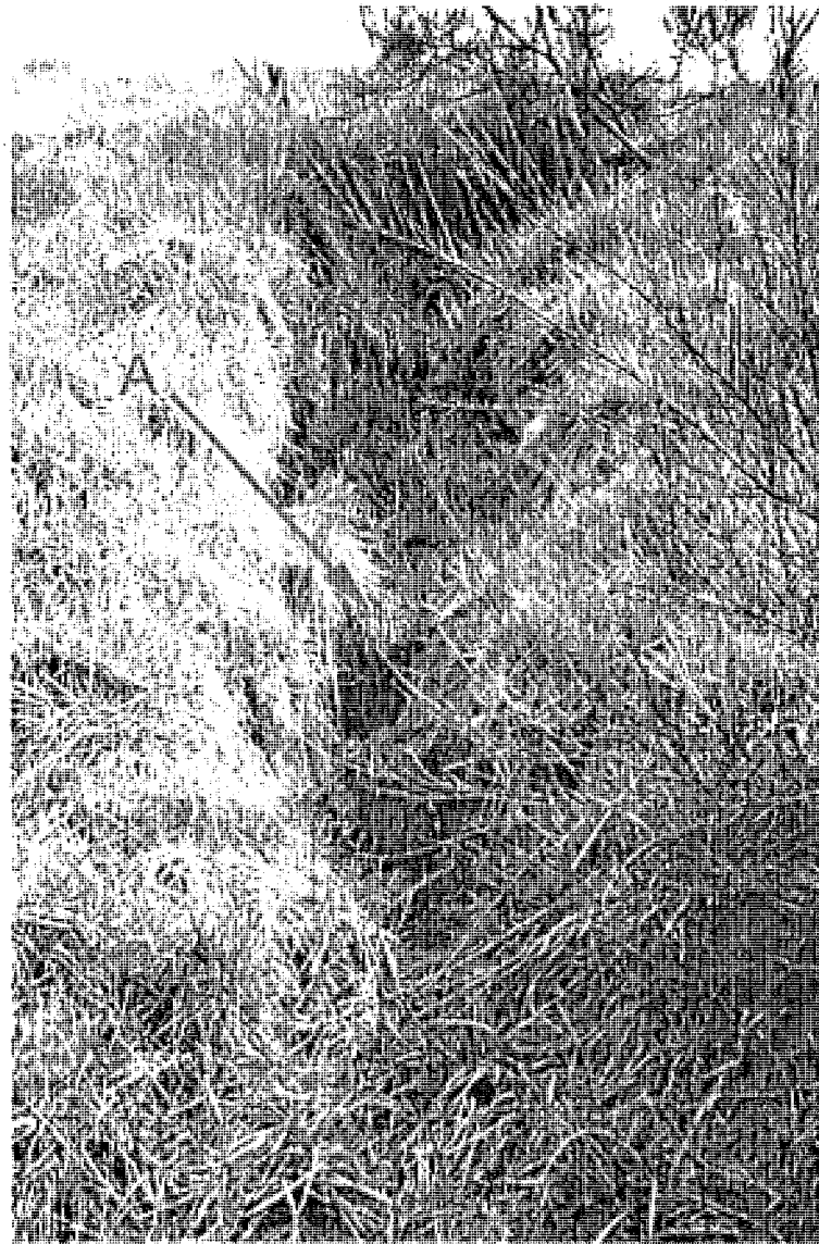
Photo 6-2 LDA. Surface erosion and cap failure ("A") on central part of the LDA.
