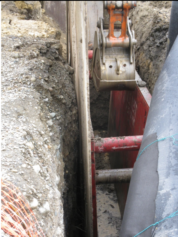
Water in bottom of trench.
