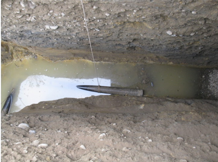
Water in trench today near piezometer B-11.
