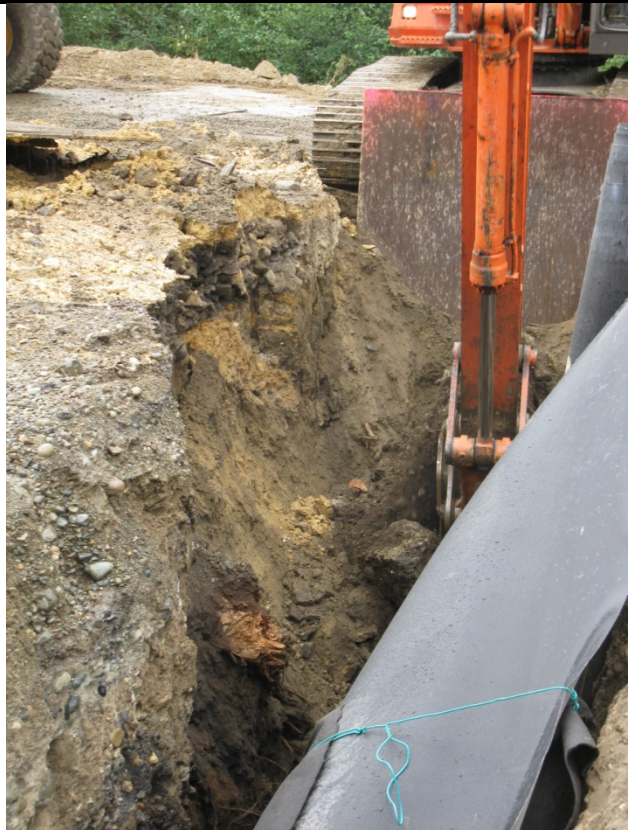
Trench caving on south wall.
