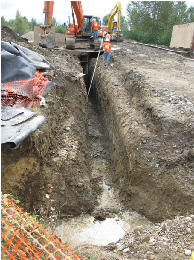
Test pit 2 drainage trench. Seep is large cobbles on trench bottom. (center)
