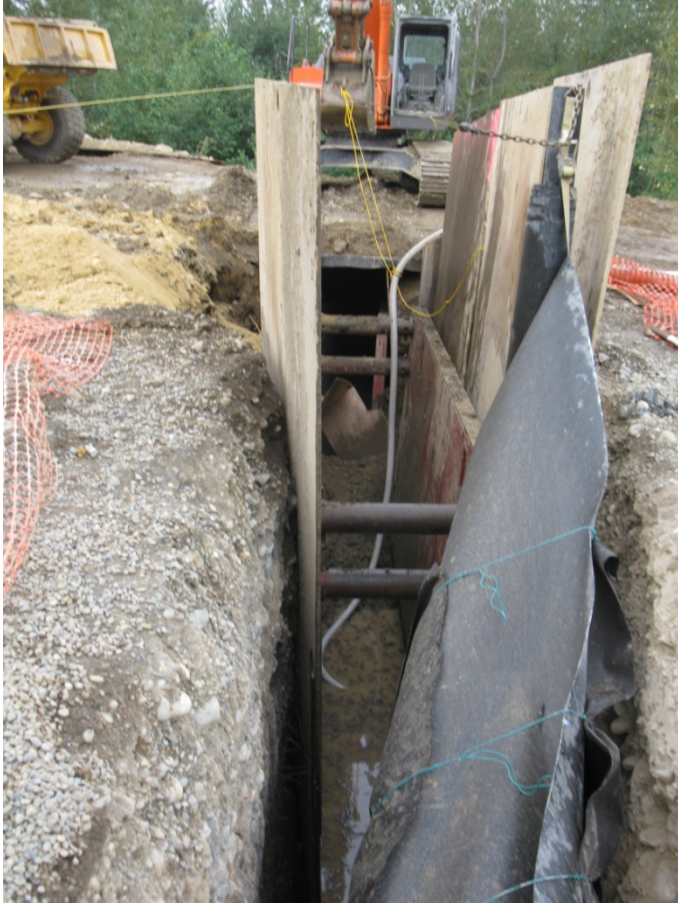
Water in bottom of trench.
