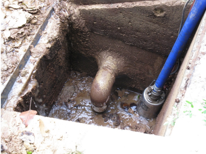
Sediment level in plugged catch basin on travertine bench.
