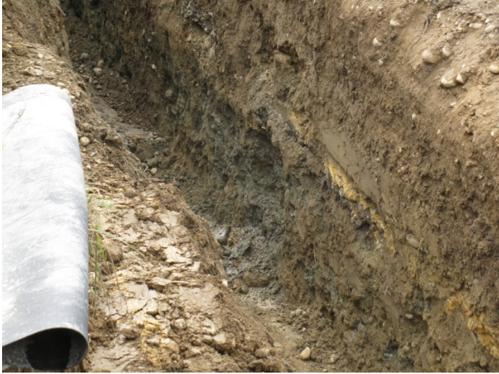
Water producing gravel seep in test pit 2 trench. (center of photo)
