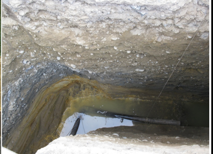
Water infiltrated into trench near piezometer B-11.
