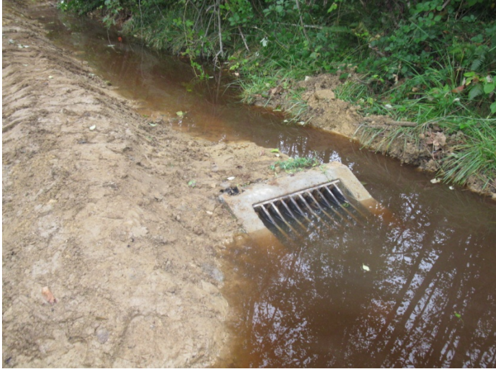
Travertine bench catch basin plugged.
