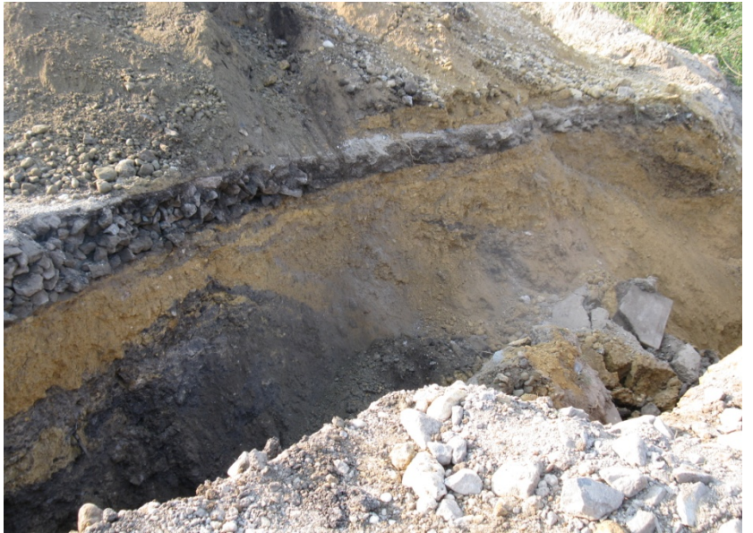
Area of trench collapse on south side of trench.
