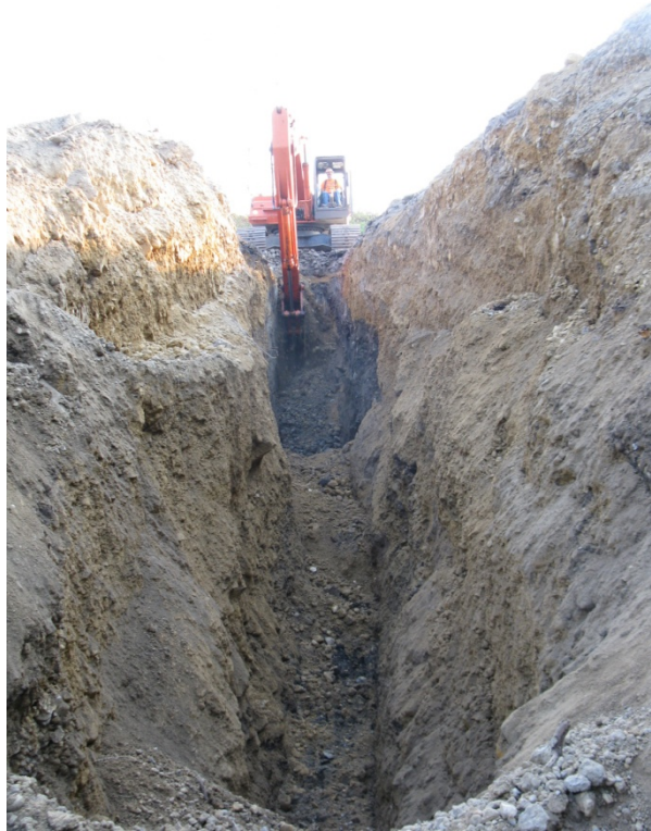
Trench looking north-east from discharge pipe outlet before collapse.
