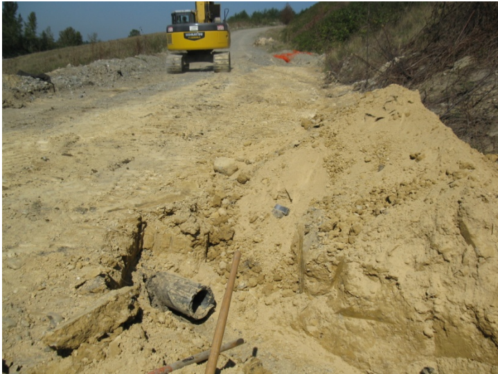
10" HDPE culvert to be repaired.
