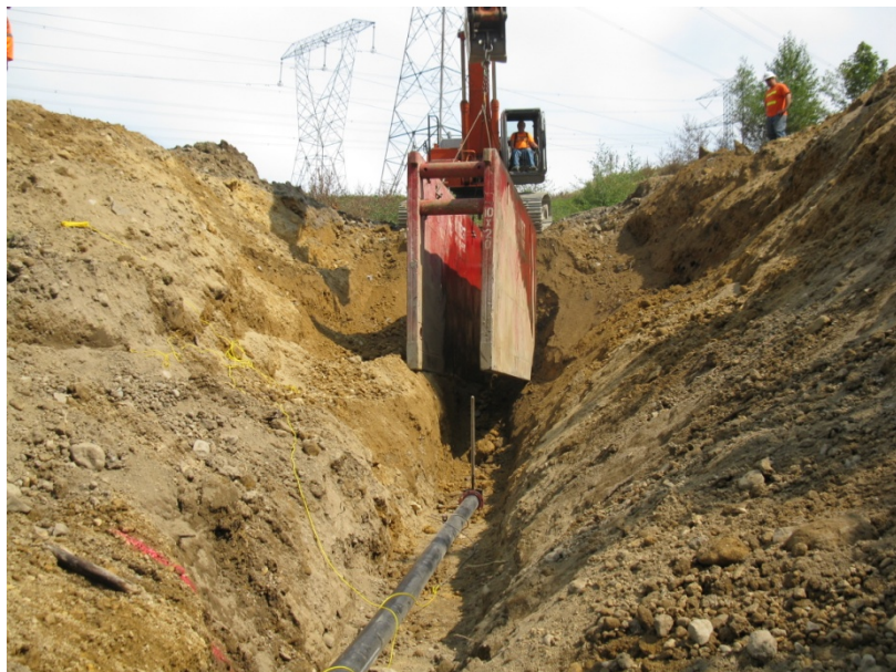
Large benched excavation looking north-east after collapse.
