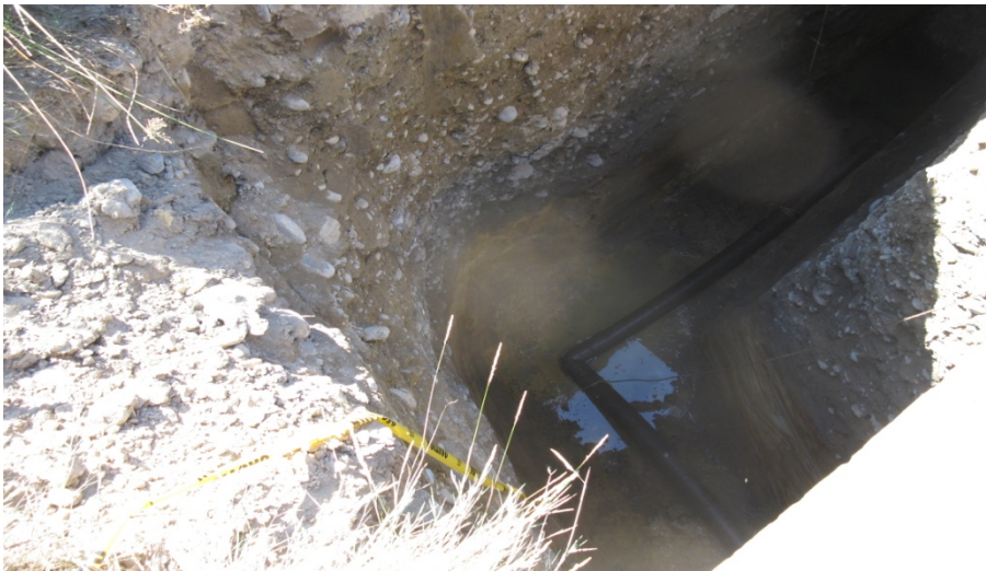
Water in trench near piezometer B-11.
