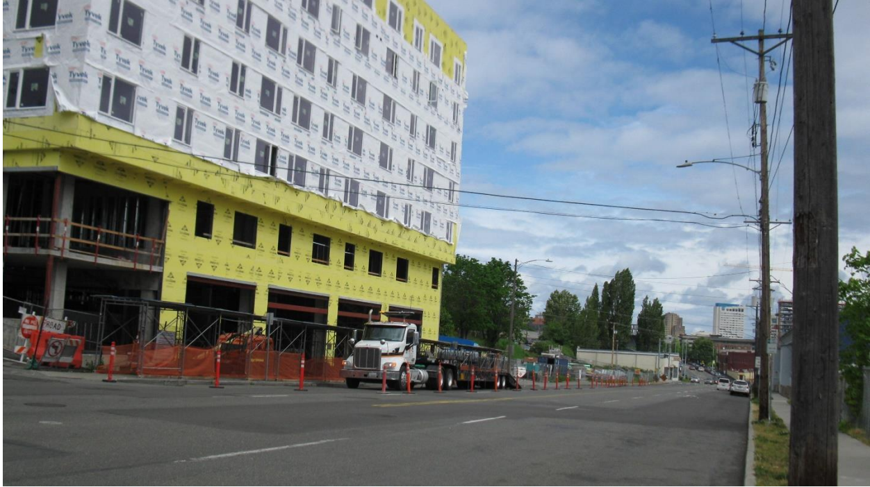
Photo 1: Residential Units Construction on Southern Portion of the Site - From the Southwest of the Site/From South 23 rd Street
