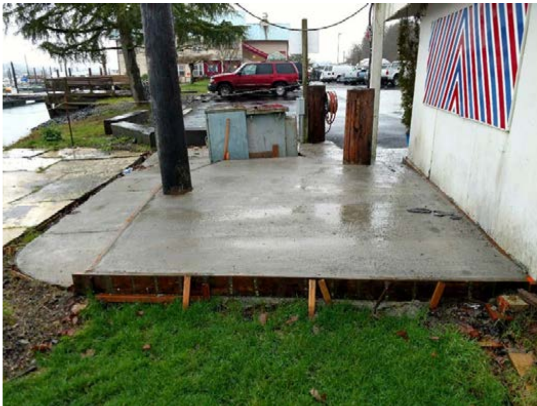
Photograph 10 – View south from the eastern portion of the excavation, showing the hydroseeded grass growing on the excavation backfill, and the newly installed concrete cap to the east of the building.
