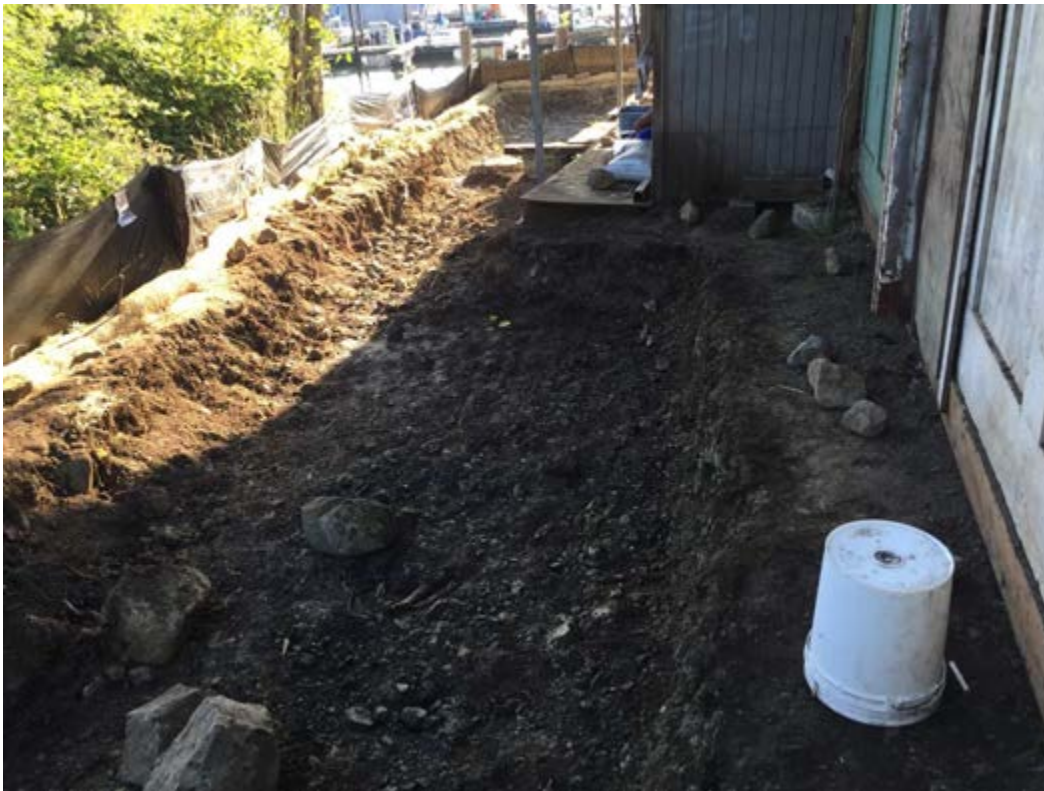
Photograph 4 – View east from the northwest corner of the office structure, showing most of the completed northern excavated area prior to backfilling.
