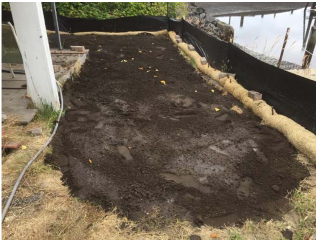
Photograph 7 – View north from the southeast extent of the excavation, showing the completed topsoil backfill and silt fencing and straw waddles remaining in place.
