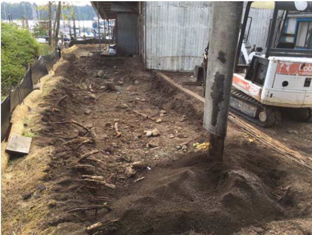
Photograph 6 – View east from the western extent of the excavation, showing the initial placement of topsoil backfill using the conveyor boom truck. The down tube was placed as low as possible to minimize dust.
