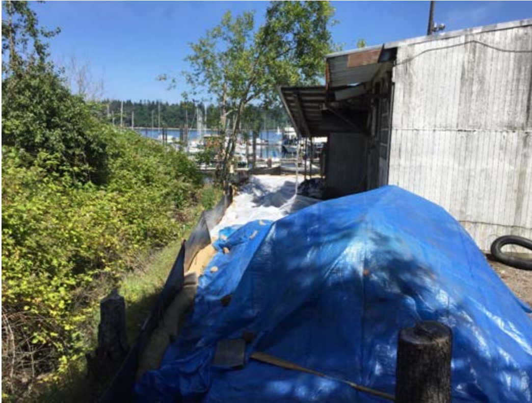
Photograph 5 – View east from the western extent of the northern excavation, showing the covered excavation area. The blue tarp covers a remaining tree stump and the white plastic covers the open excavation.
