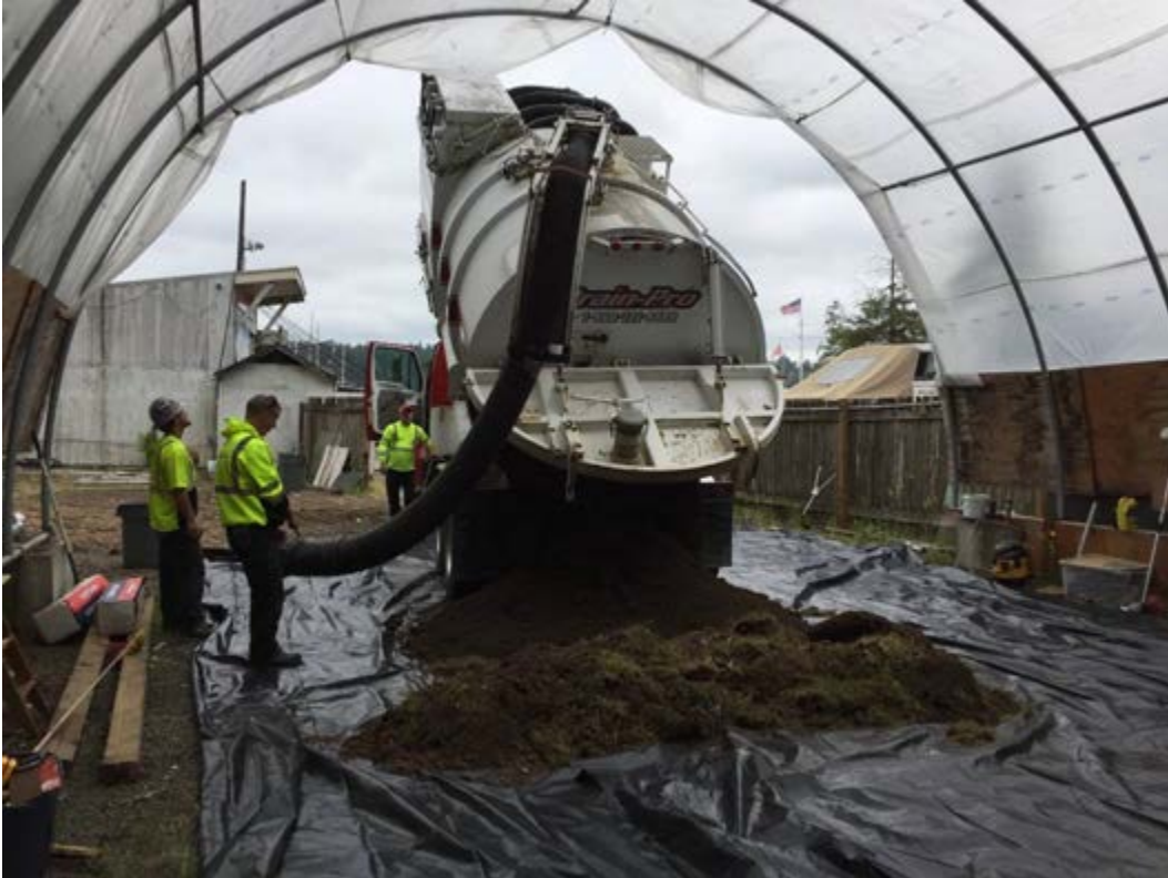
Photograph 3 – View of the covered stockpile area in the northwestern portion of the Property, showing the vacuum truck discharging its first load to the tarped stockpile area.
