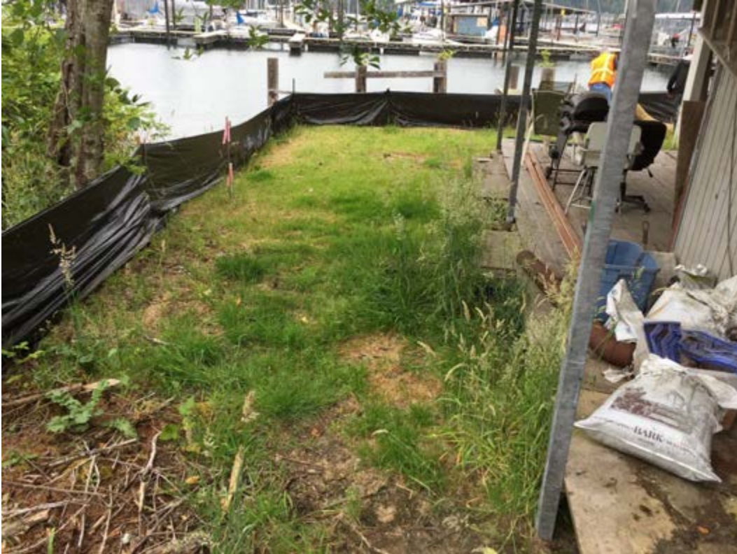
Photograph 1 – View east of the northern extent of the Property, showing installation of silt fencing along the northern and eastern excavation extents prior to placement of straw waddles.
