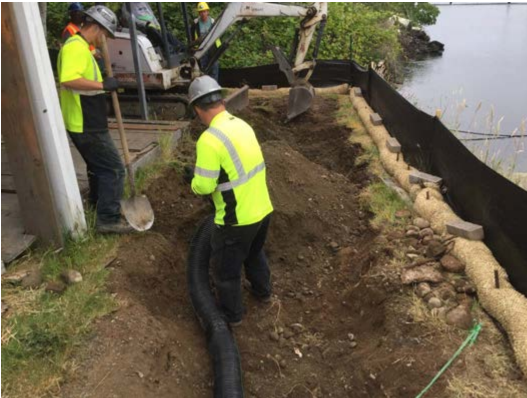
Photograph 2 – View north from the eastern extent of the Property, showing initial excavation and vacuum removal of contaminated soils, and the stormwater BMPs protecting the marine environment from impacts.
