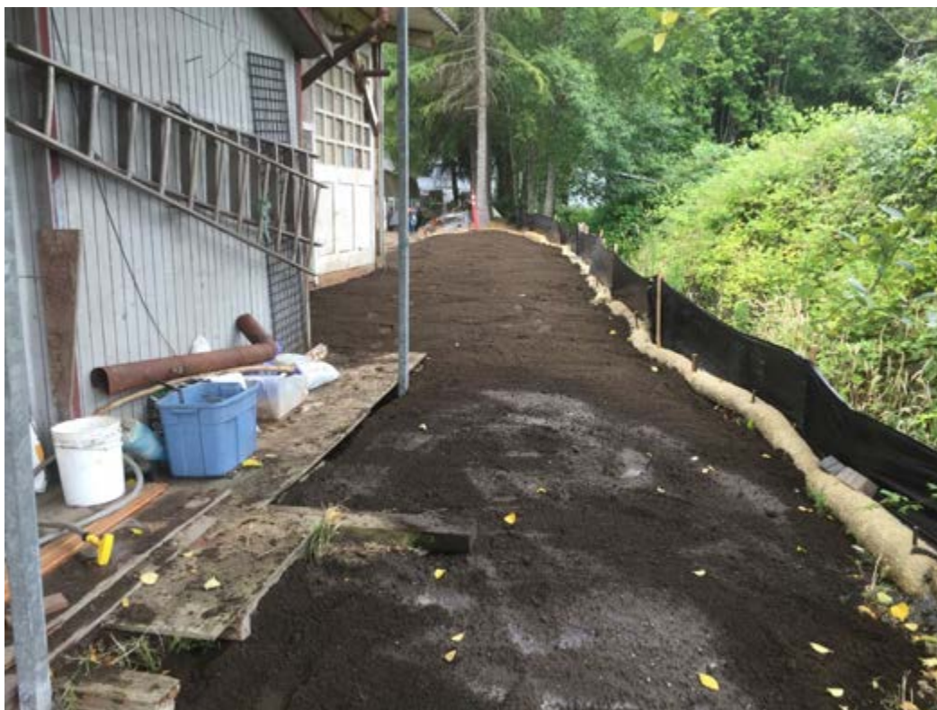
Photograph 8 – View west from the western region of the excavation, showing the completed topsoil backfill and silt fencing and straw waddles remaining in place.
