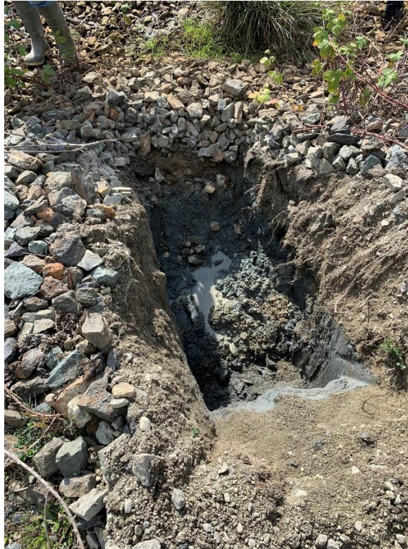
Photograph 1. TP-1 following 0- to 2-foot interval sample; the 2- to 4-foot interval flooded as soon as it was excavated. Note quarry spalls on surface.
