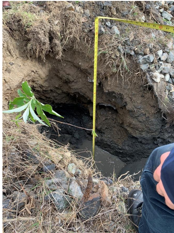
Photograph 2. TP-2 at total depth of 6 feet. Remains of broken east to west pipe visible at 3 feet bgs.
