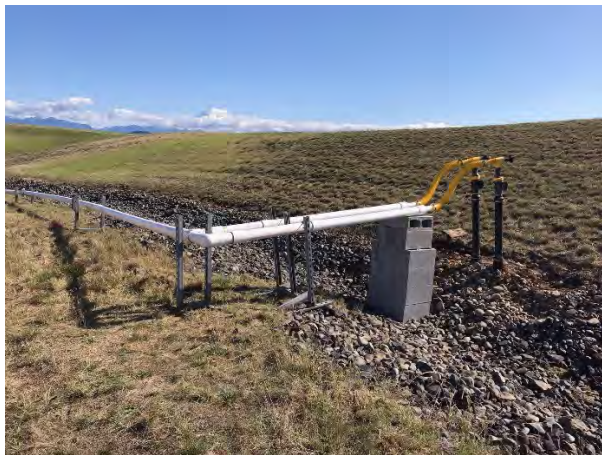
New QED wellheads at N-73 and N-75
