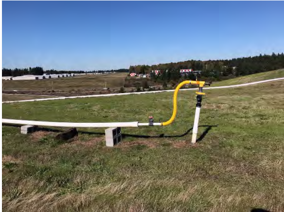
New QED wellhead at E-7
