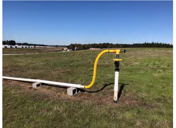
New QED wellhead at E-43
