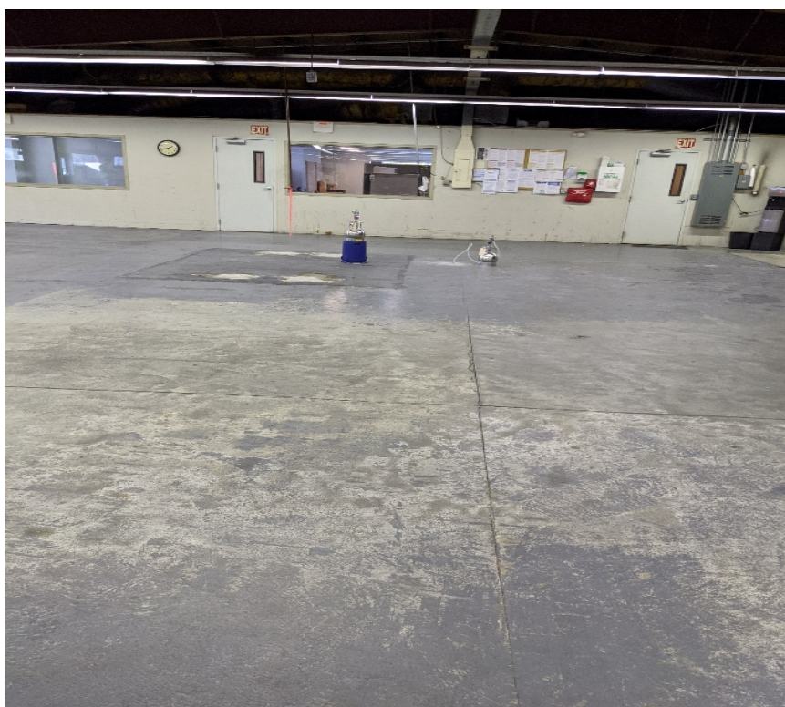
Photograph 3: Date: February 21, 2020 time: 13:39. Sample location and setup of SV-5 and IA-5 and large cracks and seams along the western half of the USM building, looking west.
