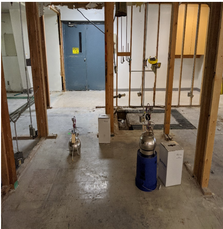
Photograph 5: Date: March 11, 2020 time: 12:52. Sample location and setup of IA-2 and SV-2 in the UMC building, looking south.
