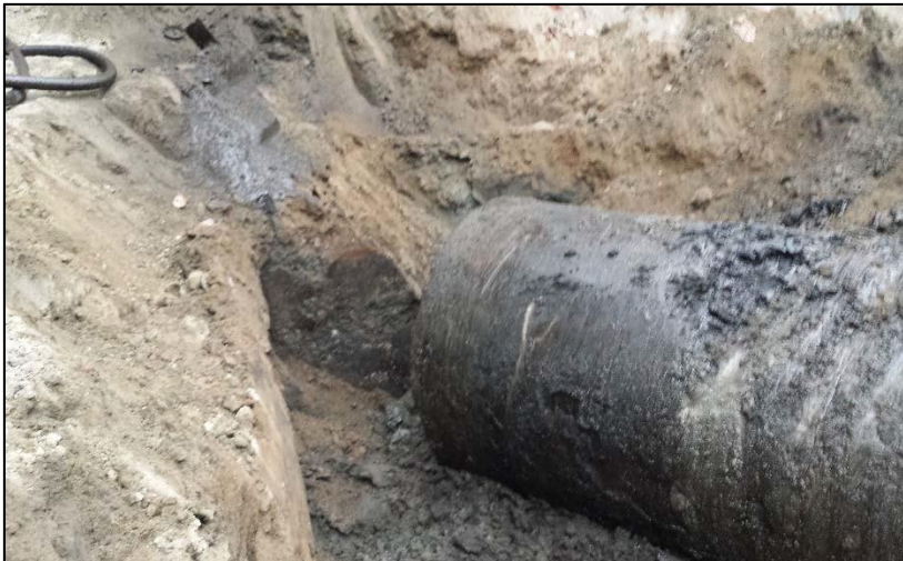
7. Controlled Density Fill inside the former UST2 and associated contaminated soil prior to excavation – Looking West
