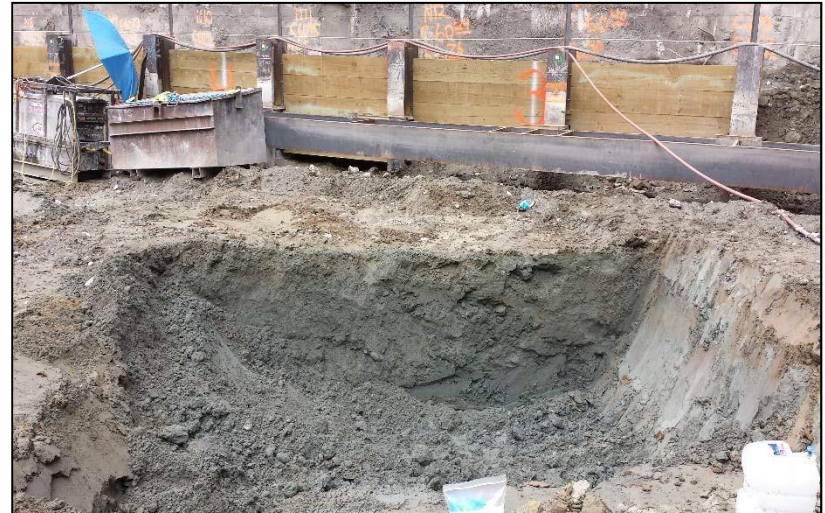
16. Clean native soil following excavation of contaminated soil at the former UST3 location – Looking North
