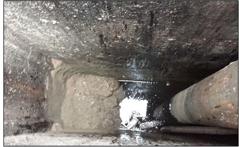
10. Concrete vault of former hydraulic hoist in central portion of subject property
