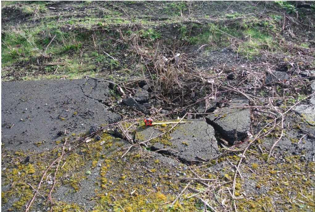
Photo 3. Damaged pavement in drainage swale (map note 5)
