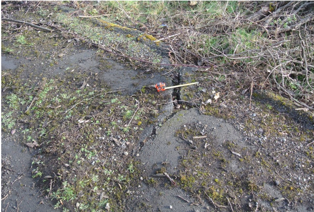
Photo 5. Damaged pavement in drainage swale (map note 7)
