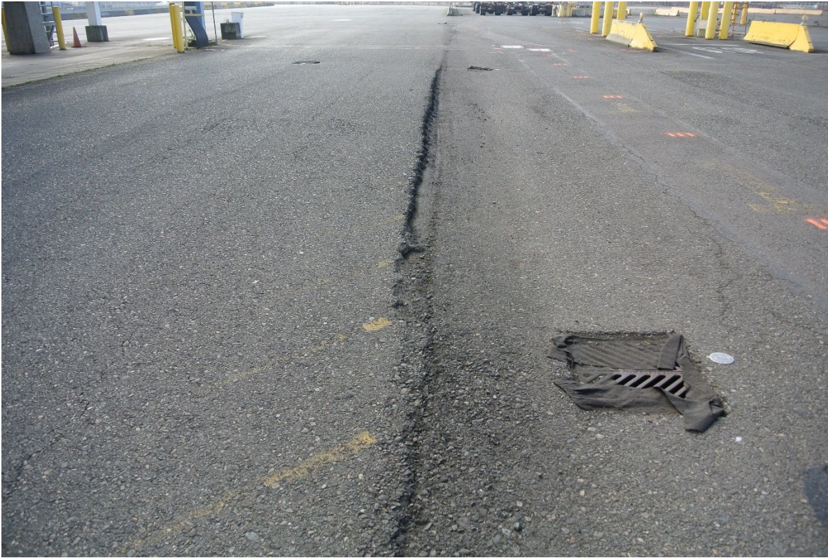
Photo 9. Pavement deterioration (map note 11)
