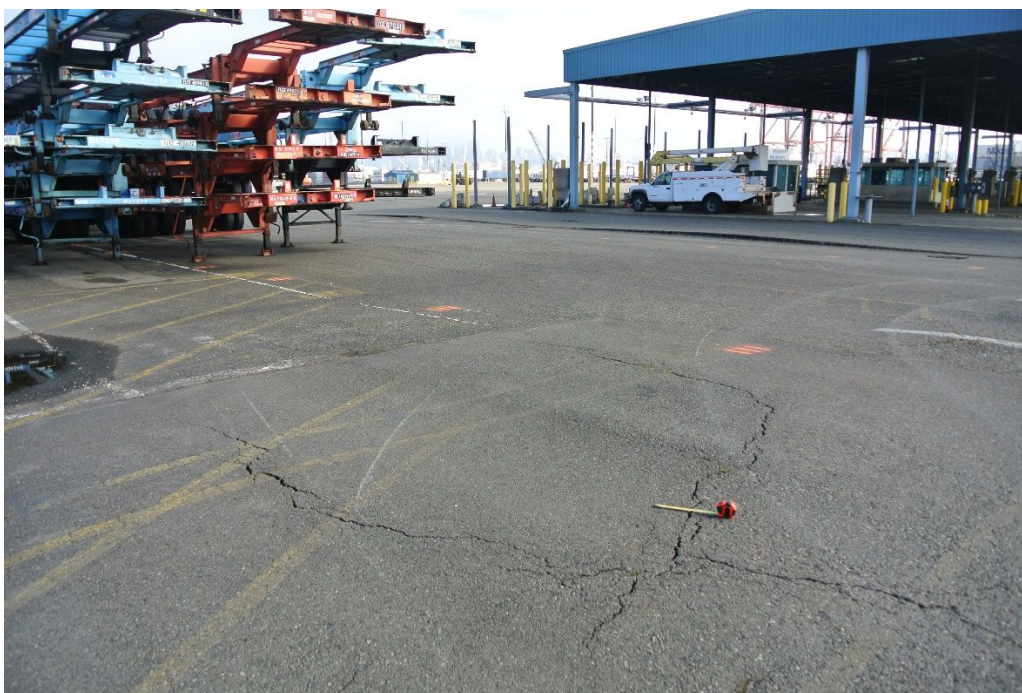
Photo 8. Pavement mounding and cracking in RA-2 (map note 10)
