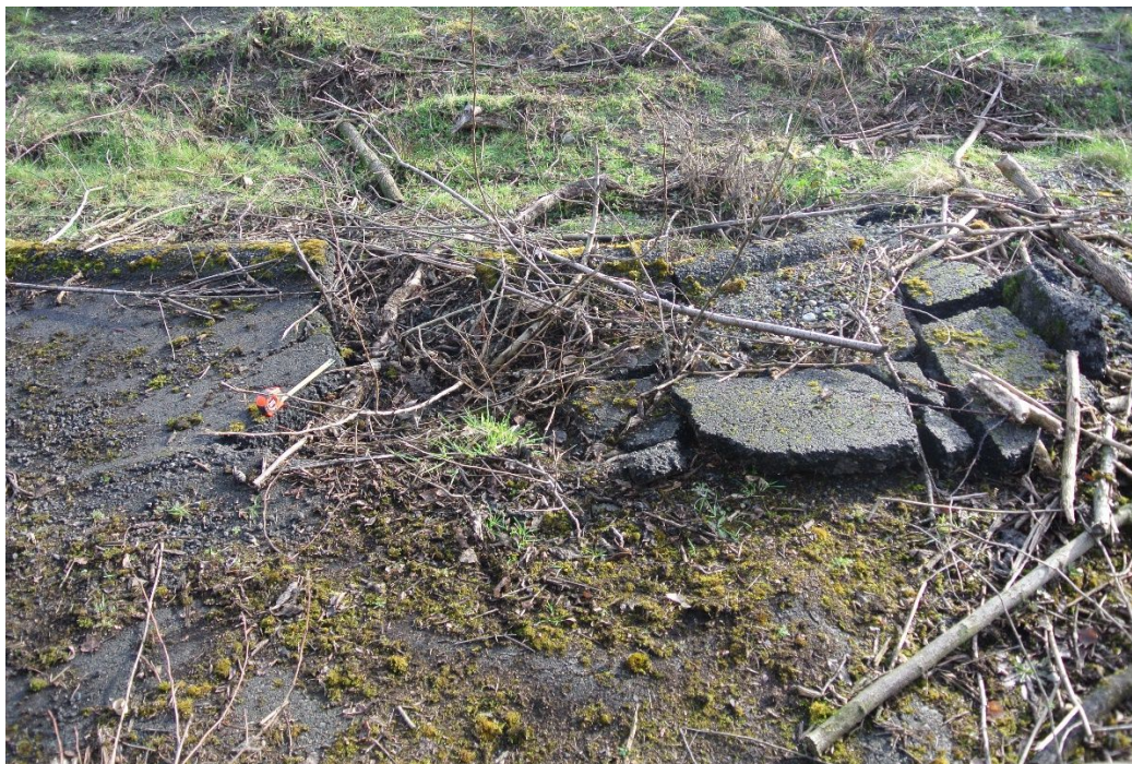
Photo 4. Damaged pavement in drainage swale (map note 6)
