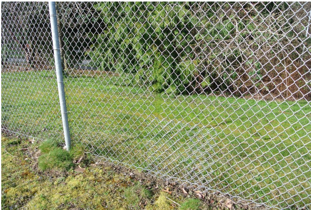
Photo 2. Hole in fence, west side of consolidated landfill: RA-3 (map note 2)
