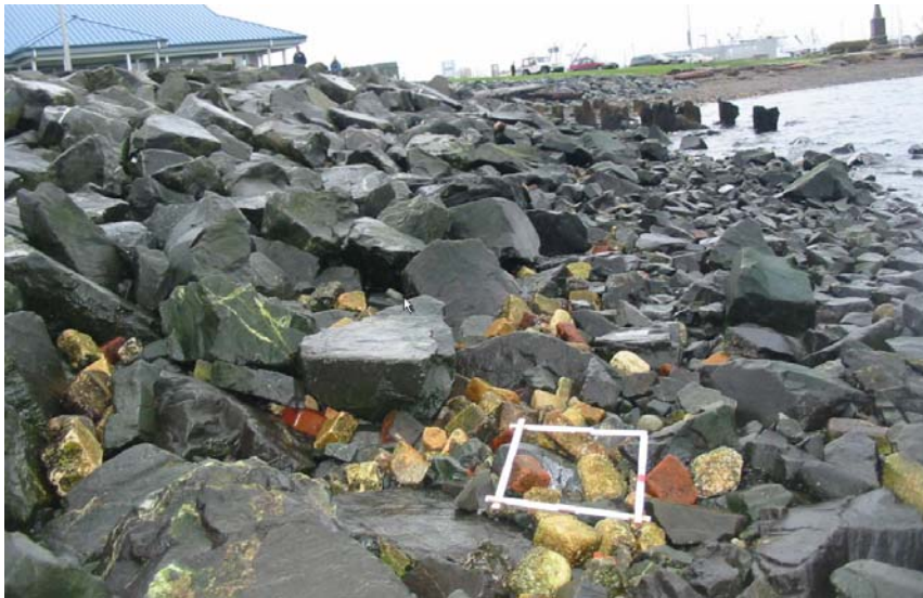
Figure 3. Revetments reduce already limited source of sediment for feeding the beach
