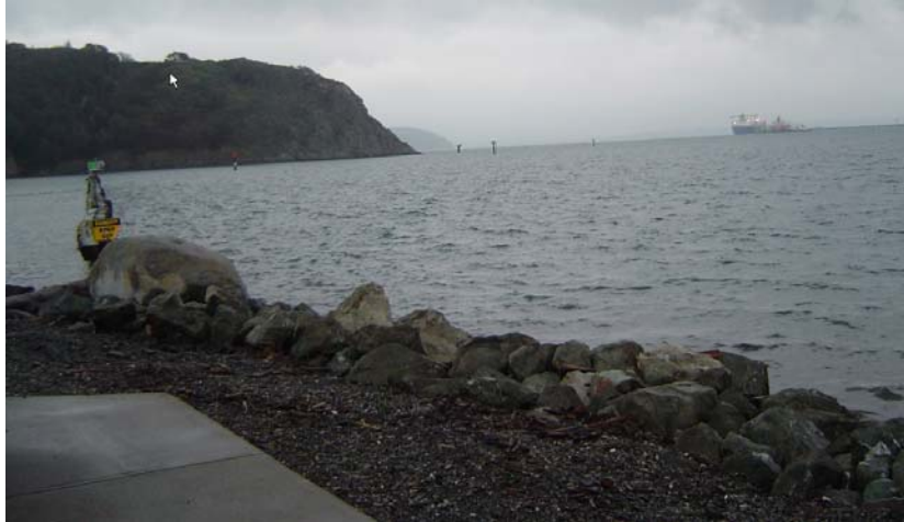
Figure 4. Rock material adjacent to timber wall breakwater that protects shoreline from incoming and reflected waves
