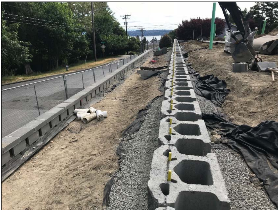
View facing east of Bristol View Apartments showing the western retaining wall along N. Bristol Street- June 5, 2018.
