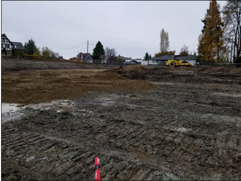
View facing east showing the 4 to 6-inches of structural fill placed following excavation of 1 to 2 feet of surficial soil within Remedial Area 2 (HCMC building) – November 8, 2017.
