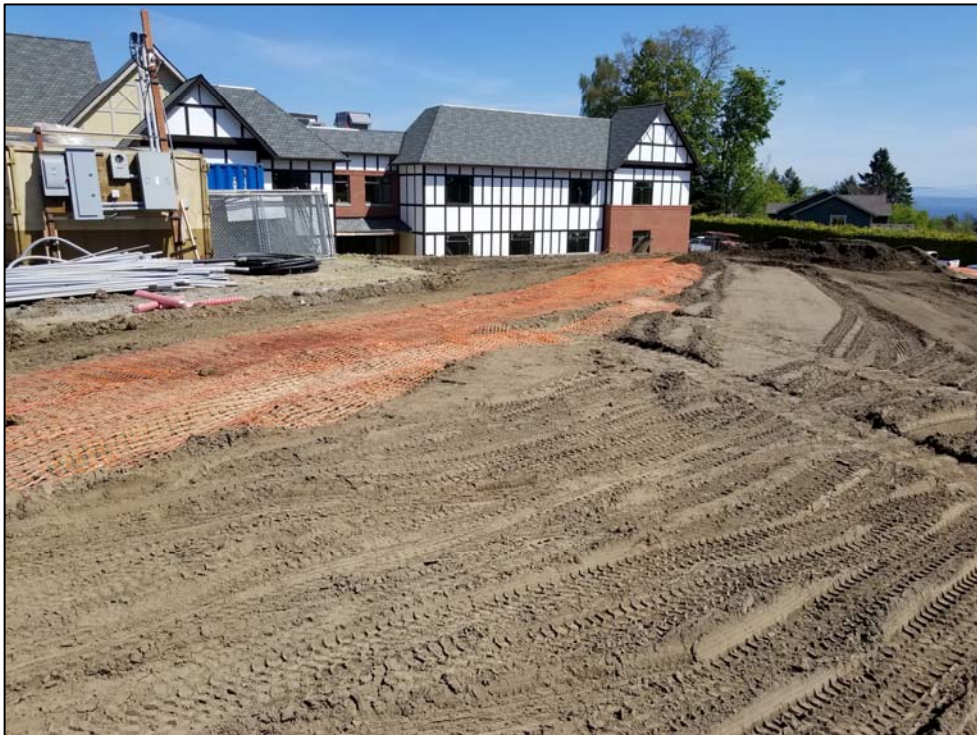
View facing northeast of modified Type 1 cap in area of HCMC-CONF-10B - May 1, 2019.
