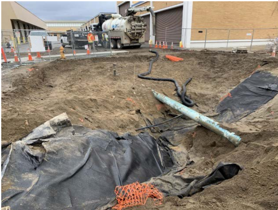
Photograph 4. Exposed section of damaged liner, looking North.
