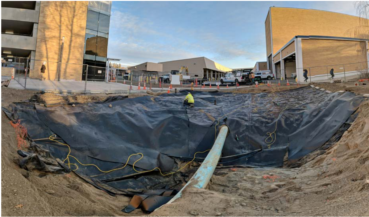
Photograph 9. ACF West places 40-mil thick LLDPE geosynthetic liner over bedding sand within the liner repair area, looking North.
