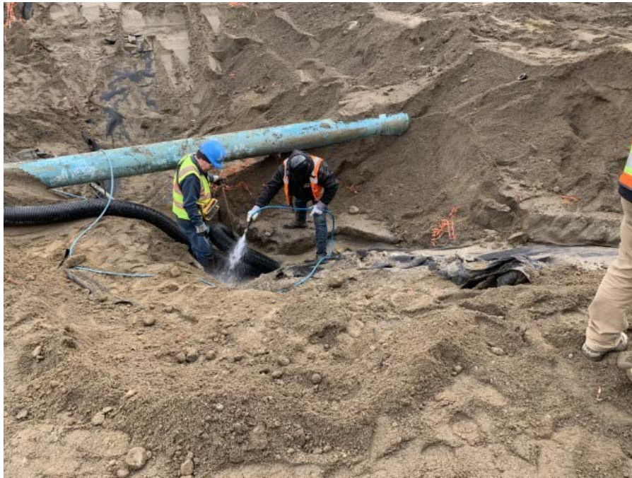
Photograph 2. SES exposes damaged liner using pressurized water and a Hydroexcavator vacuum truck, looking West.
