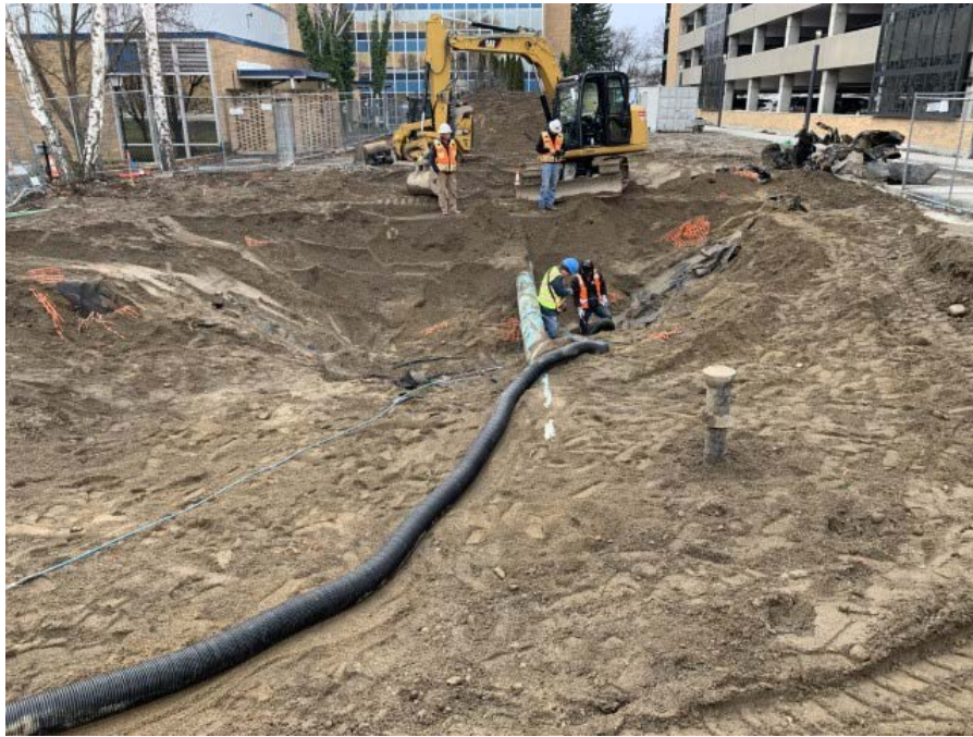
Photograph 1. SES over excavates to expose damaged liner at the north end of the site, looking South.
