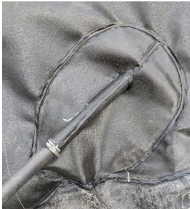
Photograph 12. Welded liner boot around the east side of the protruding water line, looking East.
