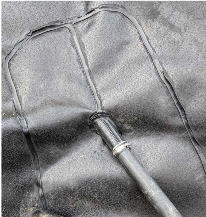
Photograph 13. Welded liner boot around the west side of the protruding water line, looking West.
