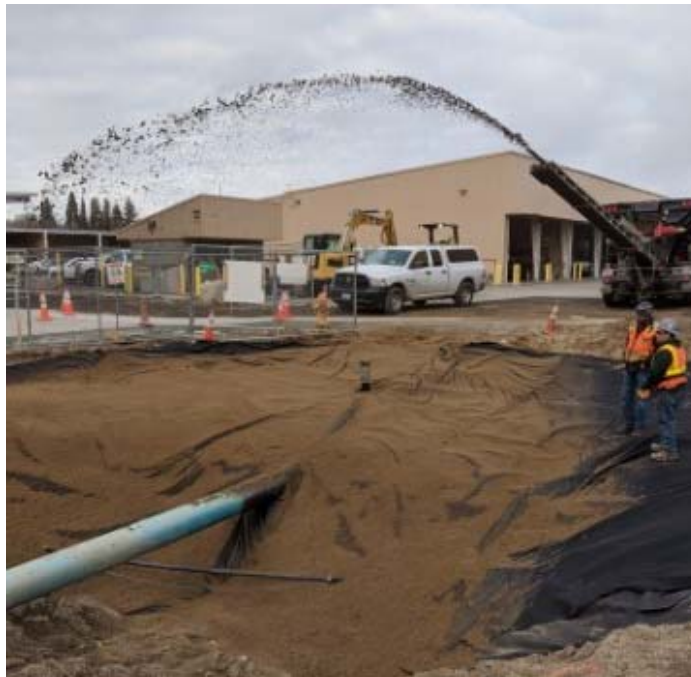
Photograph 18. SES places approximately 4-inches of bedding sand over geotextile fabric using a dump-truck conveyor belt system, looking Northwest.
