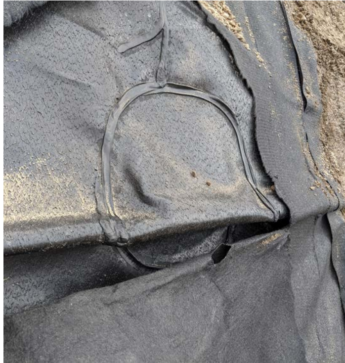
Photograph 15. Welded liner patch near the eastern edge on the existing liner, looking East.
