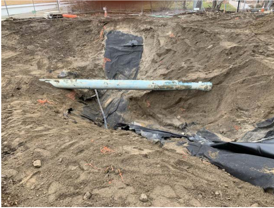
Photograph 5. Exposed section of damaged liner, looking East.
