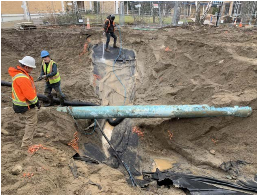
Photograph 3. SES exposes section of damaged liner, looking West.
