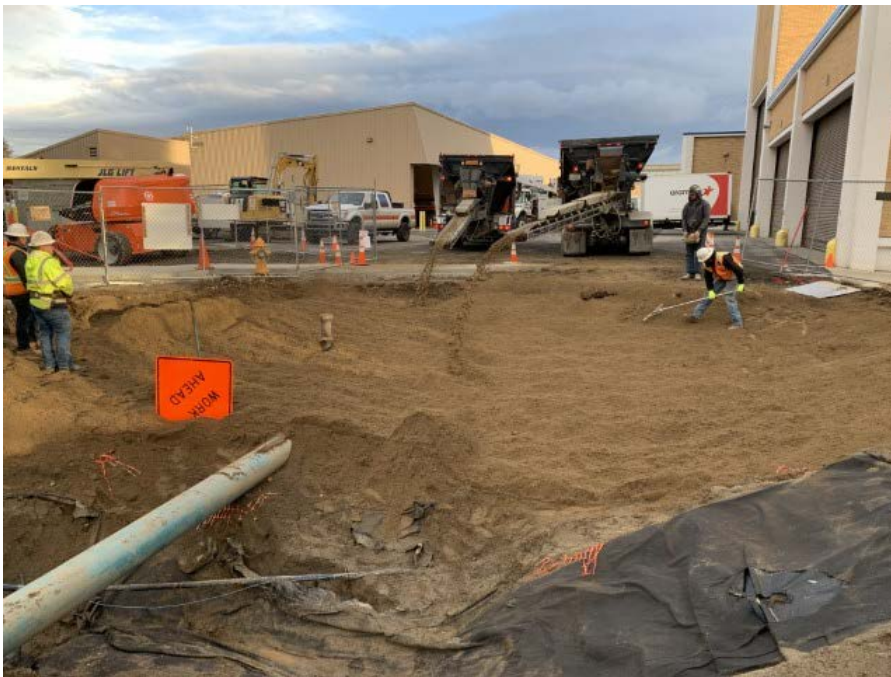
Photograph 6. SES places bedding sand for geosynthetic liner repair using two dump truck conveyor belt systems, looking North.
