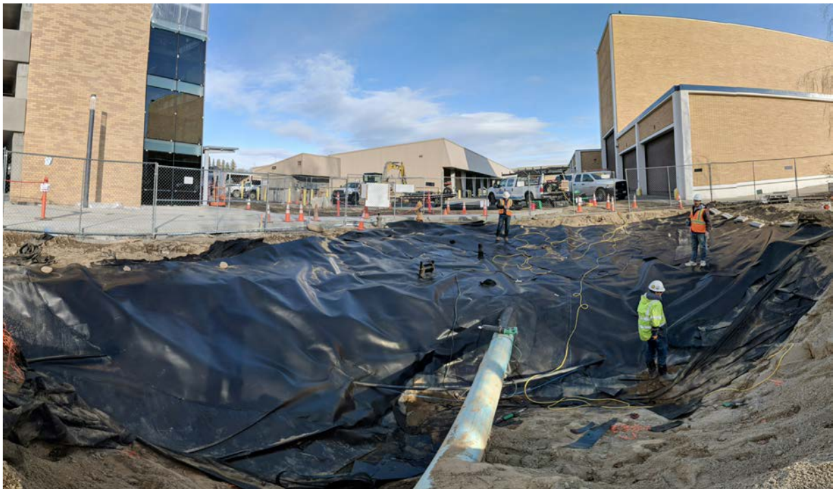
Photograph 16. ACF West finishes welding replacement liner section to existing liner, looking Northwest.
