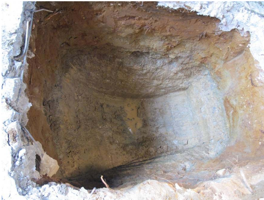
13. North hydraulic hoist soil excavation, measuring approximately 6 feet wide by 8 feet long and 9 feet deep
