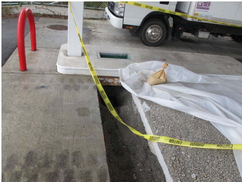
12. Fuel dispenser island piping excavation showing saw cut concrete and fuel dispenser sump
