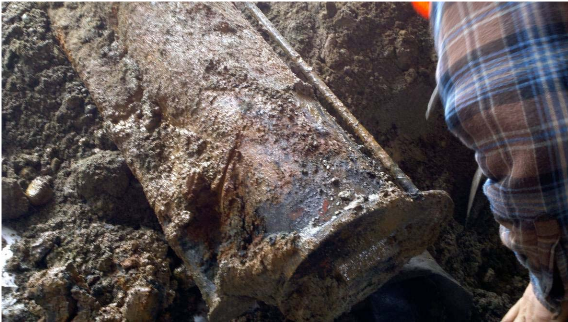
3. North hydraulic cylinder during removal showing corrosion at base of cylinder
