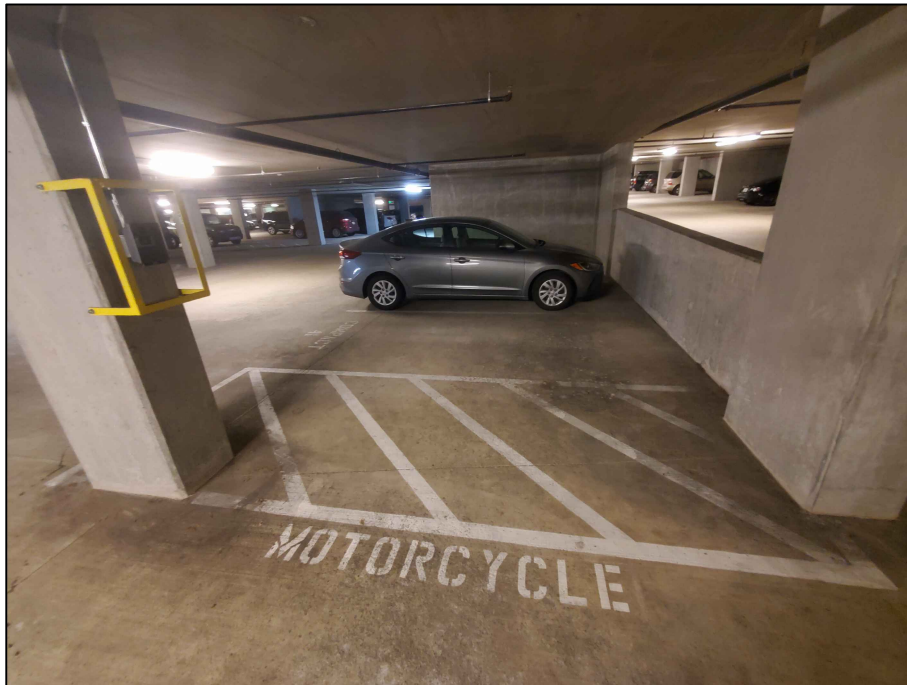
Photograph 3: View looking east representing the condition of the garage floor slab in Area 2.
