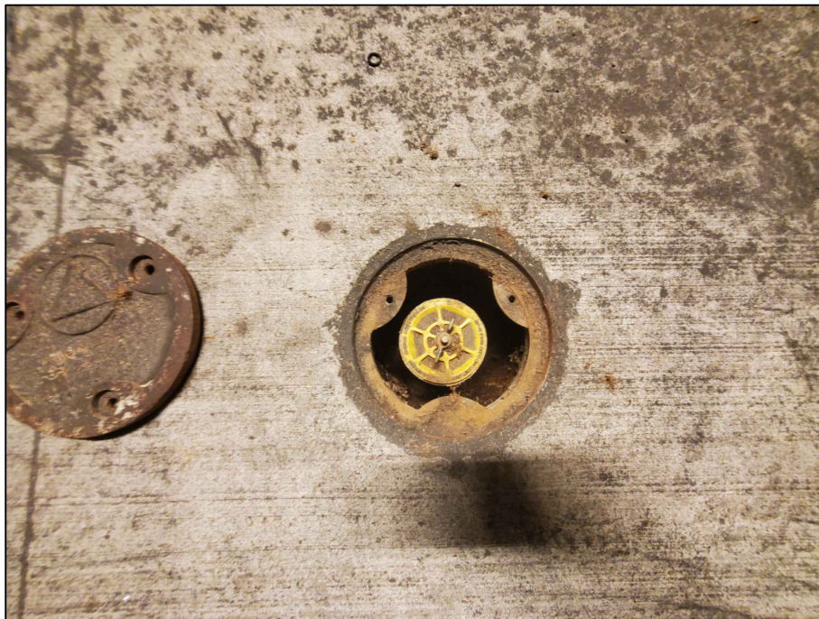
Photograph 6: View of well RW1 without the well cover.
