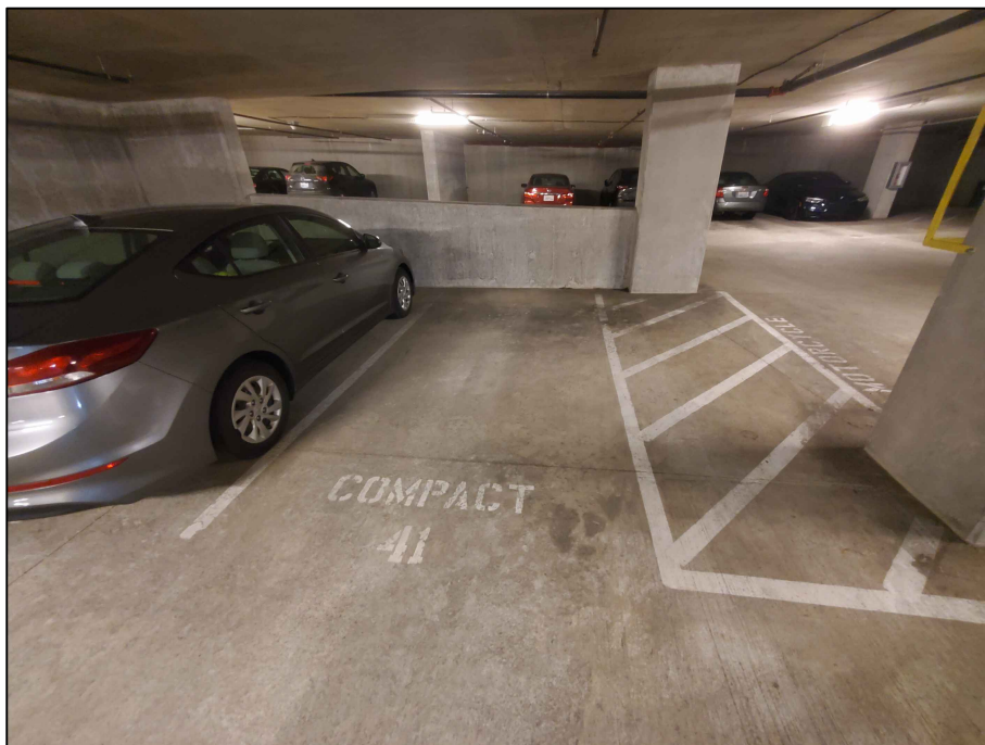
Photograph 4: View looking south representing the condition of the garage floor slab in Area 2.
