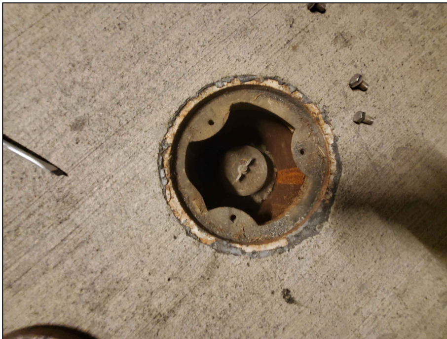
Photograph 8: View of well RW2 without the well cover.
