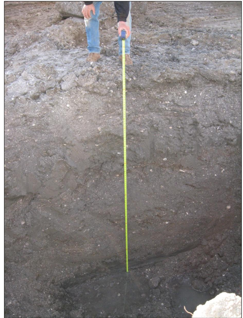
4. Soil conditions after excavation of concrete vault structure; no sheen observed on soil or exposed groundwater
