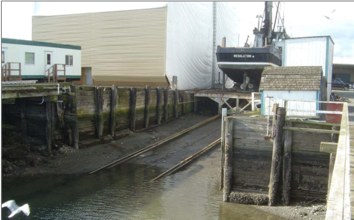
2. General layout and conditions; orientation is to the northwest. Marine railway extending upland with a boat shown on the cradle; timber bulkhead around upland perimeter; metal building with white tarp provides covered area for boatyard activities.
