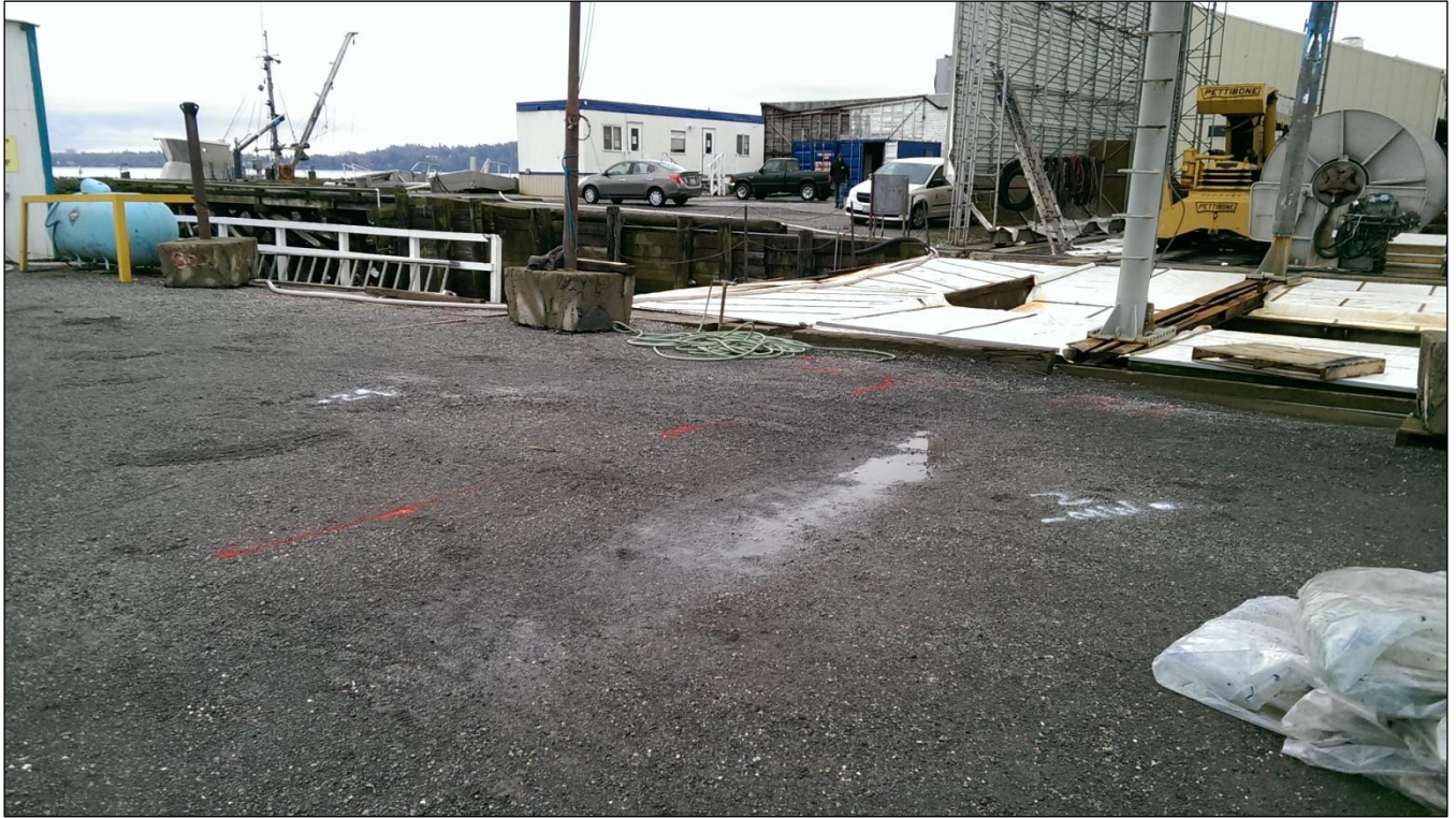
1. General layout and conditions; orientation is to the southwest. Gravel working surface in foreground; boat cradle on the right.
