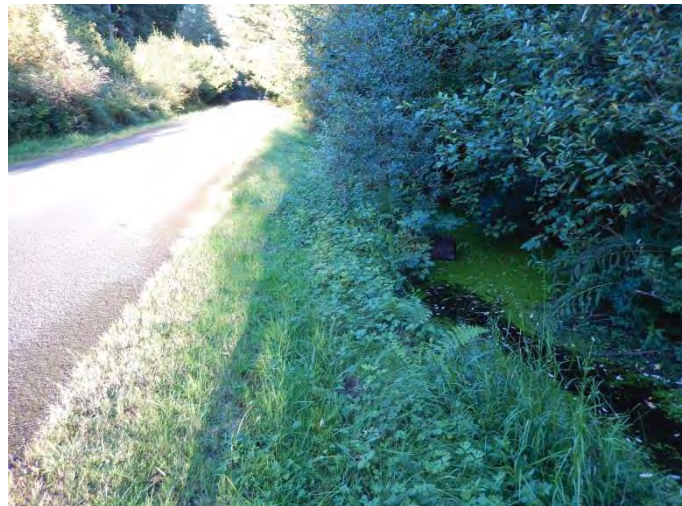
Photo 28: 28 th Avenue NW north of Subject Property Water in ditch and slowly flowing through culvert.
