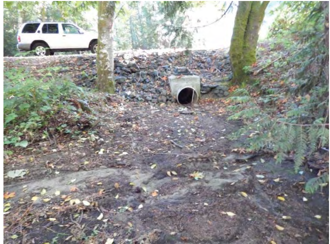
Photo 20: Dry ditch at 14 th Ave E of Cooper Point RD
