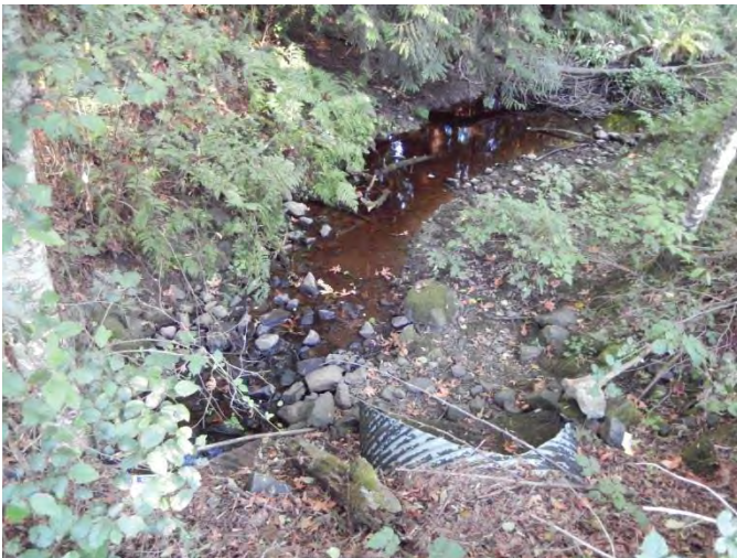
Photo 27: Kaiser Road North of Subject Property Flowing water & associated wetlands
