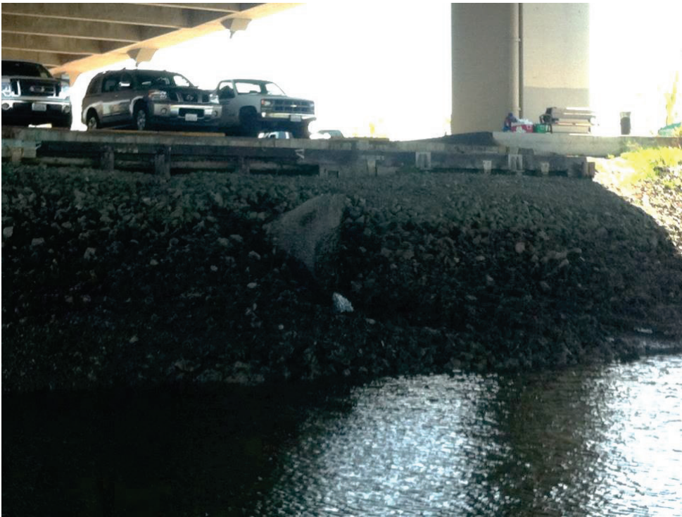
Figure 25 – Looking at Outfall 243 on the East Bank Slope under the SR-509 Bridge
