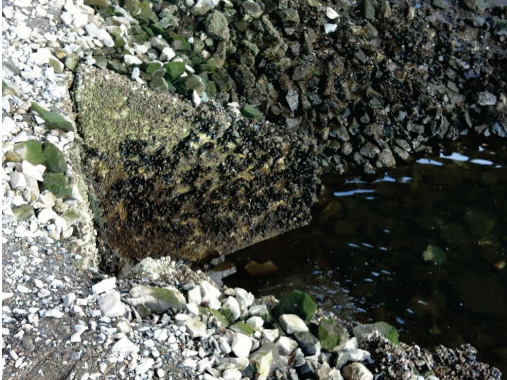
Figure 3 – Outfall #235 South Wingwall Separation
