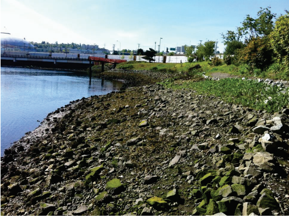
Figure 11 – Looking Southeast at Derelict Pier and West Bank Slope of the Waterway
