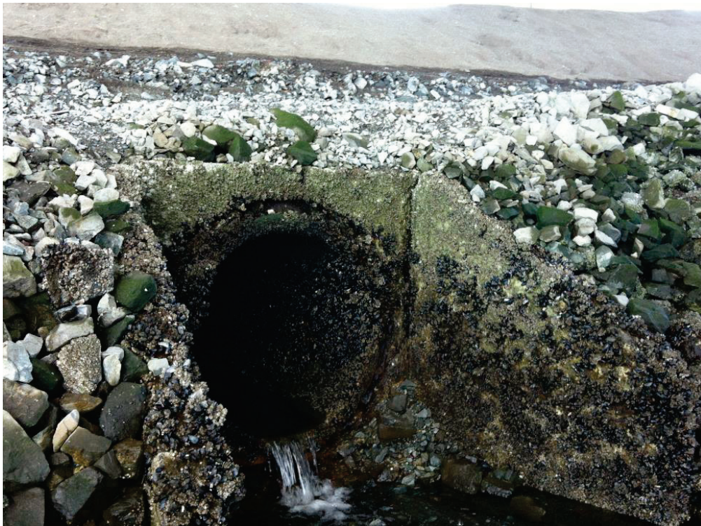
Figure 4 – Outfall #235 Wingwalls Separation
