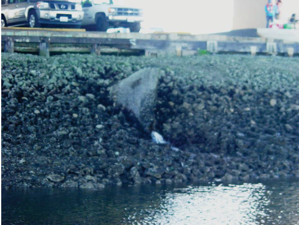
Figure 26 – Outfall 243 on East Bank Slope of the Waterway Covered with Barnacles
