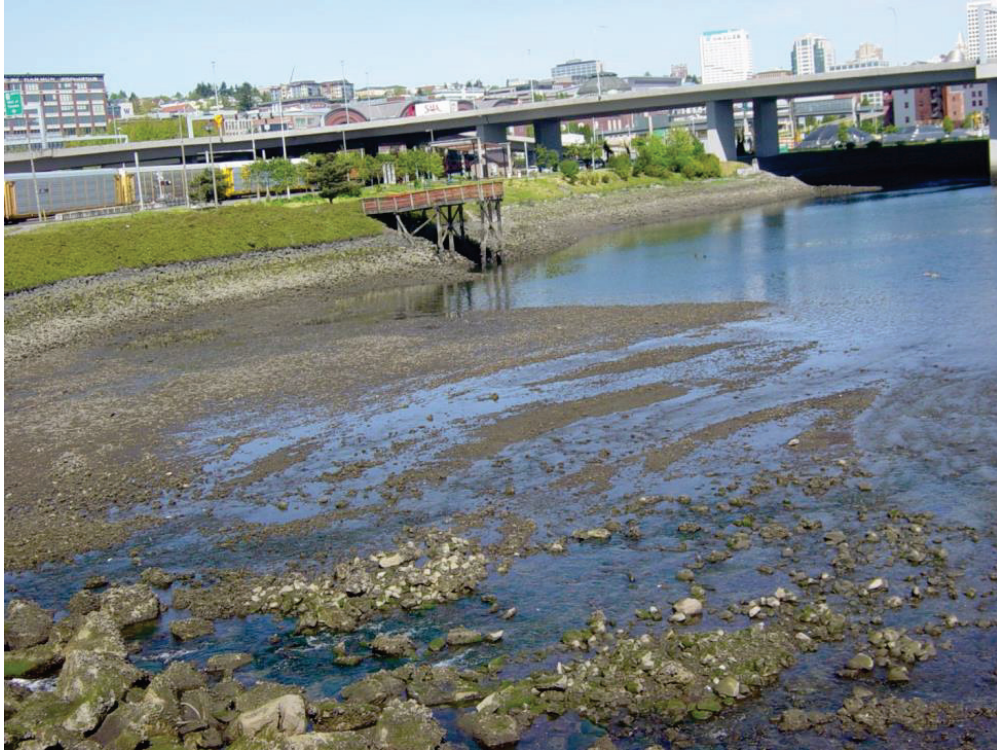
Figure 20 – Looking West across the Scour Apron at the Head of the Waterway
