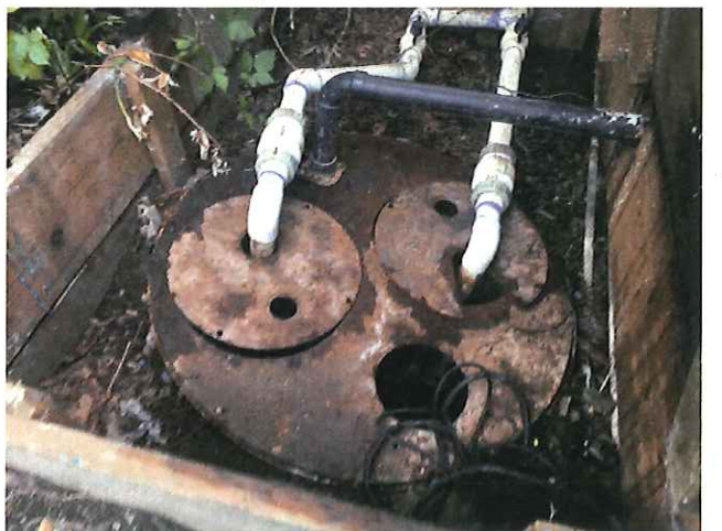
Photograph 6. Sewage pump located northwest of the building.
