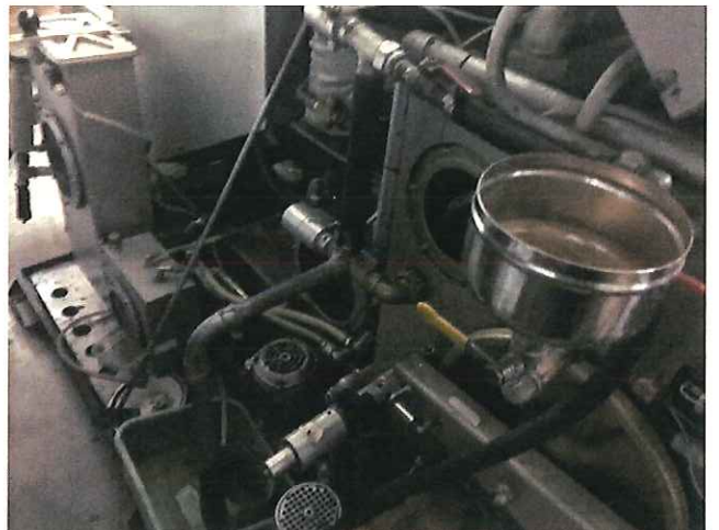
Photograph 4. Dry cleaning machine showing metal plate beneath for secondary containment.
