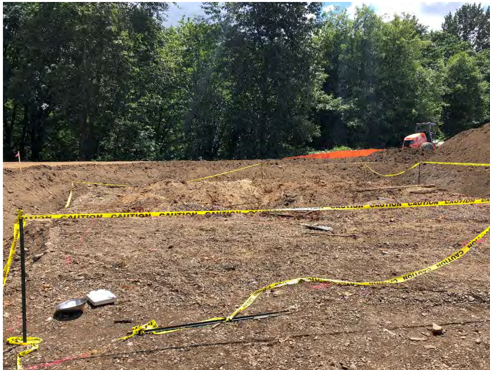
5. Looking south at AOC3 before excavation and with temporary construction road in the background.
