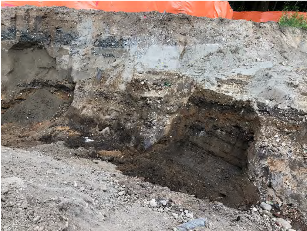
7. South sidewall of AOC1, with AOC1-SW17 on left and AOC1-SW-18 on right.
