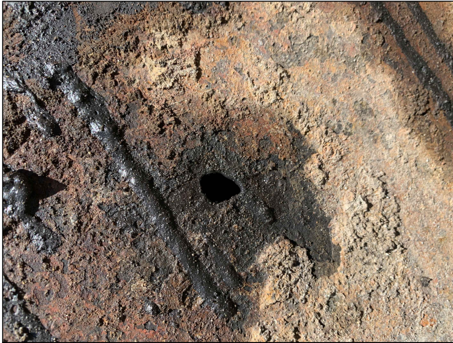
Photograph 3: View of the approximately 0.5-inch hole located on the top east side of USTA.
