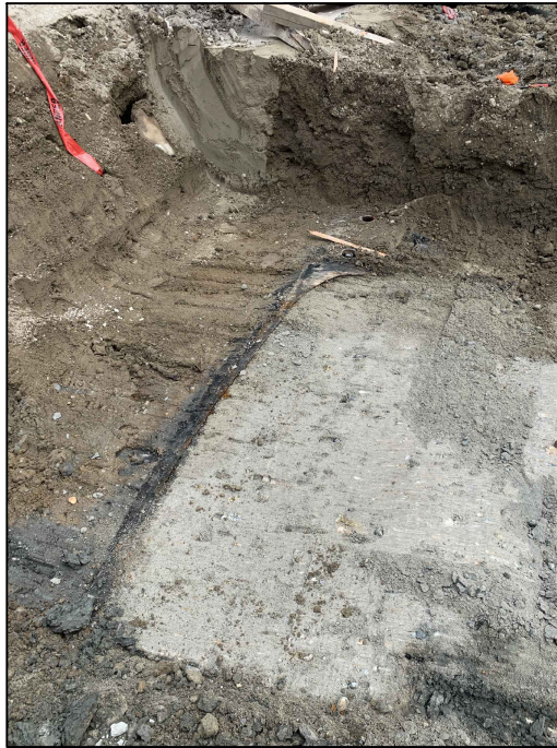
Photograph 5: View of a large hole on the top of UST6B where the UST was likely cut prior to filling the UST with CDF.
