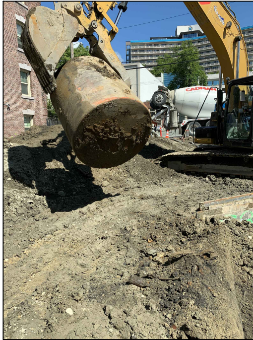
Photograph 1: View of the removal of 1,066-gallon diesel UST4A situated on the west-central portion of the Property. No evidence of holes or a release were encountered.
