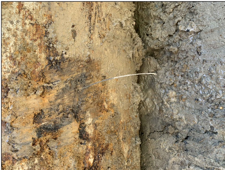
Photograph 4: View of the approximately 3 millimeter hole located on the bottom east side of USTA.
