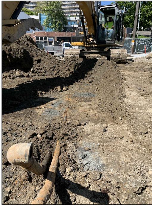
Photograph 11: View of suspected product pipe situated on the southwest portion of the Property, which may have been associated with former UST4.
