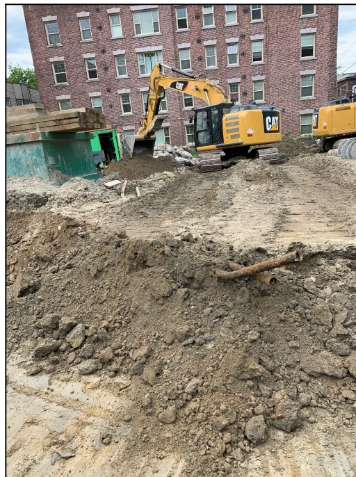
Photograph 8: View of suspected product piping encountered on the east-central portion of the Property near former boring DP3. It was not confirmed which UST this pipe belonged to.
