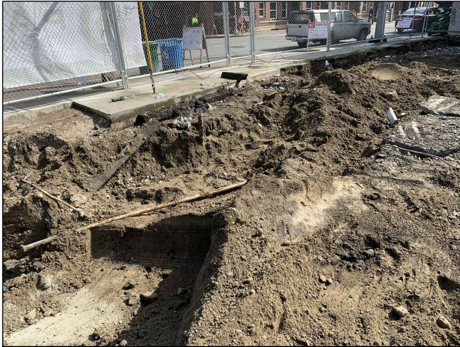
Photograph 9: View of a former pump island and associated product pipe situated on the east-central portion of the Property, which may have been associated with UST6B.
