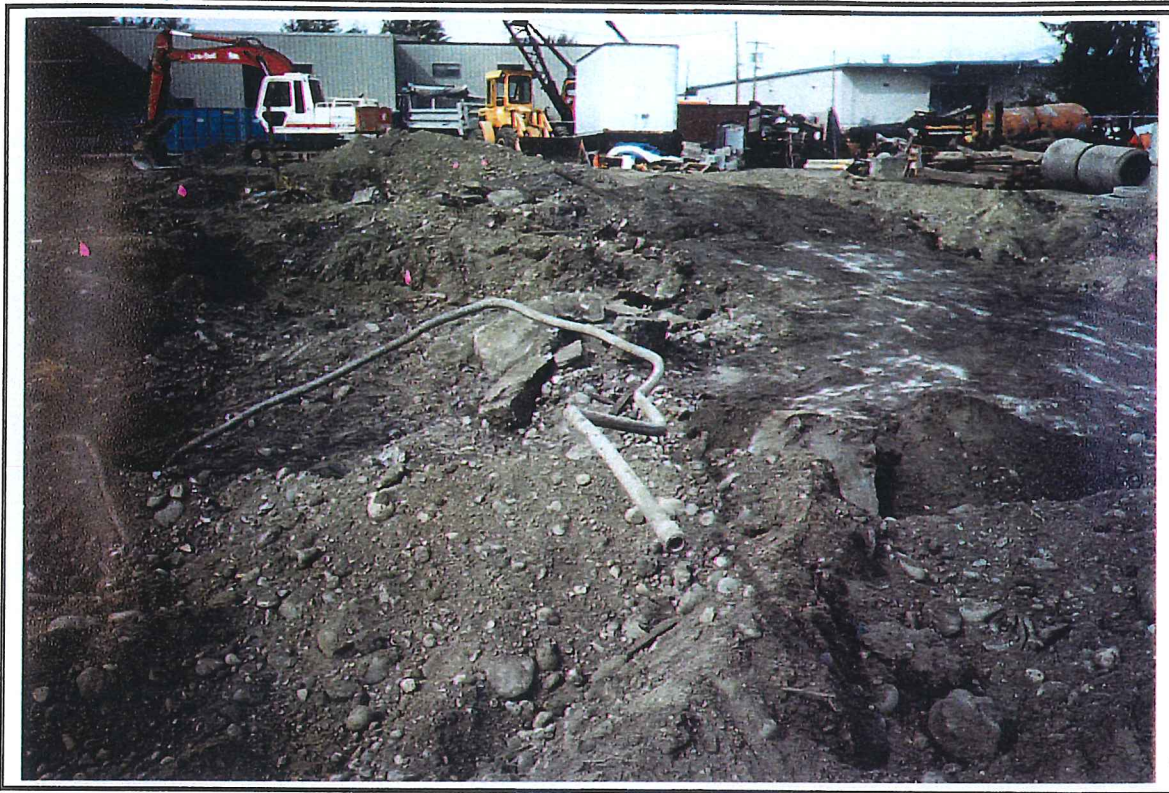
Photo #21: Metal steam lines unearthed adjacent to the removed fuel storage tank on the Westwater Construction site, facing north. The old foundation of the demolished home is depicted on the right side of the photograph. Approximately 1-1/2 feet of fill material contaminated with heavy oil and lead was scraped from off of the slab and disposed of. Diesel fuel contaminated soil was remediated left of the slab. Photo taken on 8/31/01.
