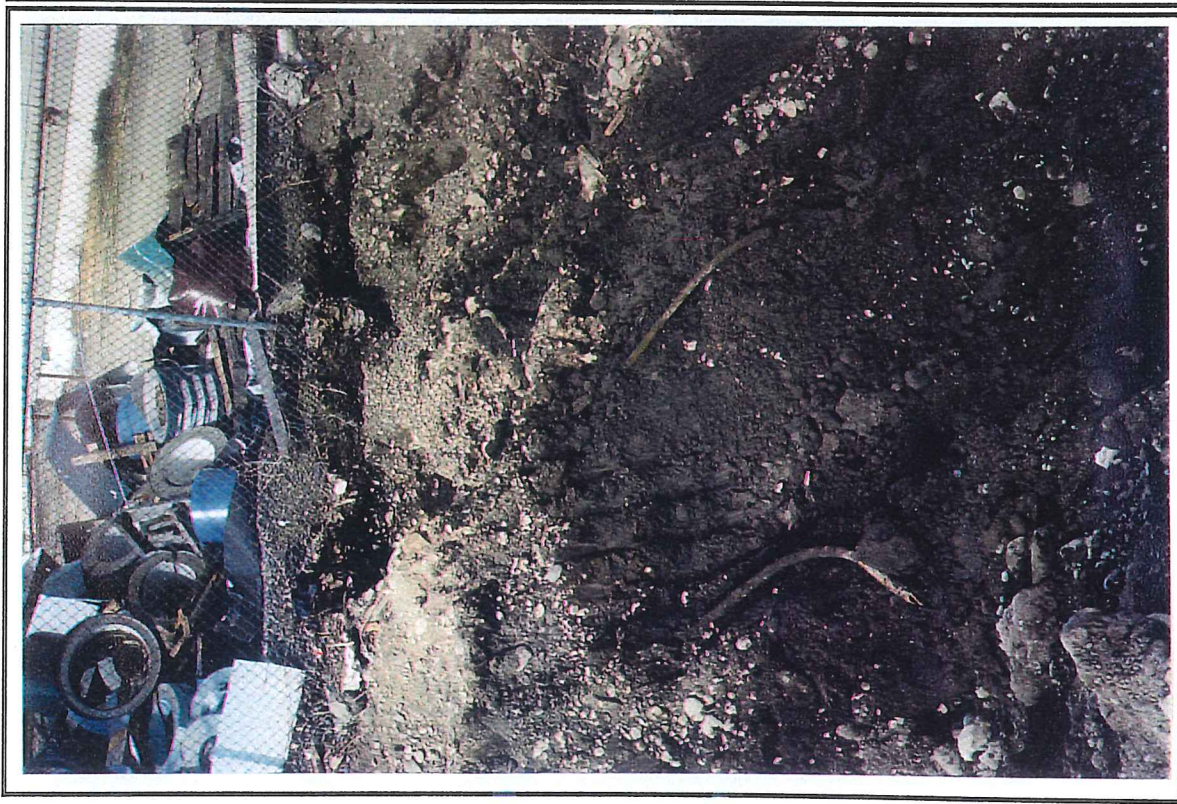
Photo #22: Two water or steam lines unearthed near the northwest corner of the Westwater Construction site, facing northwest. Photo taken on 9/4/01.
