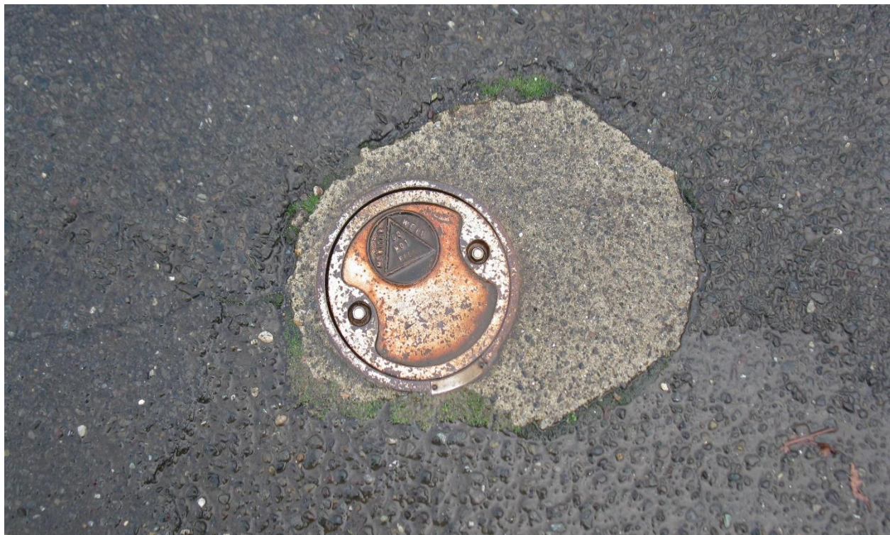
Photo 6: Groundwater Monitoring Well on Sylvia Street.
