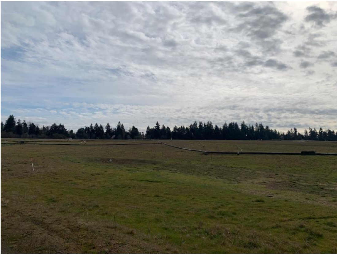
Area of ponding on landfill that requires regrading
