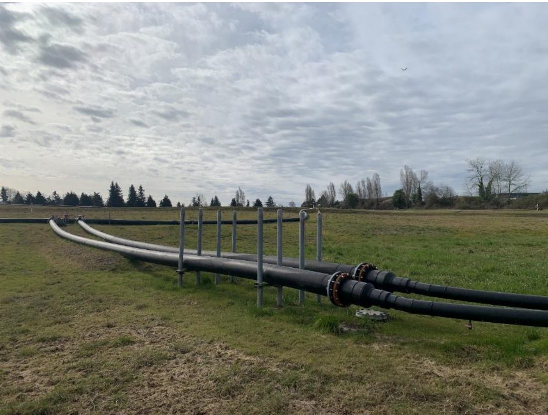
Gas collection infrastructure on landfill
