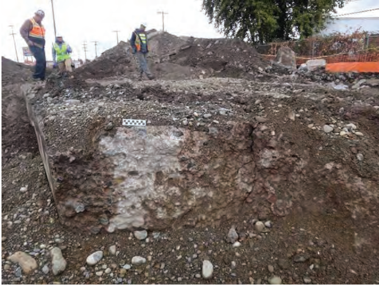
Photograph 2. Historic poured concrete foundation uncovered within eastern project area. Northwest foundation corner, facing southeast.
