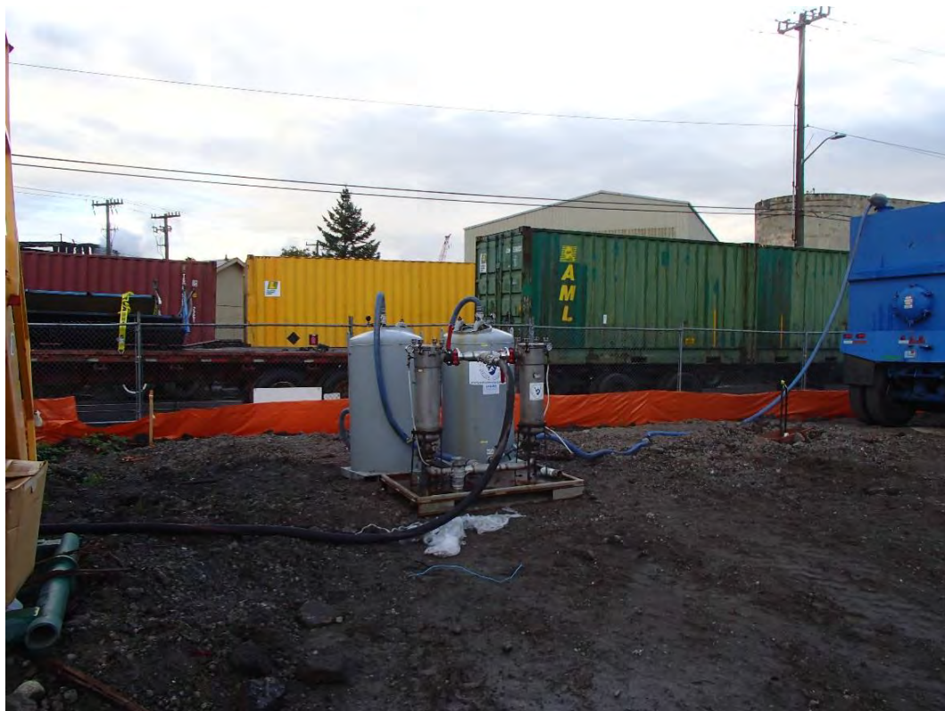
Photograph 16. Dewatering water treatment system bag filters and granular activated carbon vessels
