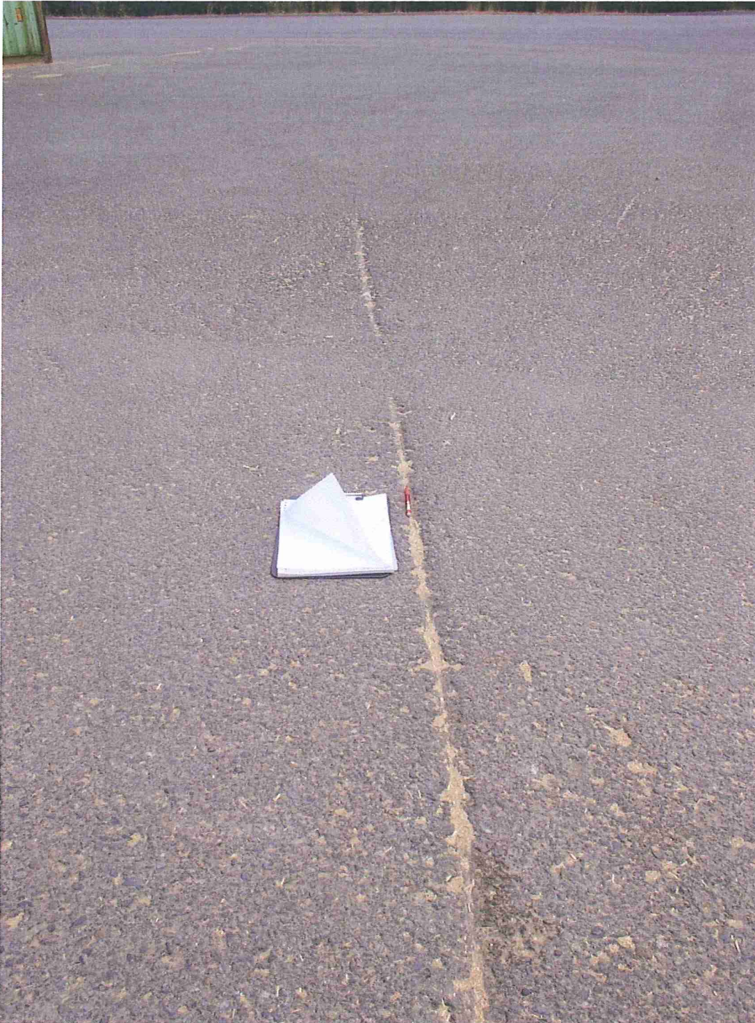
Photo 1: Scratch near the stockpile area with a pencil in the scratch and 8.5" x 11" clipboard for scale.
