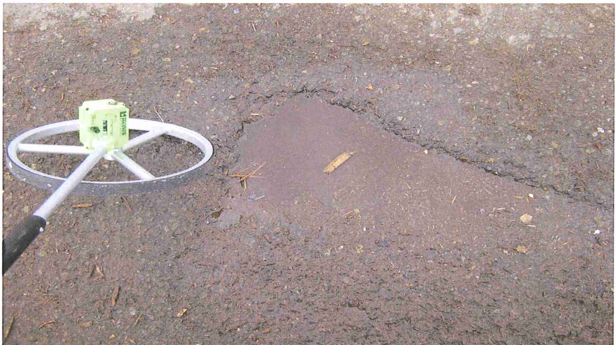
Photo 2: Small rut in pavement
