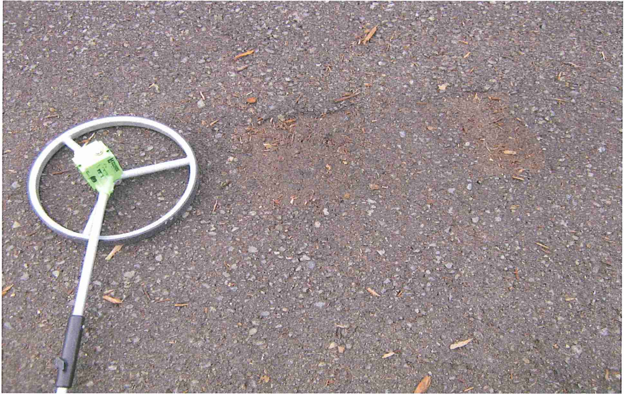
Photo 1: Small rut in pavement
