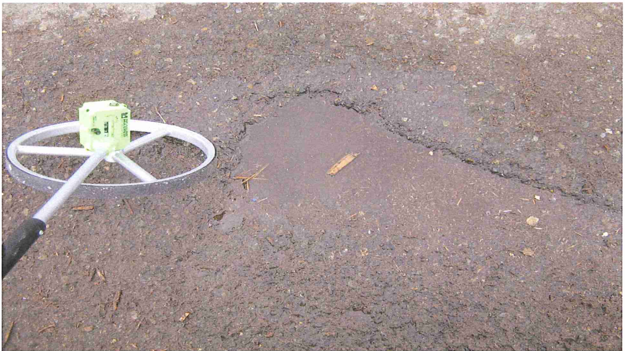
Photo 2: Small rut in pavement
