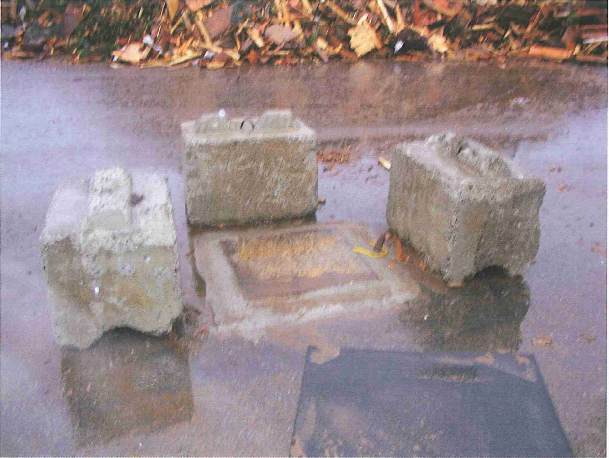
Photo 5: Alteration of well PZ-1A well head to prevent inflow of surface water.
