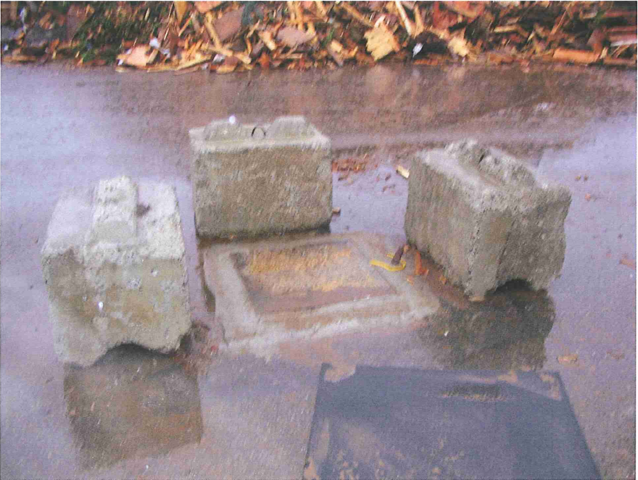
Photo 5: Alteration of well PZ-1A well head to prevent inflow of surface water.
