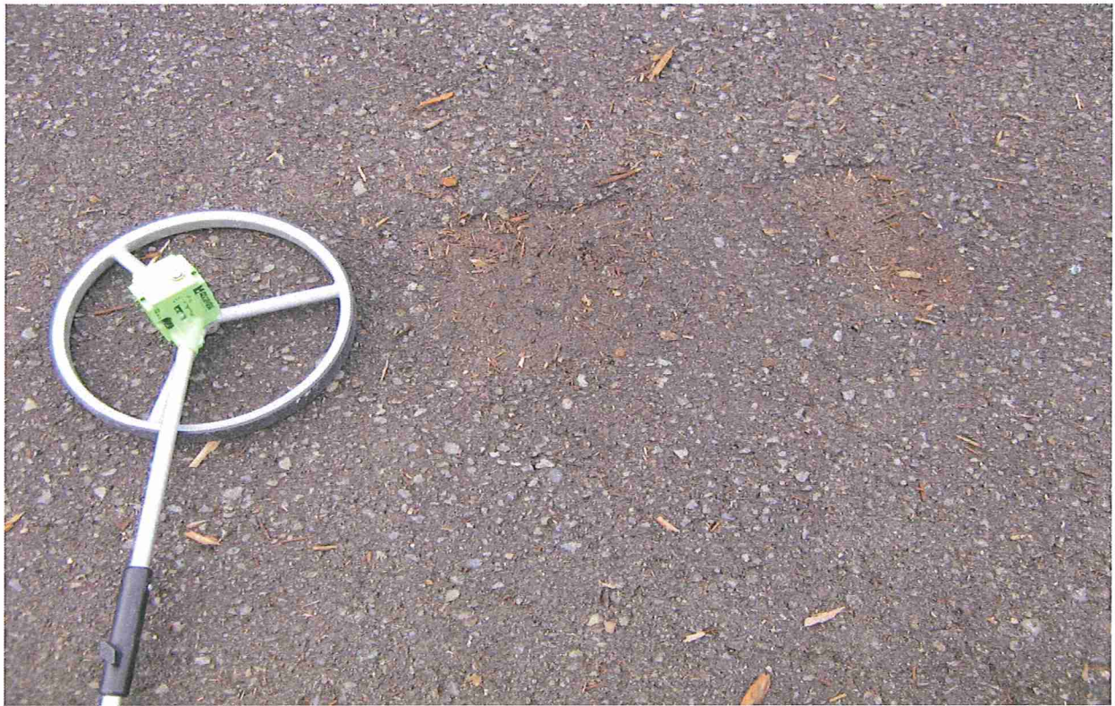
Photo 1: Small rut in pavement
