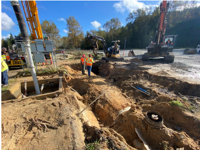
Photograph 1. Standing at east corner of excavation and oriented facing west. At the southwest end of the tank (closest), the fill port and fuel dispenser ports are visible. The two vent ports are at the far end of the tank by the two workers. In the photo, the transformer vault is being cleaned using a vacuum truck and will be eventually supported by the crane present in the left side of the photo during UST removal.
