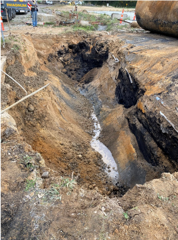
Photograph 3. The tank excavation after removal. Groundwater has begun infiltrating at a depth of approximately 6 to 7 feet below ground surface. The sloughing soil from the northwest sidewall (left hand side of photo) was removed prior to collecting the bottom sample.
