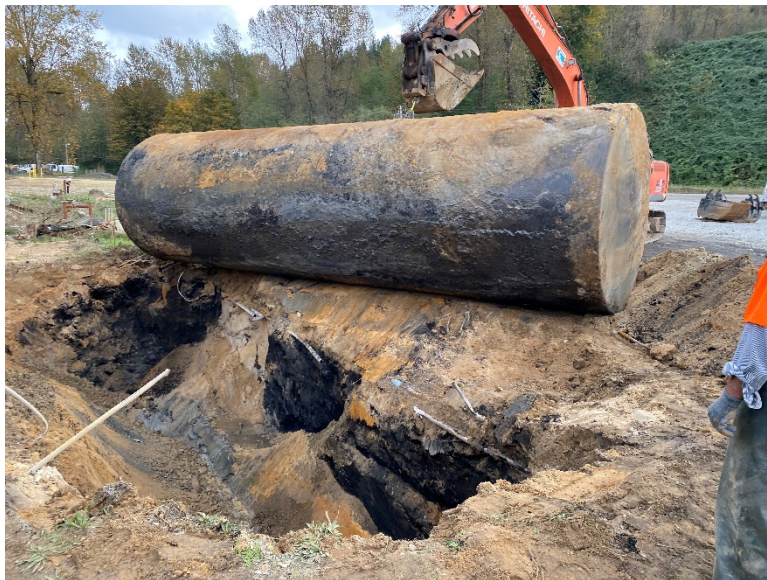
Photograph 2. The UST as it was removed from the tank pit. Photograph taken from the eastern corner of the excavation facing southeast.
