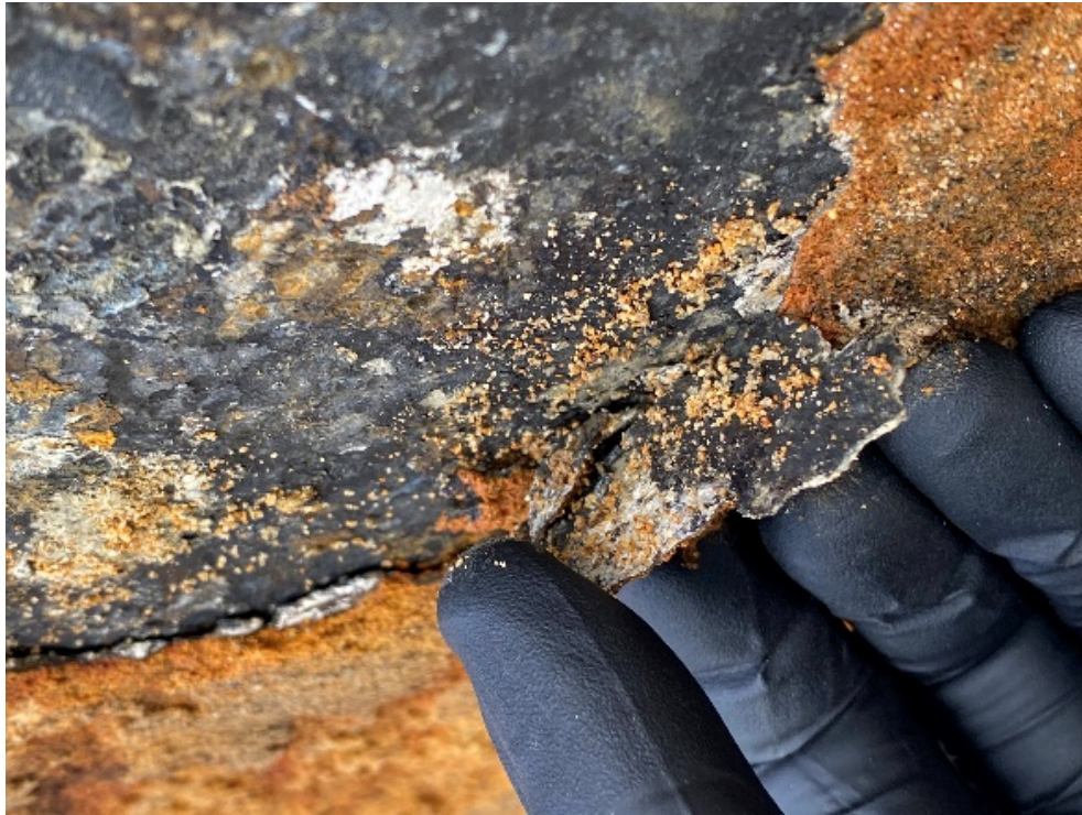
Photograph 4. UST condition on removal. Some scale buildup and small pitting in the steel surface. No visible cracks or holes were noted.
