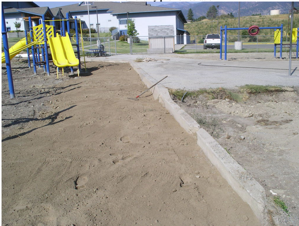
Photo P-2 Manson Elementary play area post-excavation with some clean fill import
