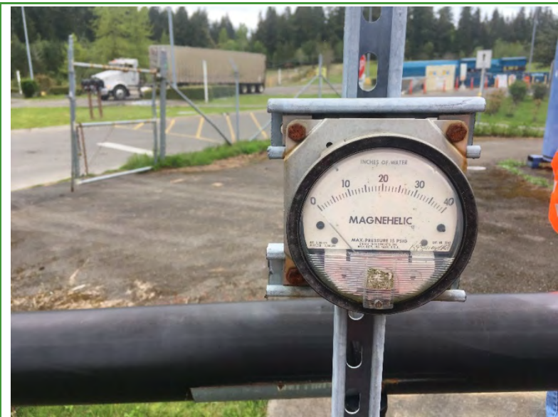
15. Inlet flow reader downstream of diffuser
