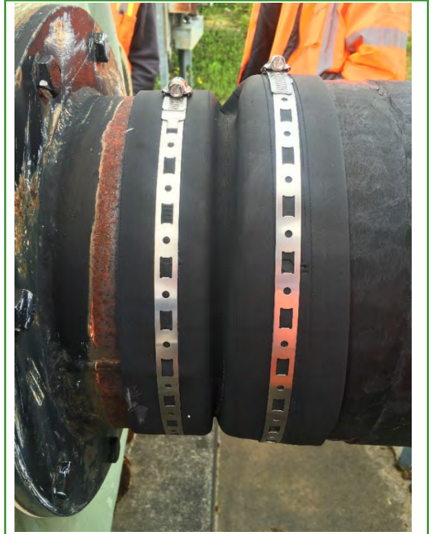
58. Blower inlet flex fitting
