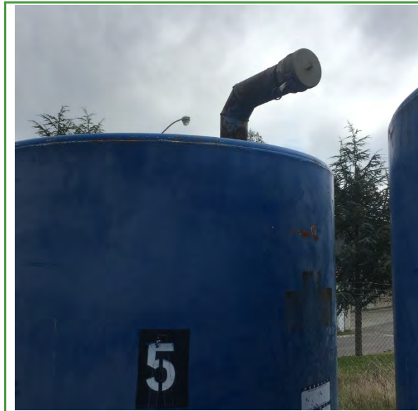
39. Gas outlet fitting
