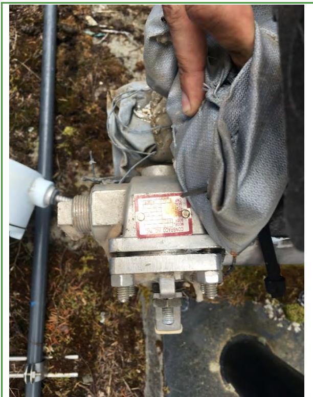
67. Heat traced drain valve
