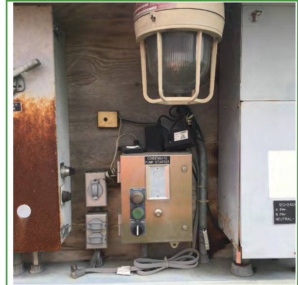
51. Condensate pump control
