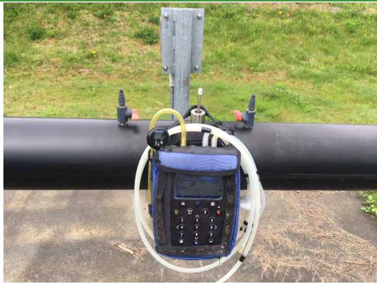
9. Inlet monitoring station
