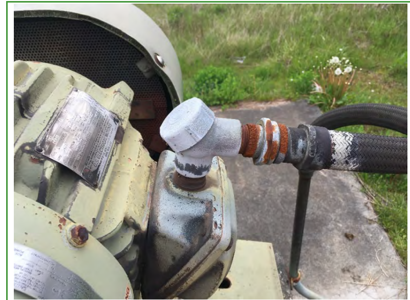
18. Power supply to motor
