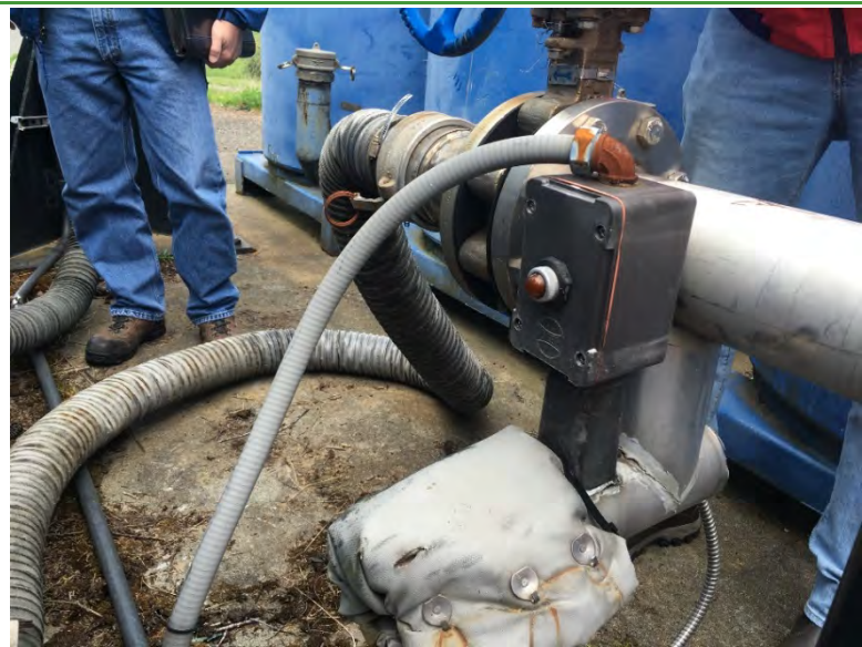
31. Heat traced drain valve
