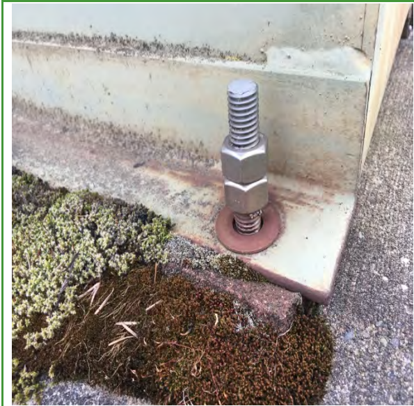
49. Blower pad anchor bolts
