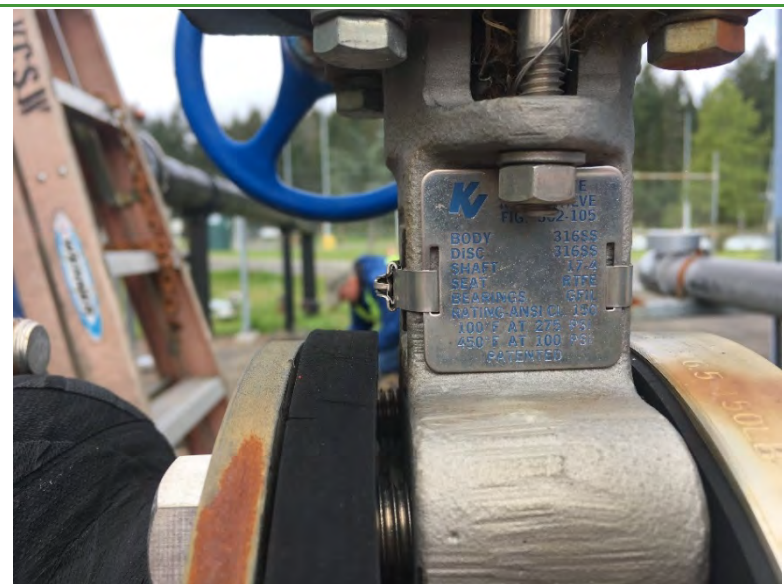
21. Discharge butterfly valve
