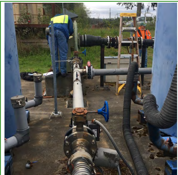
40. GAC inlet hose
