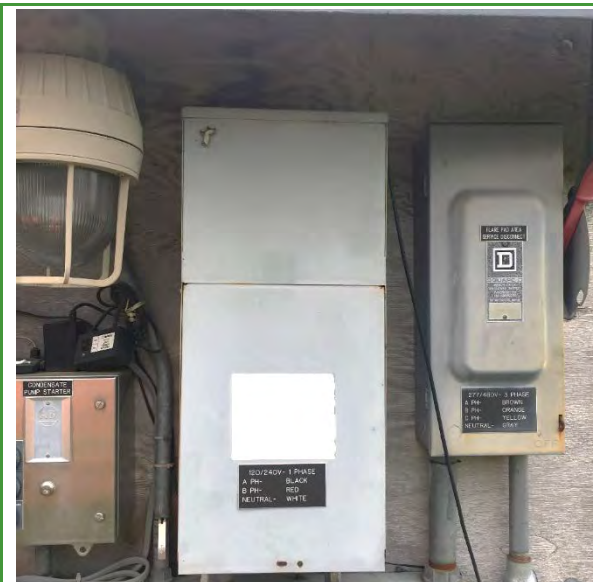
46. Electrical panel showing old weather station wire
