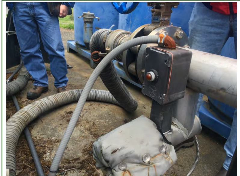
32. Heat traced drain valve
