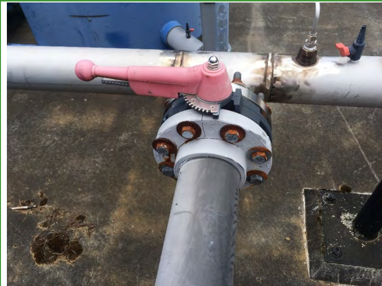
6. Broken valve flange at GAC manifold
