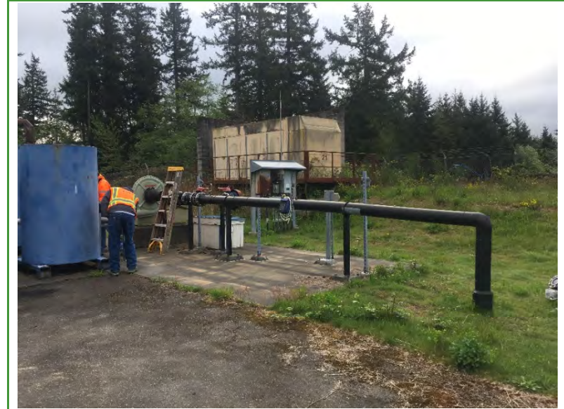
2. Blower inlet piping
