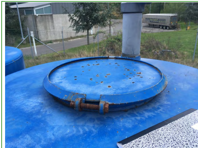
26. GAC vessel hatch
