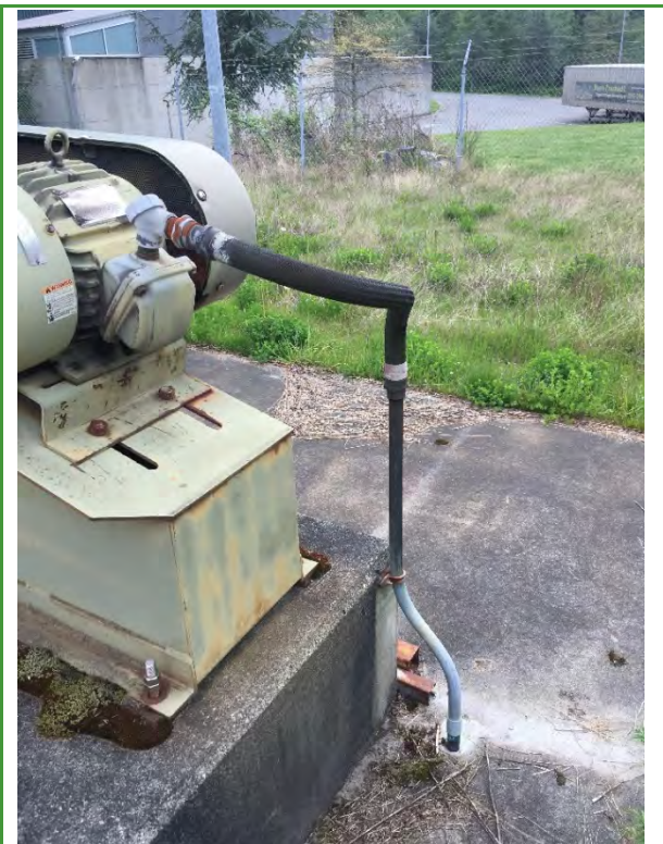
63. Power supply to motor
