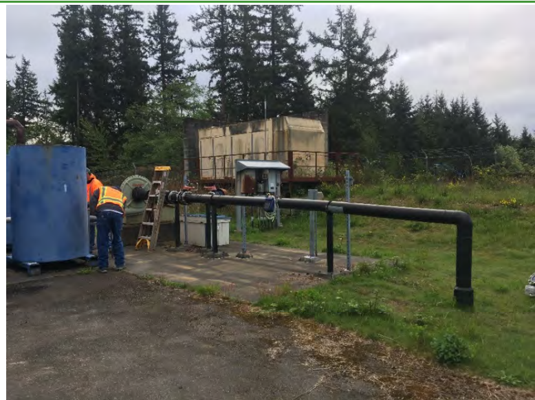
3. Blower inlet piping
