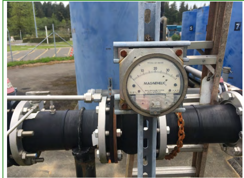
10. Inlet pressure gauge; broken tubing
