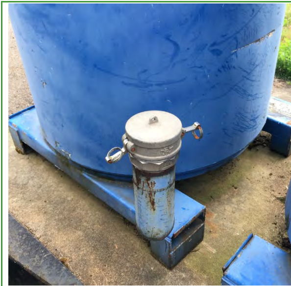
38. GAC inlet fitting
