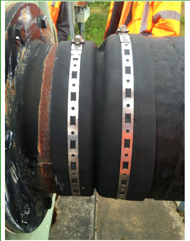
57. Blower inlet flex fitting
