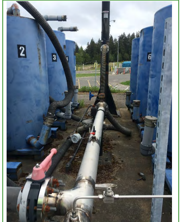
70. GAC stainless steel 4-inch manifold
