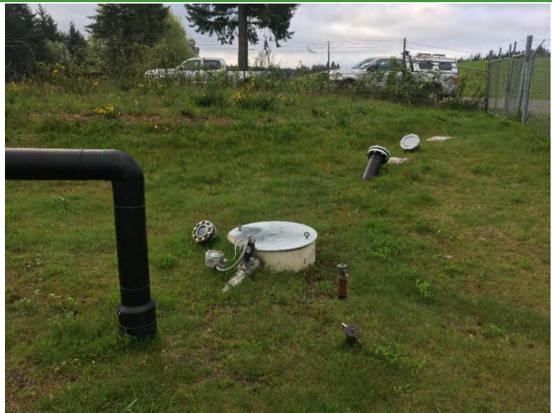
5. Knockout and condensate pump
