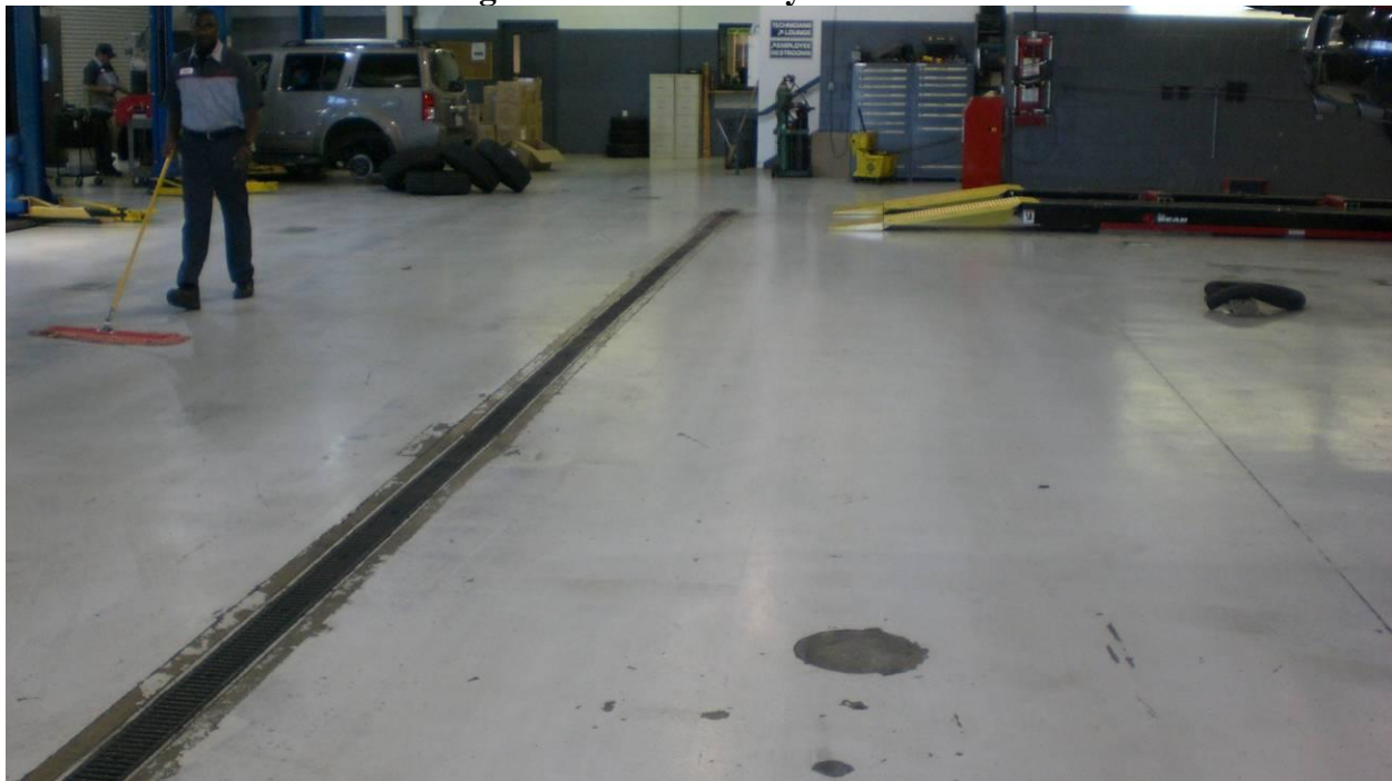
Photo 2: Abandoned Monitoring Well in Service Bay – from the east
