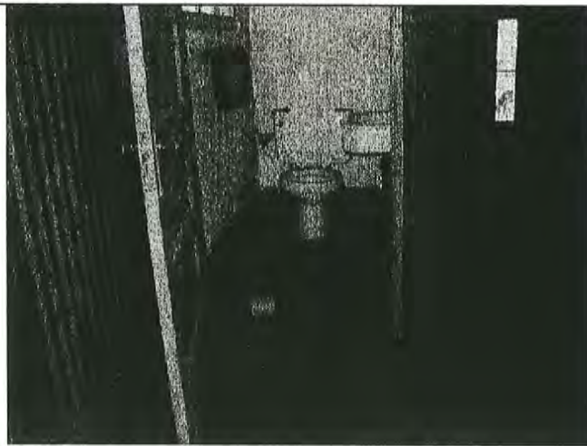
Photo 3: Bathroom Floor Tile
