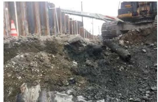
An abandoned heating oil tank.
