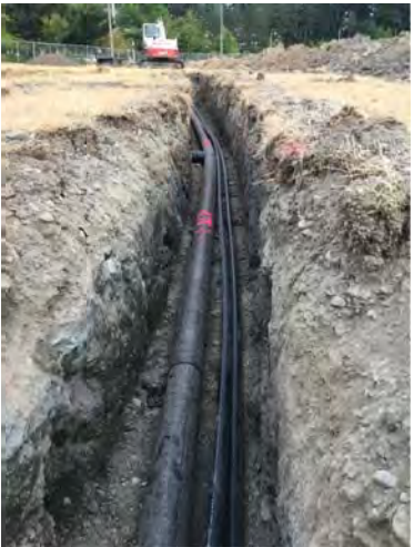
6"Ø GAS, 2"Ø CONDENSATE & 2"Ø AIR SUPPLY PIPE
