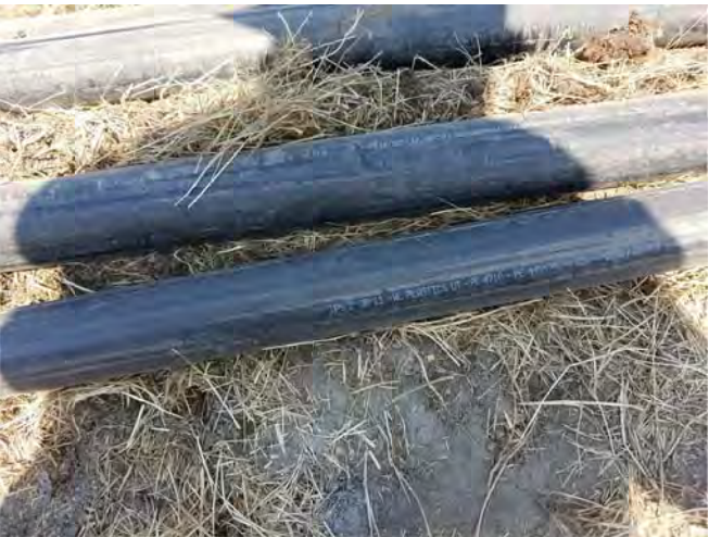
SDR OF 2"Ø CONDENSATE & AIR SUPPLY PIPE
