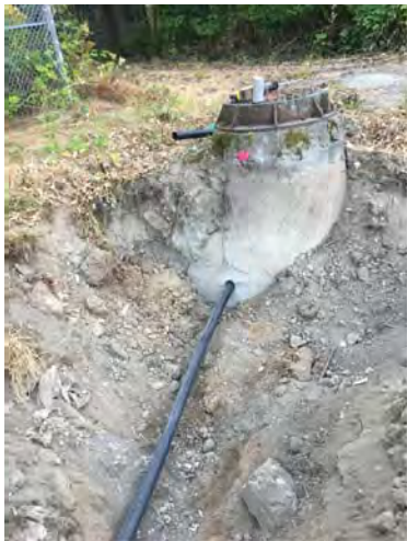
CONDENSATE PIPE CONNECTION TO SEWER PIPE
