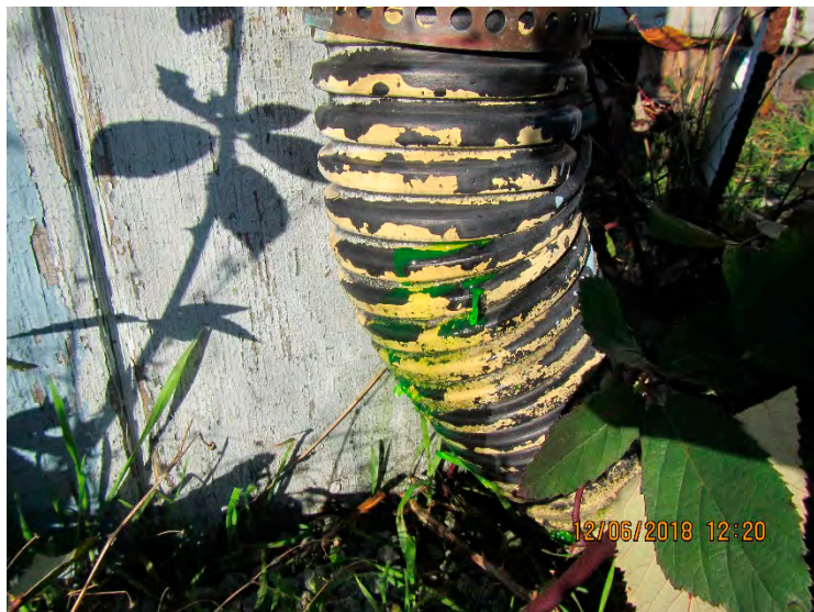
Photograph 15: Visual confirmation of dye solution leaking from the roof drain located at the northeast corner of the Woodworking Shop, approximately 20 feet downgradient from the central roof drain where dye solution was injected.
