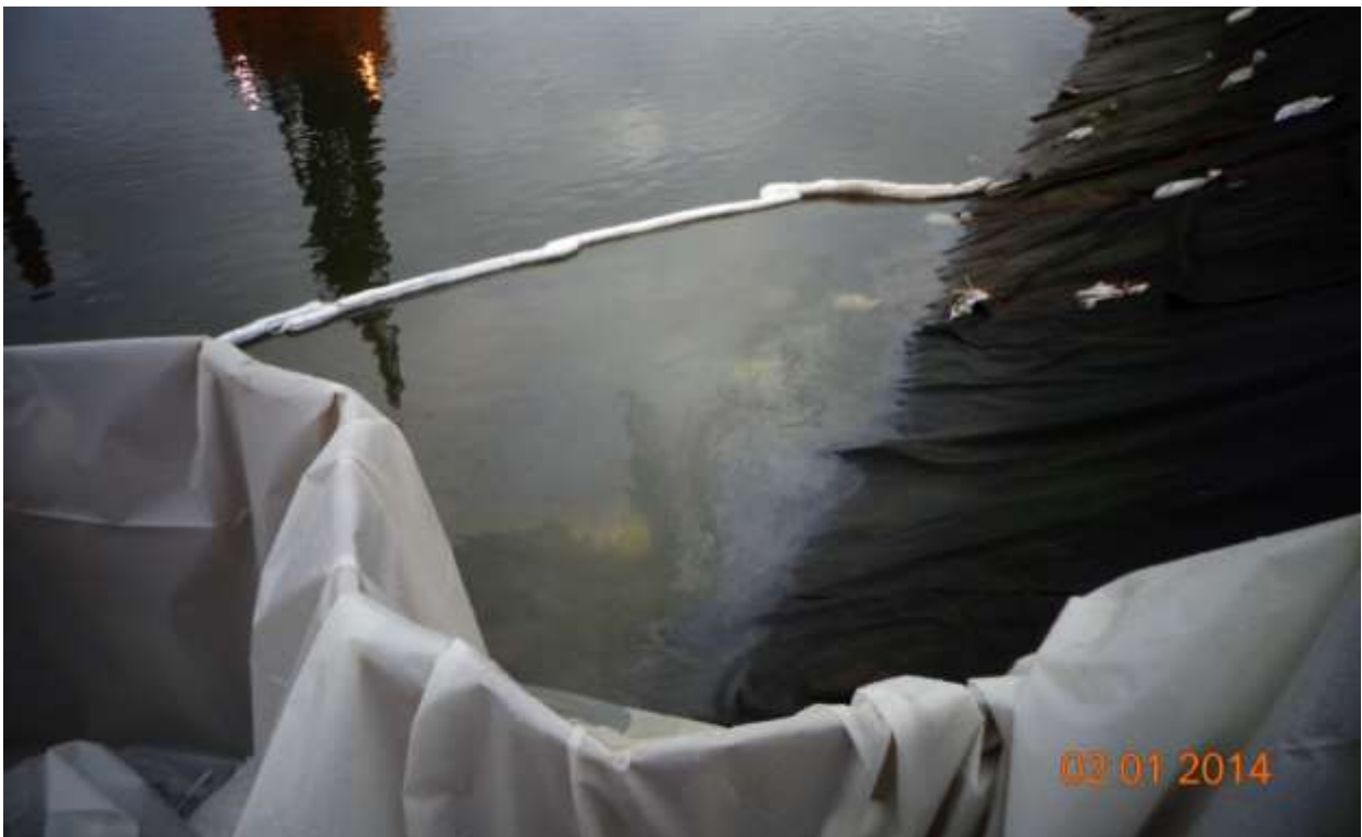
Photo 2: Sheen in DU3 observed lingering near southeast corner of the South Park Marina looking south (sheet pile wall in foreground), 2/1/14, 16:11 (source: AECOM)
