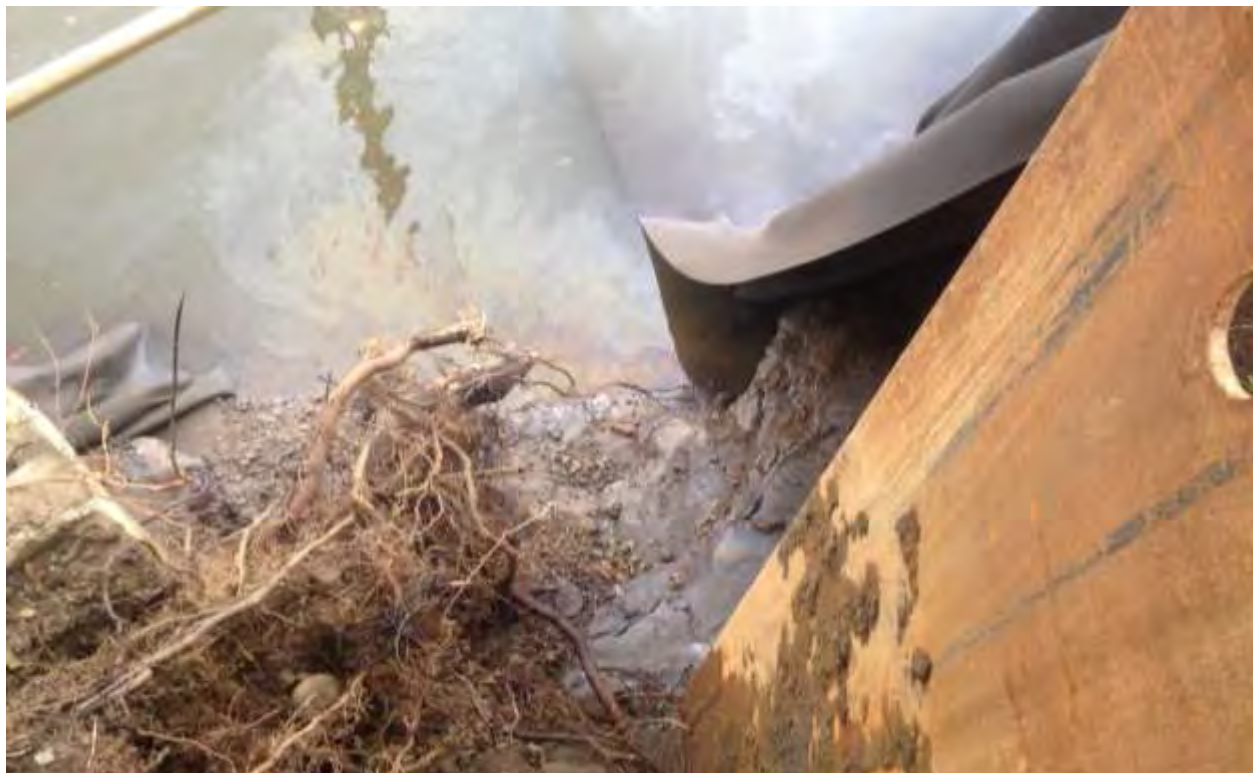
Photo 4: Sheen at base of sheet pile wall at the southeast corner of the South Park Marina, looking down, 2/21/14, 12:25 (AECOM)
