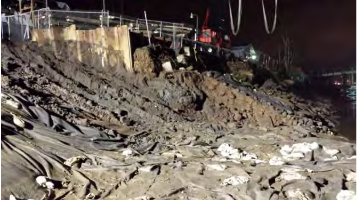
Photo 1: Excavation of North Bank A at corner of South Park Marina, 1/4/14, 00:21 (source: AECOM)
