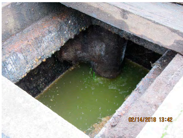
Photograph 2: Visual confirmation of fluorescein dye solution discharging from CB-01 to the sanitary sewer vault.
