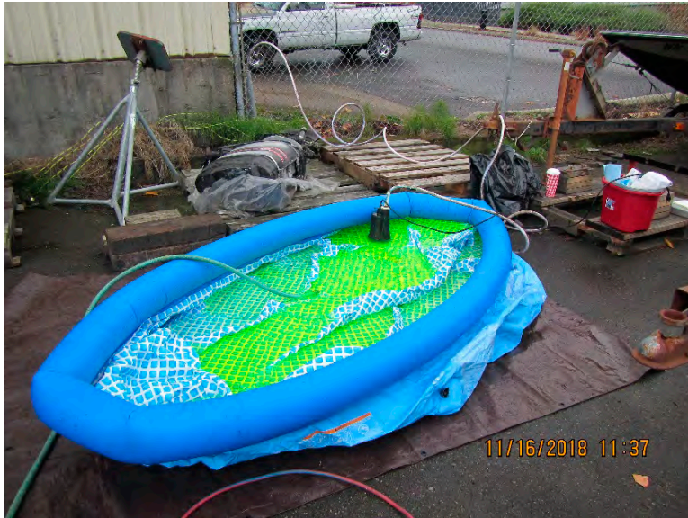
Photograph 11: Pumping dye solution into the roof drain located the northwest corner of the SPTF shop.
