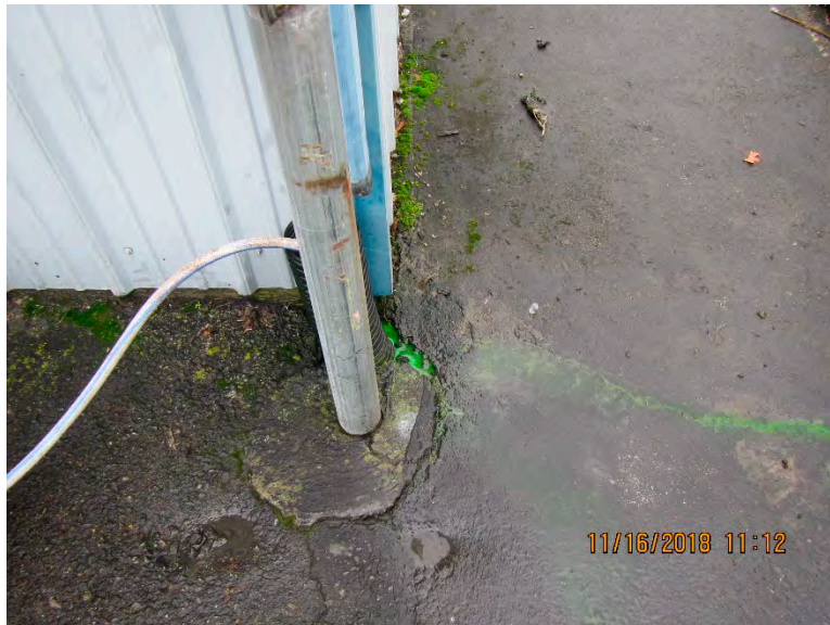
Photograph 9: Pumping dye solution into the roof drain attached to the northeast corner of the RMM Shop. Note the seepage of dye solution through cracks in the asphalt.
