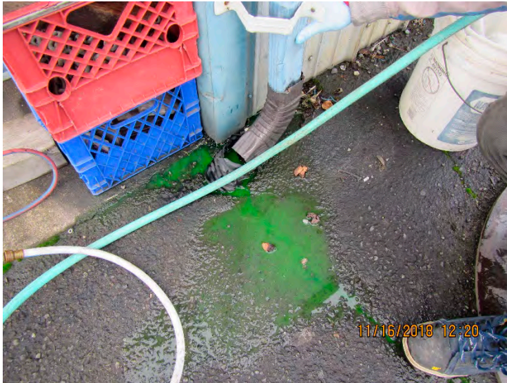
Photograph 13: Refusal of dye solution into clogged subsurface piping associated with the roof drain located at the southeast corner of the RMM Shop.
