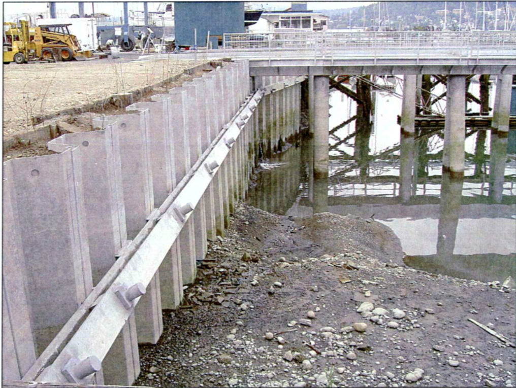
26. Segment B bulkhead and tieback system.
