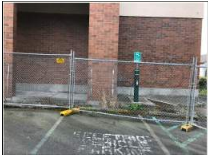
22. View of electric vehicle charging station
