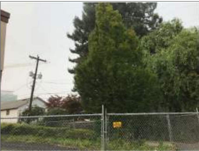
21. View of adjacent pole-mounted transformers
