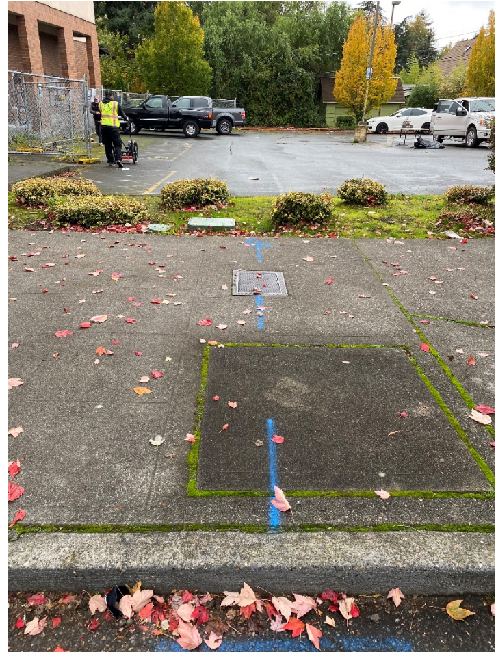
Prior to drilling, a private locator cleared all boring locations. Pictured is the locator using GPR to clear boring locations for GSB-1 and GSB-2.
