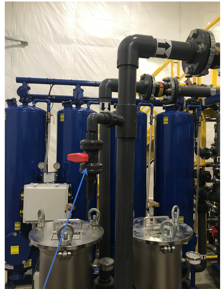
Final Effluent Sampling Station Sampling located after bag filters, prior to valves controlling flow to infiltration basin, wetlands return, or fire pond.
