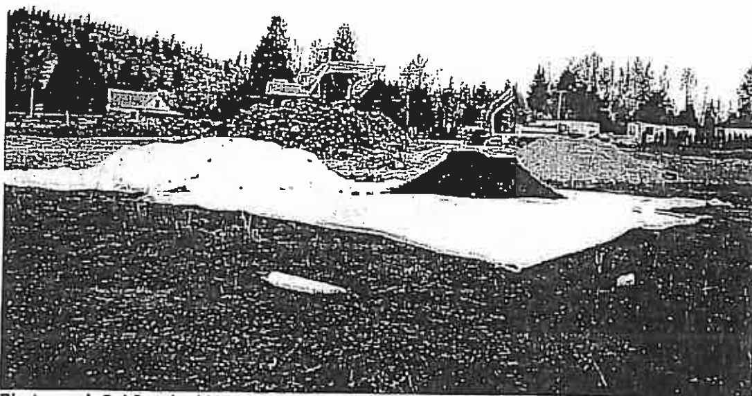
Photograph 8. View looking over the area of stockpiled soil. The petroleum-impacted soil is in the foreground; soil excavated from the area of the former dry cleaner area is in the background. Soil from the UST excavation was later placed to the west of the visible stockpiles.
