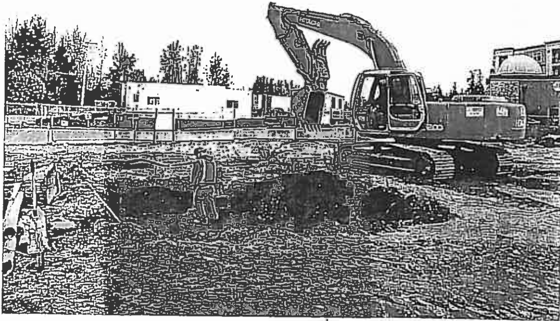
Photograph 3. View of excavation in progress in the area of the previously stockpiled-PCS.
