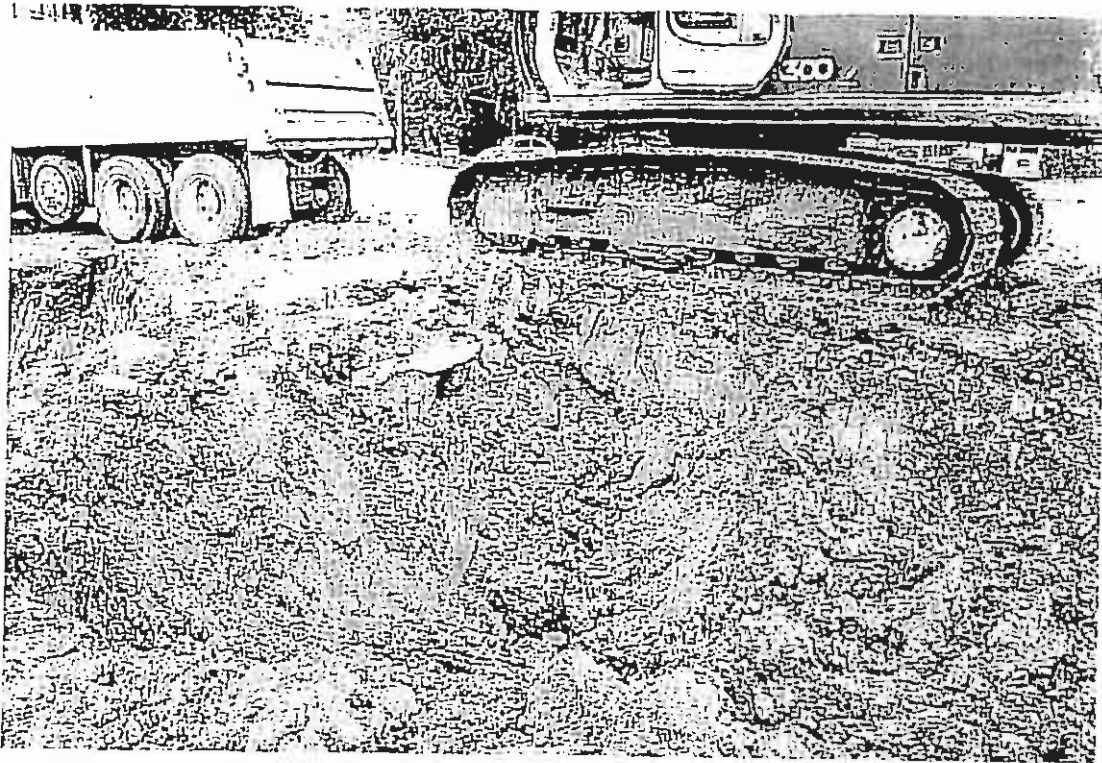
Photograph 5. View of the excavation after removal of the UST. Note area of gray-colored PCS.
