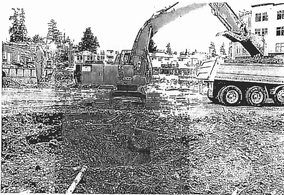
Photograph 1. View of the excavation in progress in the area of the former dry cleaners.
