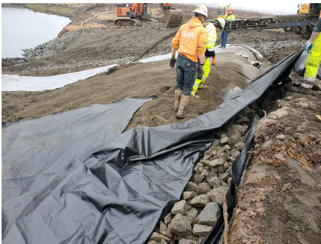
Photograph 19: Keying in the RCM and geotextile at the top of the slope.
