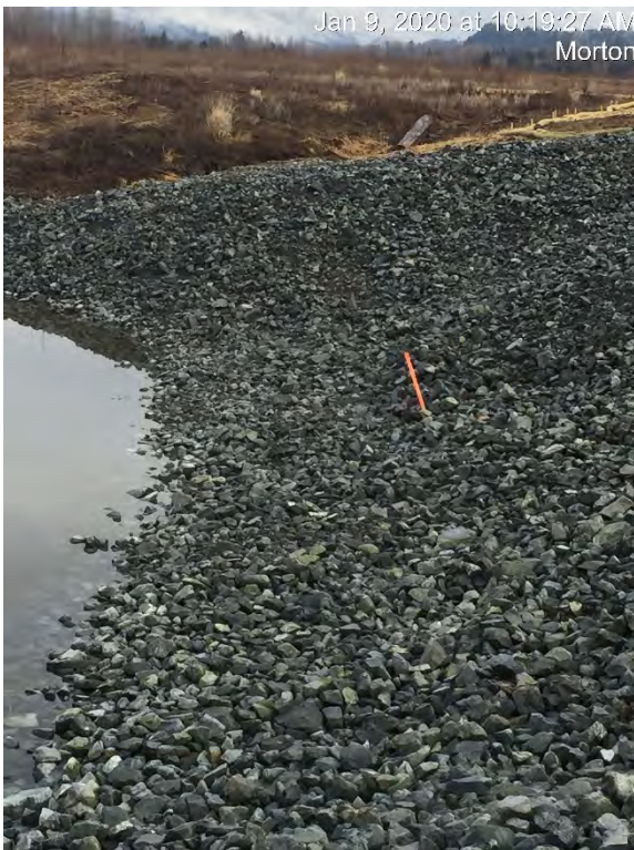
Photograph 22: Completed cap and elevated water level. View looking east, towards the former ravine drainage area.
