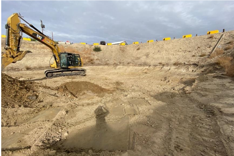
Looking northwest - northern portion of excavation. Average depth of approximately 1 to 20 feet bgs.
