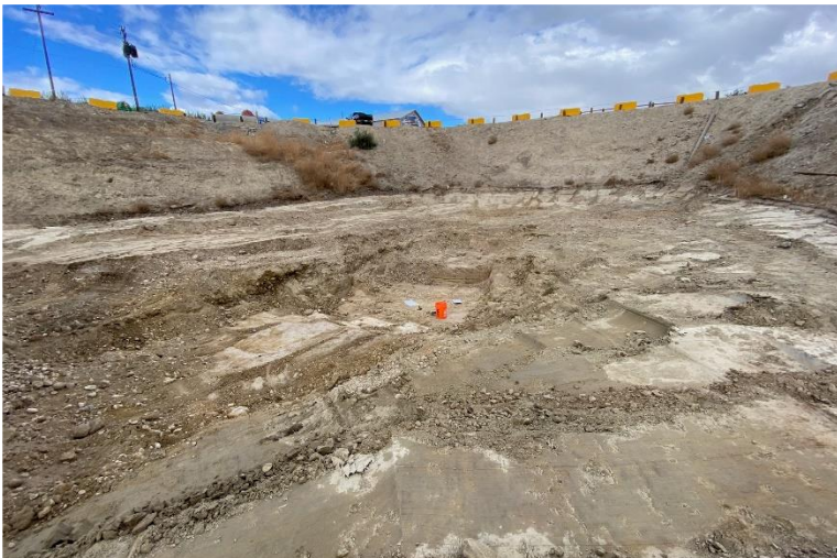
Looking northwest - excavation observed with localized areas in central portion excavated to approximately 4 to 9 feet bgs.
