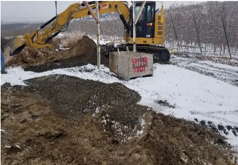
Looking west – Site location of smudge pot storage area with gravel overburden. Water piping for mixing chemicals is present. (12/03/19)
