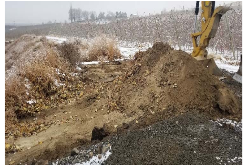
Looking west – Initial excavation of east side of site. Orchard located to the north. (12/03/19)
