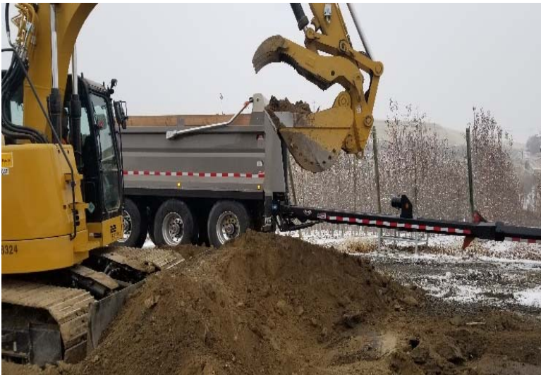
Looking north – Excavator loading gravel overburden and contaminated soil into Columbia Asphalt truck with trailer. (12/03/19)
