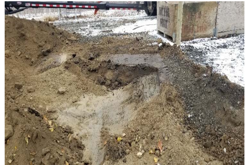
Looking north – Discoloration, odor, and diesel spillage identified. (12/03/19)
