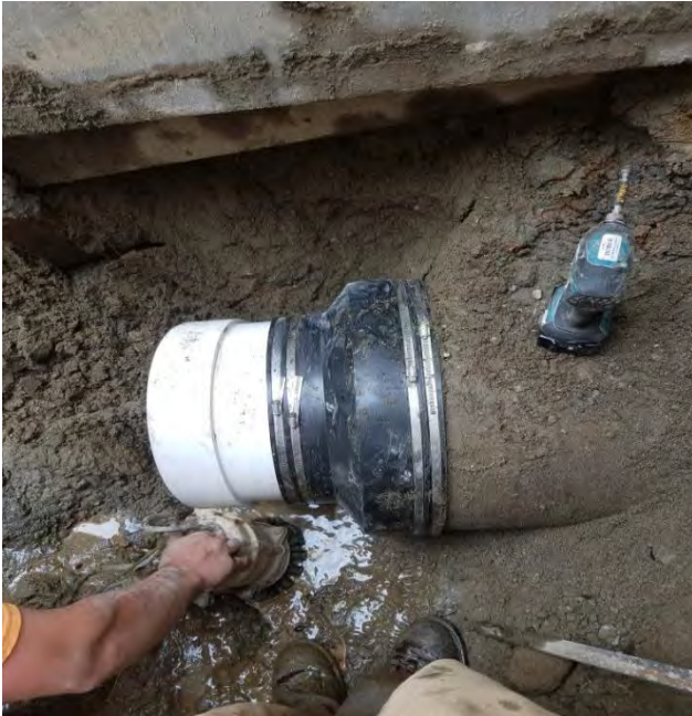
Photograph 3. Pipe K with “Fernco” removable plug attached.
