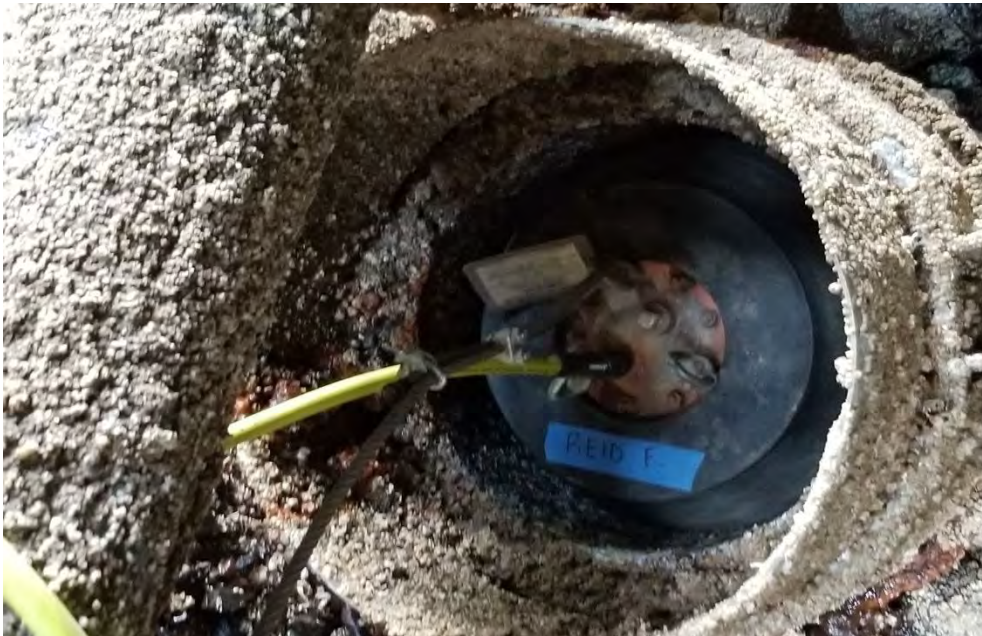
Photograph 1. Pipe K outfall under wharf with temporary pneumatic plug.
