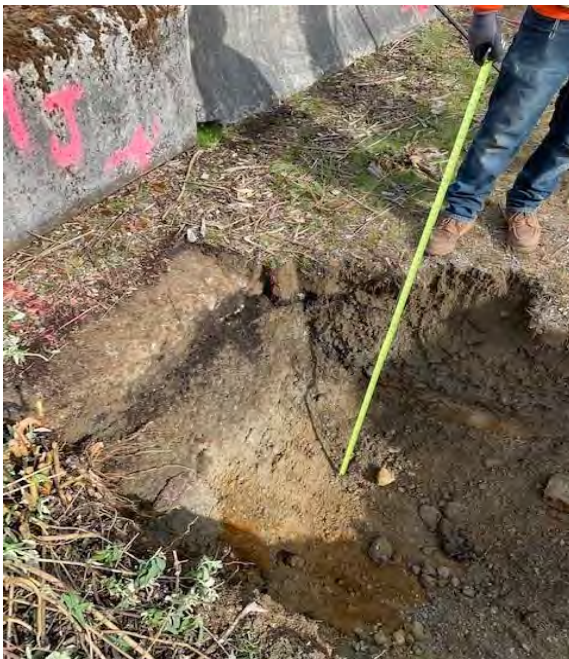
Photograph 2. Pipe J location excavated to 4.5 feet on west side of ecology block wall.
