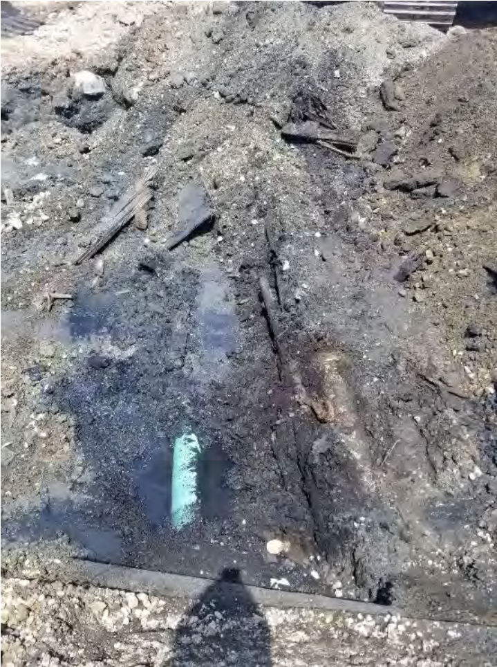
Photograph 5. Initial observation of Bunker C fuel pipe and utility pipe near south end of excavation.
