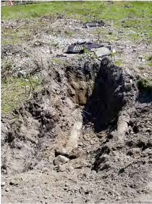
Photograph 1. Catch basins for B1 (background) and B2 (foreground), with downstream B2 pipe initially exposed.
