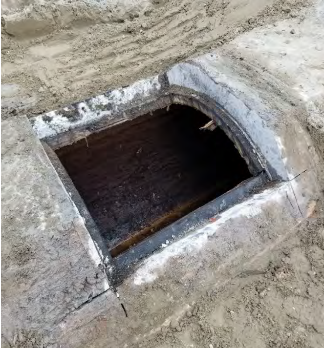
Photograph 7. Pipe F breached 75 feet east of bulkhead.
