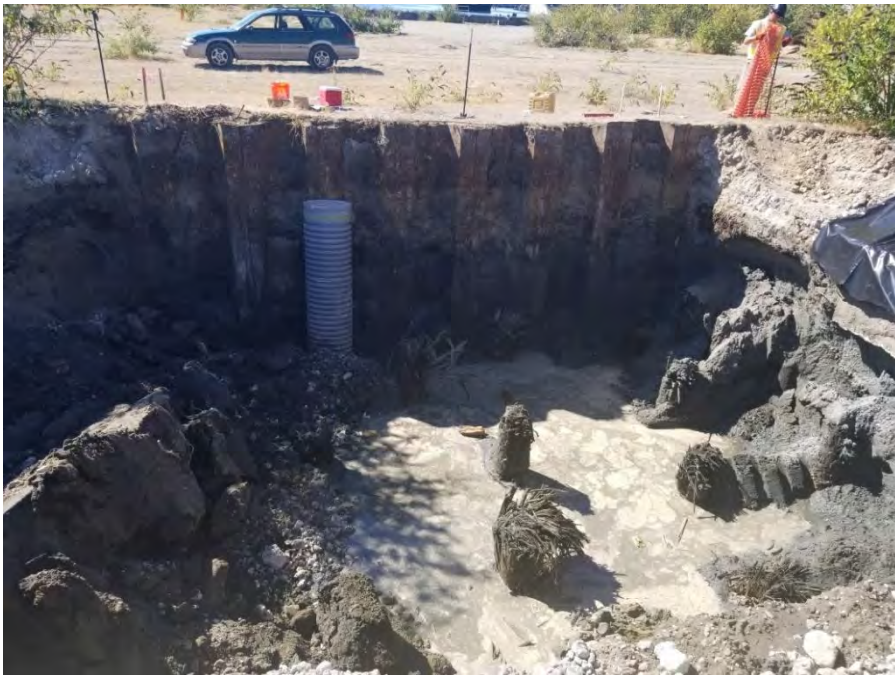
Photograph 2. Initial excavation limits on 8/28/2020 with sheet pile wall on west sidewall, view looking west.
