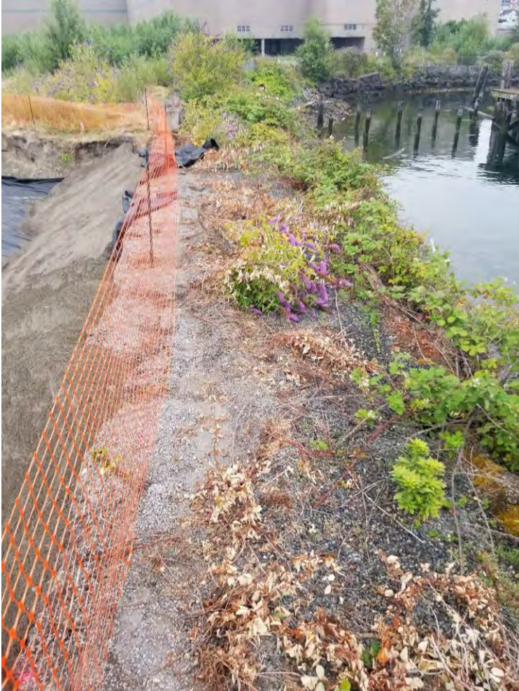
Photograph 9. Southern sidewall showing top of shoreline bank after second overexcavation, looking east.
