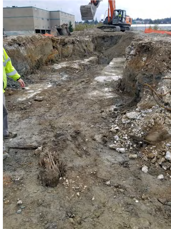
Photograph 13. View from west leg of BBH Area looking at connector segment to GFB12 Area in the background, looking south. Concrete on both sidewalls and base.
