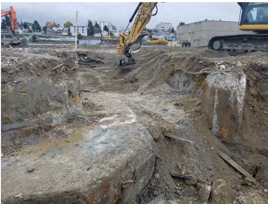
Photograph 8. Excavation extension between south leg of BBH Area (in background) and GFB12 Area (in foreground), view looking east, concrete structure comprising north sidewall evident in lefthand side of photo.
