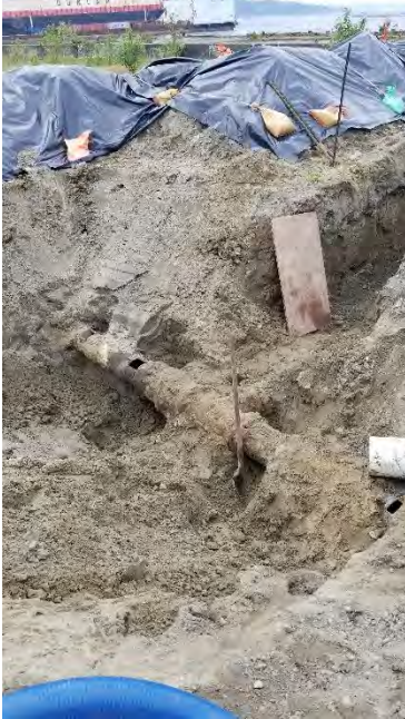
Photograph 3. Section of pipe E left in ground, preplugging.
