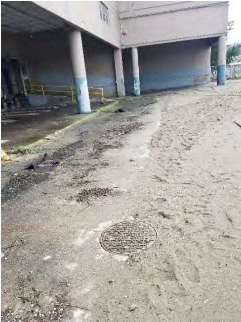
Photograph 1. Manhole D in foreground, Catch Basins C and B, respectively, in background, looking south.
