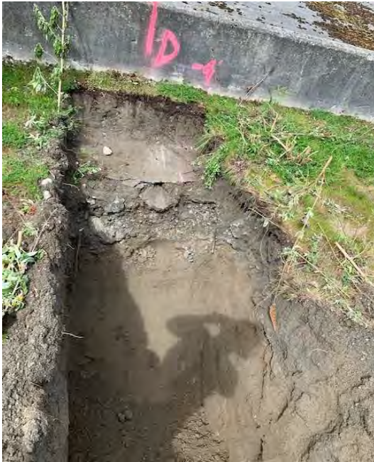
Photograph 1. Pipe D not observed at west end of ecology block wall, adjacent to bulkhead (it is plugged 18 inches east of bulkhead)
