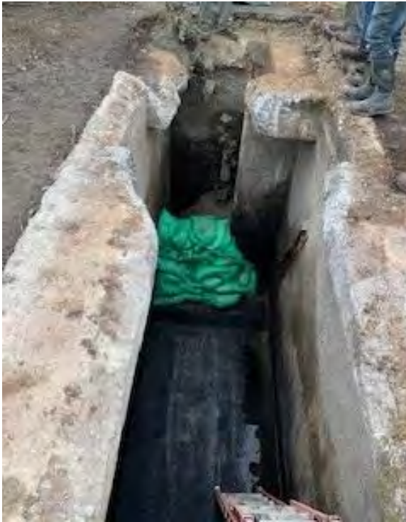
Photograph 5. Sandbags placed to confine area of CDF placement around sealed pipe entry/exit points, and, thus avoid, filling entire vault bottom with CDF.
