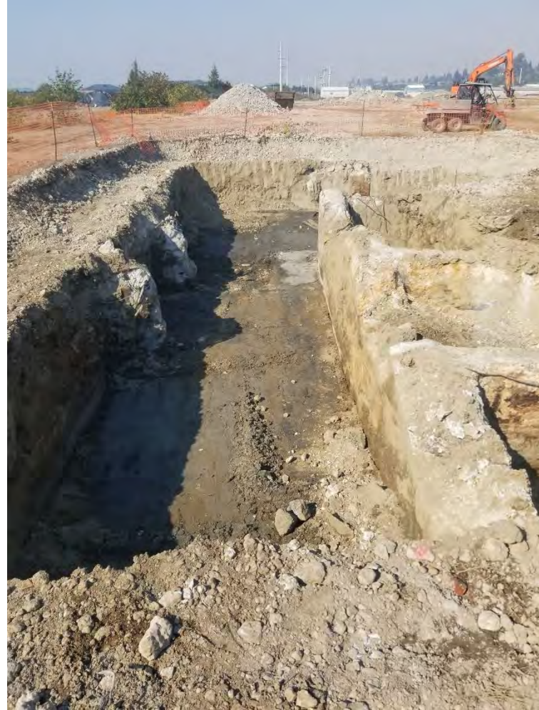
Photograph 2. Western end of western extension of BBH Area excavation, view looking north.
