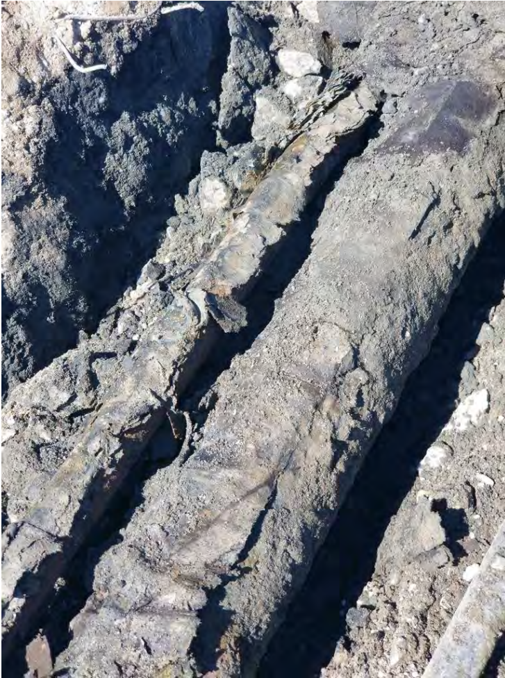
Photograph 14. Initial observation of fuel pipes near northwest corner of excavation.
