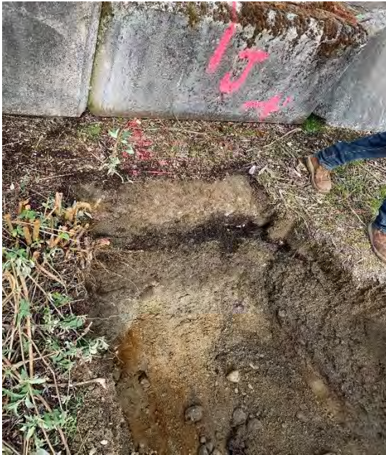
Photograph 1. Pipe J not present on west side of ecology block wall adjacent to bulkhead. Pipe plugged 16 feet east of bulkhead.
