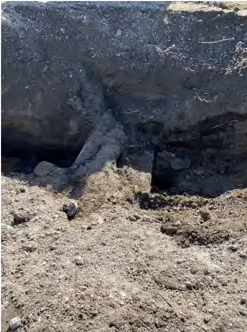
Photograph 1. Pipe M exposed 75 feet inland; concrete covering encountered on the wood stave pipe was partially intact.
