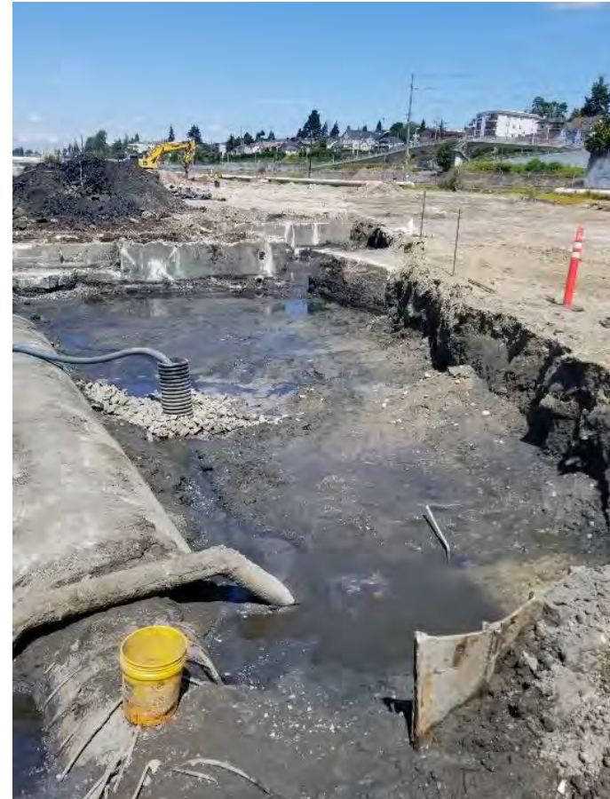
Photograph 4. Same as Photograph 3, but looking north. East-west-trending sheet pile wall in foreground.
