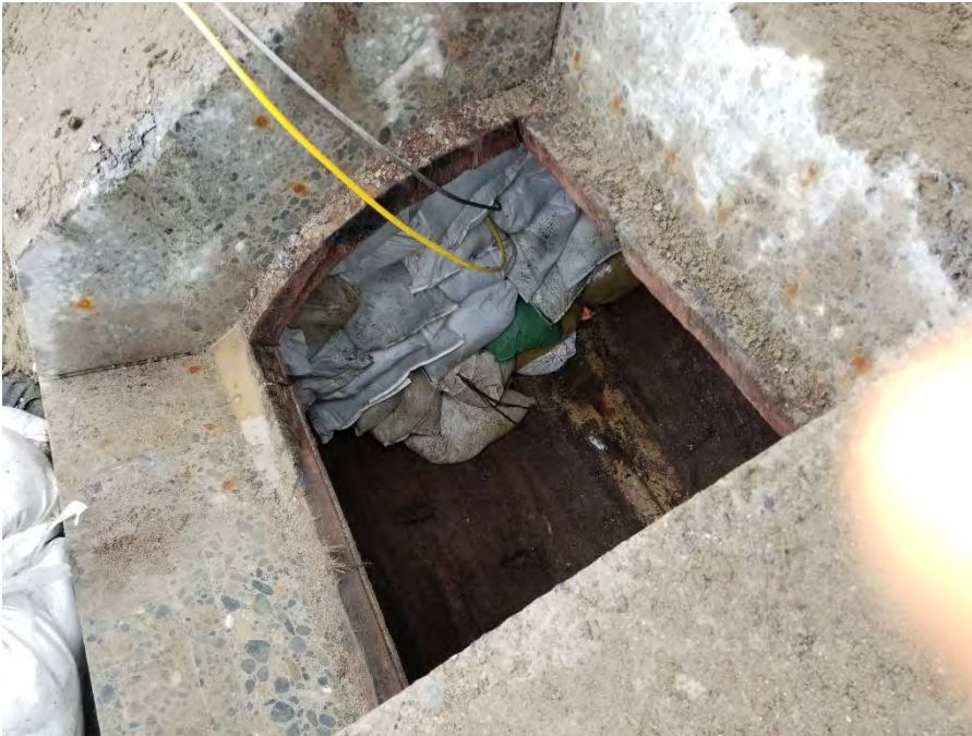
Photograph 11. Sandbag wall in place at 15-foot breach. Air line and cable for pneumatic plug visible.
