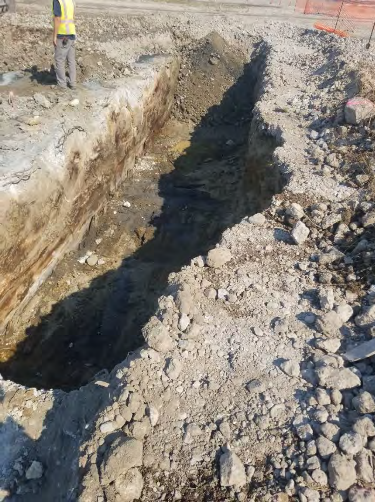
Photograph 3. Eastern end of western extension of BBH Area excavation, view looking east.
