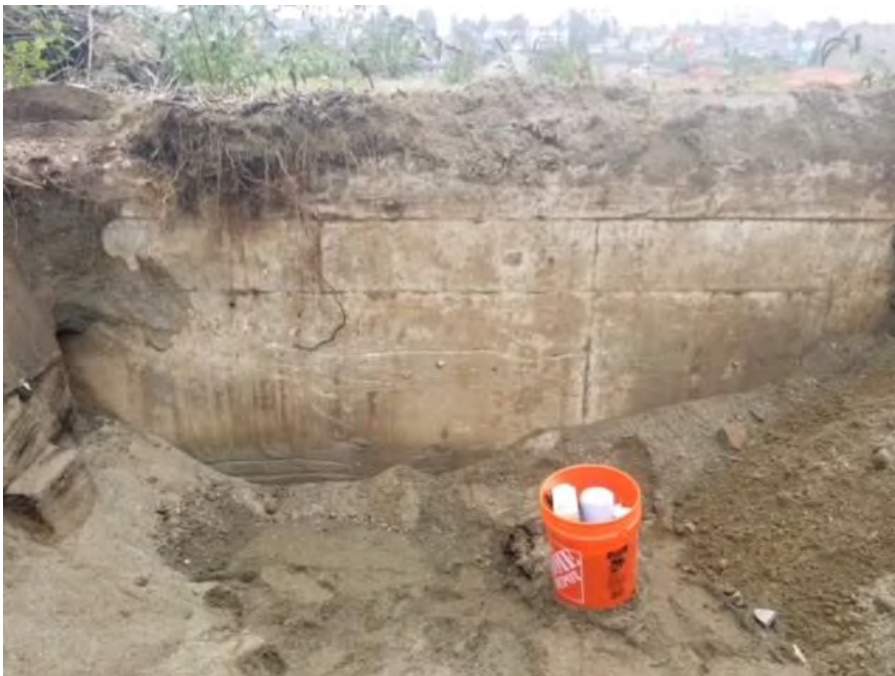
Photograph 2. Eastern wall in initial excavation, 10/5/2020, view looking east. Note treated timbers in north sidewall (left side of photo)
