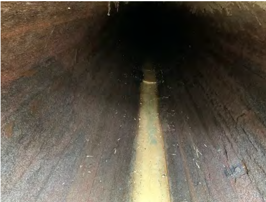
Photograph 8. Interior of Pipe F near 15-foot breach.
