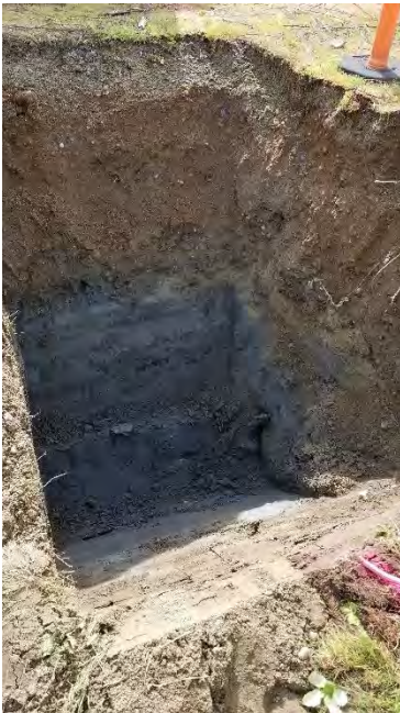
Photograph 2. Excavation for pipes Q1 and Q2 (collocated), ~7 feet east of bulkhead, no pipes found.
