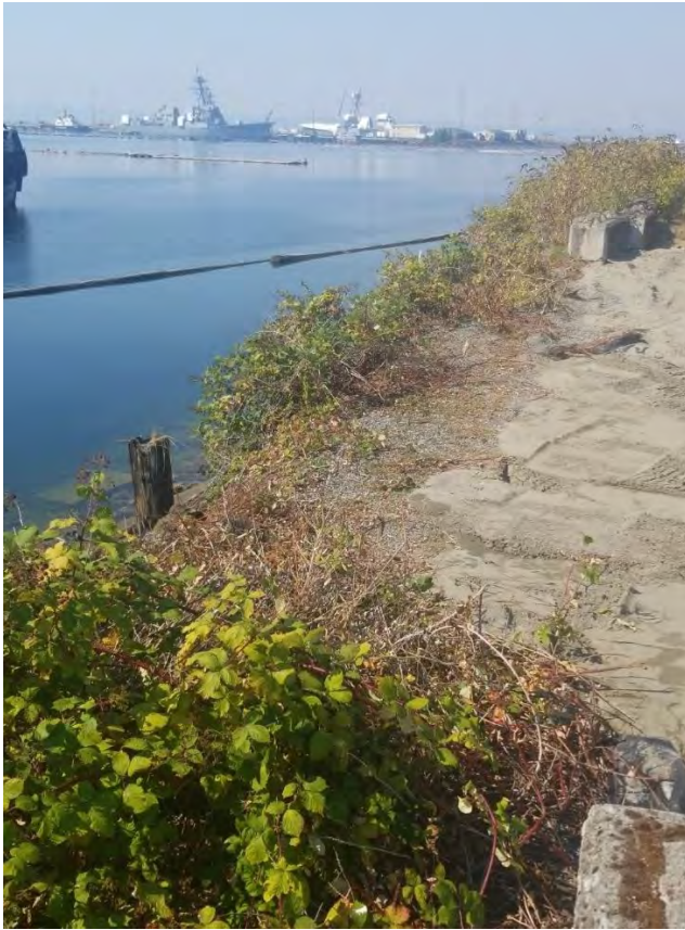
Photograph 12. Southern sidewall and shoreline bank, including remnants of wooden bulkhead, after third overexcavation on 8/27/2020.
