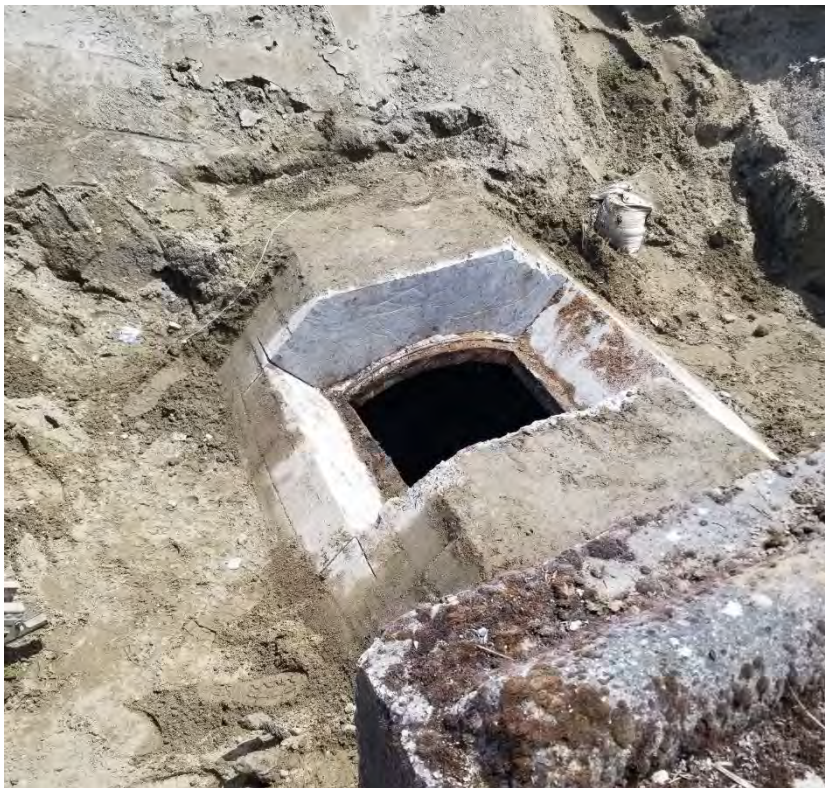
Photograph 6. Pipe F breached 15 feet east of bulkhead.
