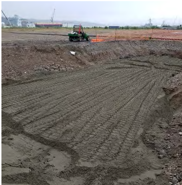
Photograph 4. Hydraulic Barker excavation backfilled to surrounding soil grade (beneath adjacent CM awaiting removal).
