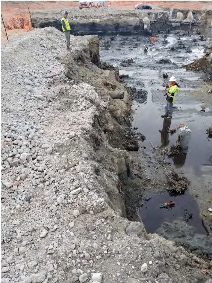
Photograph 12. View from NE corner of north leg, looking south into main part of BBH Area excavation. Concrete in eastern portion of south sidewall is evident in background.
