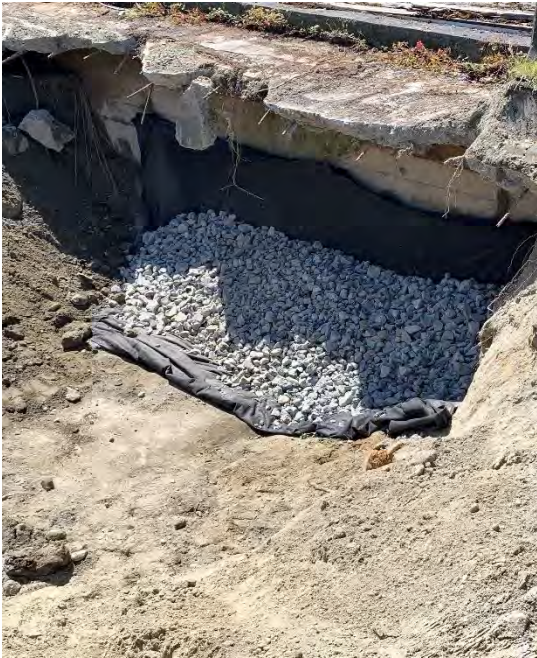
Photograph 3. Pipe F at bulkhead, fabric and quarry spalls placed to stabilize materials around void.
