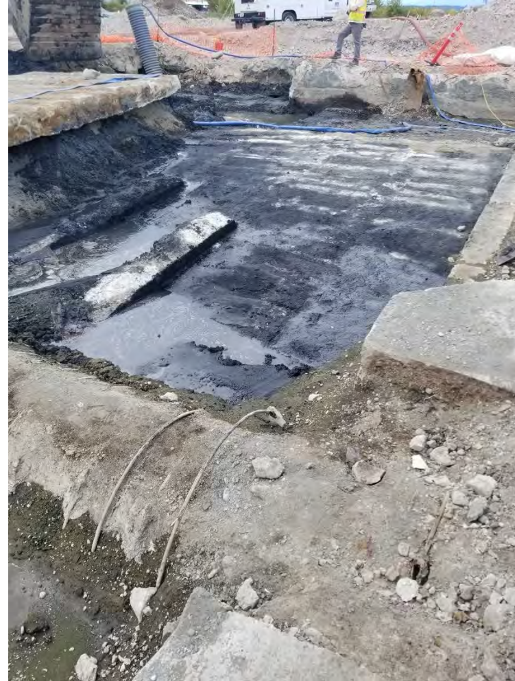
Photograph 17. Concrete slab and structures at base of CMS excavation at B-36 sample location, view looking west.
