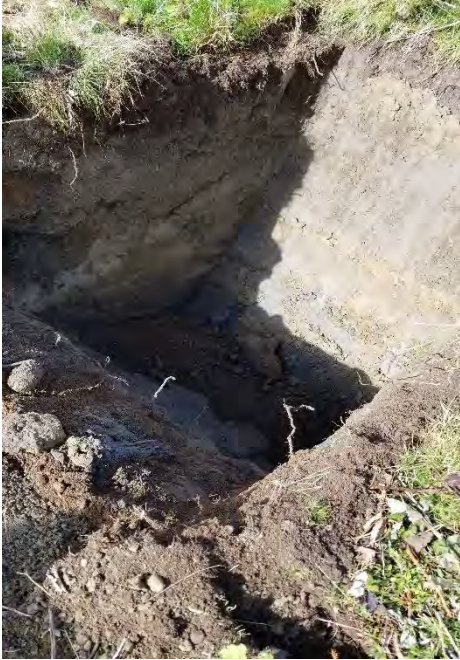
Photograph 1. Pipe P not present 7 feet east of bulkhead.
