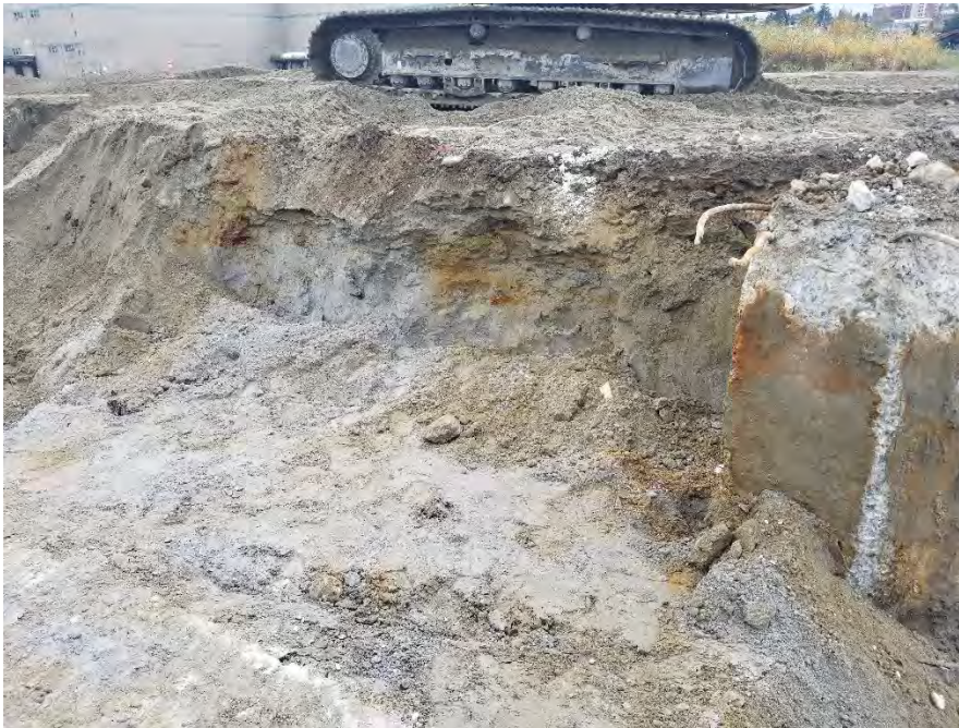
Photograph 7. South sidewall of extension between east sidewall of GFB12 Area and south leg of BBH Area, view looking south.
