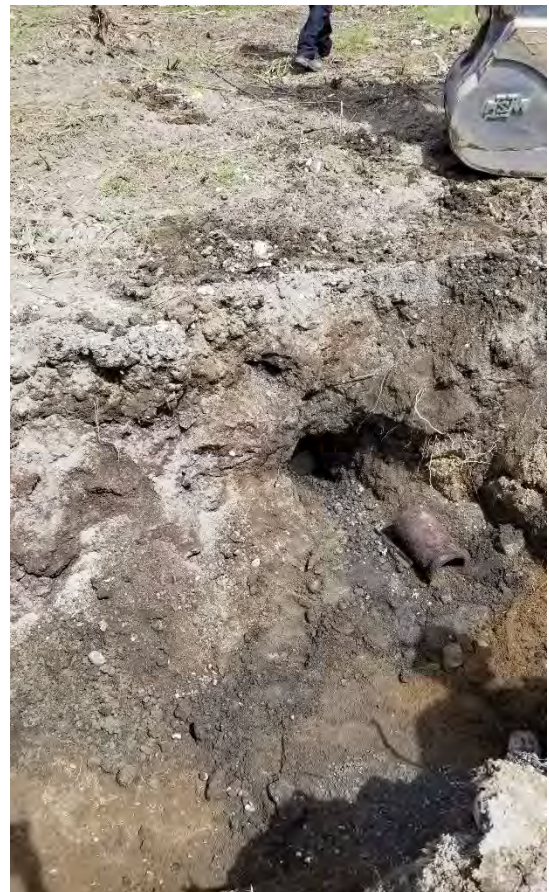
Photograph 2. B1 pipe at B2 catch basin excavation. B1 pipe was fully removed up to B2 catch basin, which was also removed.
