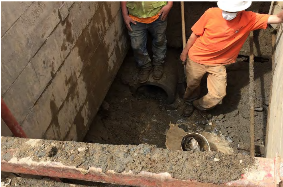
Photograph 2. Pipe K cut ~12 feet east of bulkhead, within shored excavation with active dewatering from sump. Tieback on right side was not damaged during excavation.
