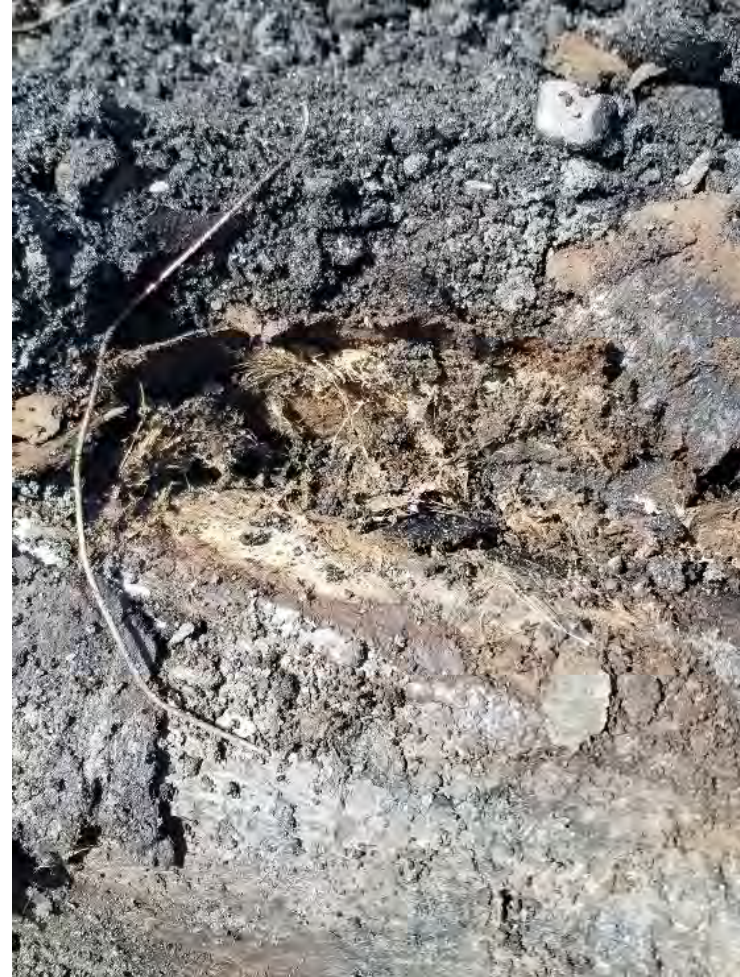
Photograph 6. Asbestos-containing material insulation on pipes.
