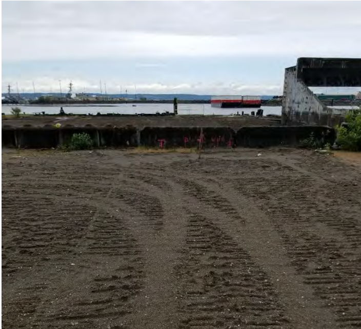
Photograph 5. Pipe K excavation backfilled, view west. A vertical 2-x-4 protruding from the backfill marks the location of the “Fernco” plug at depth.
