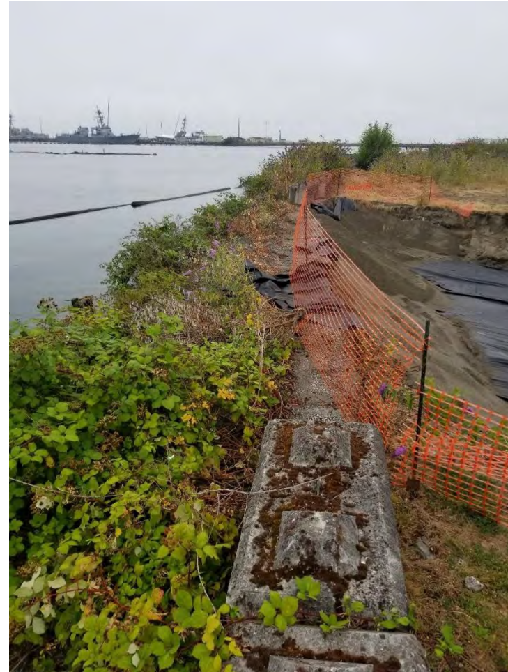
Photograph 8. Southern sidewall showing top of shoreline bank after second overexcavation, looking west.
