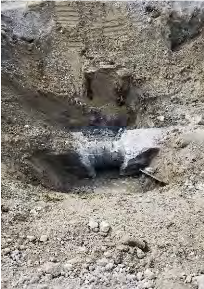
Photograph 2. Pipe M exposed 75 feet inland; concrete covering completely removed to expose wood stave pipe.
