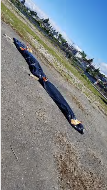
Photograph 3. Fuel oil pipe staged in visqueen pending off-site disposal.
