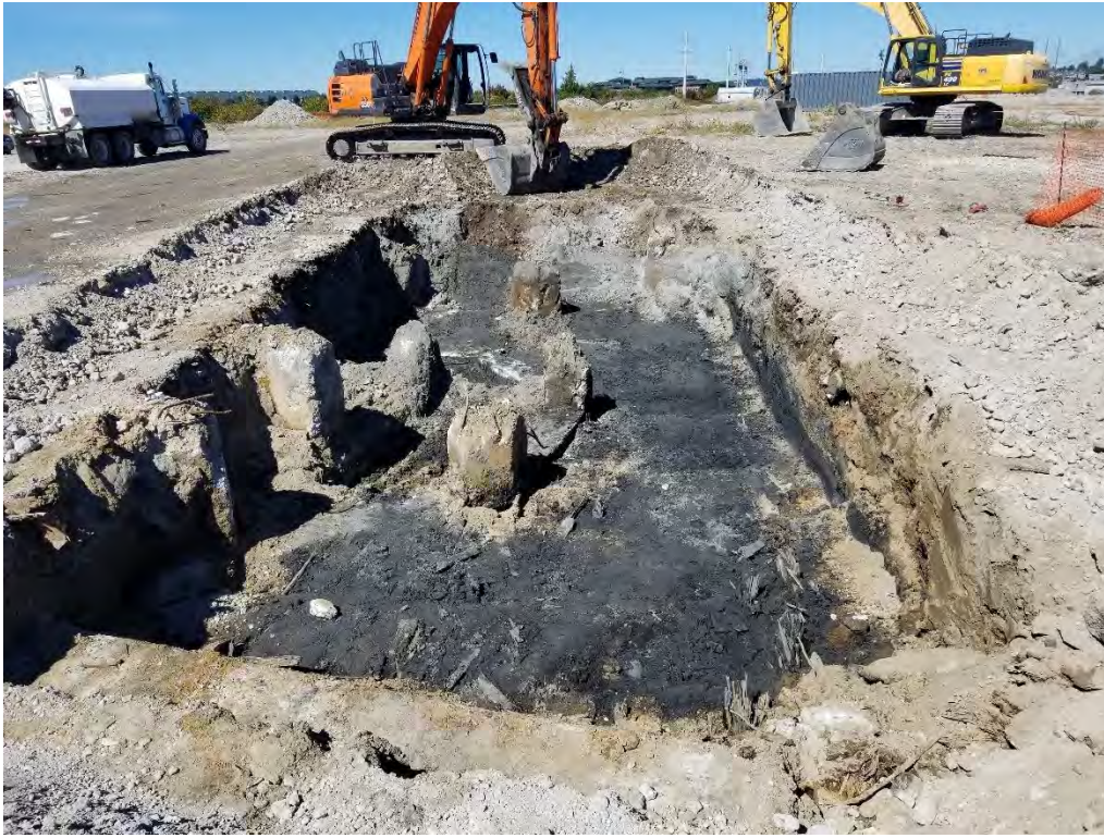
Photograph 1. Southern leg of BBH Area excavation, view looking north towards yet-to-be-excavated main excavation.
