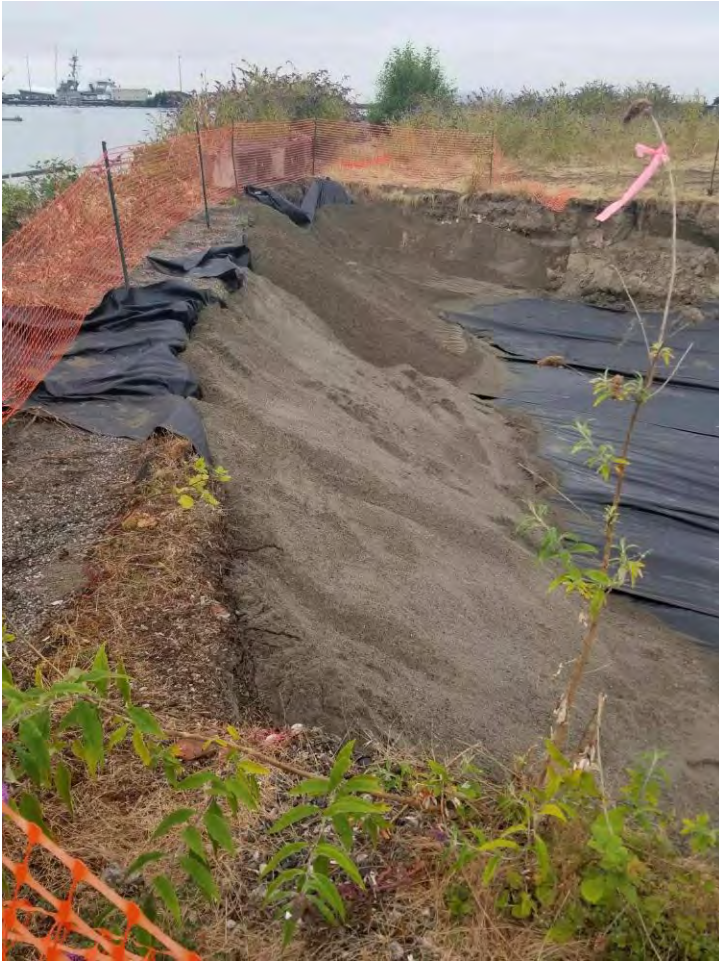
Photograph 7. Southern sidewall showing backfill placed immediately after second overexcavation to protect bank stability.
