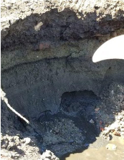
Photograph 1. South wall of excavation at 12-foot depth prior to installing dewatering sump.
