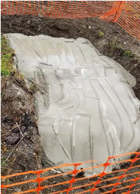
Photograph 4. Pipe B2 pipe CDF plug ~6 feet downstream of its former catch basin location.
