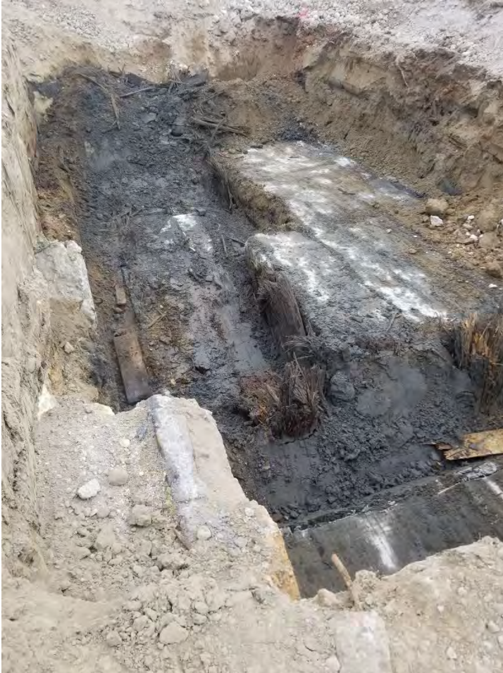
Photograph 7. Concrete slab in north sidewall of western excavation extension, beneath sidewall sample S-26 at approximately 5 feet bgs.
