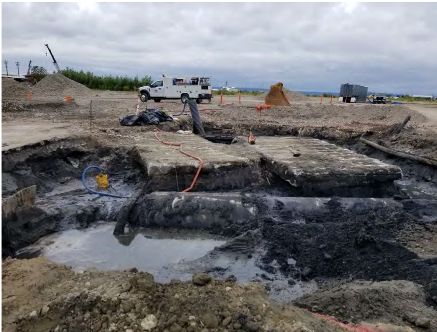
Photograph 2. South end of excavation, looking west. Concrete-encased wood stave pipe in foreground.
