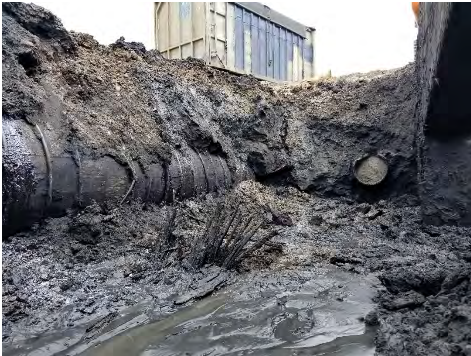
Photograph 4. North and east sidewalls on north side of concrete wall, view looking east.
