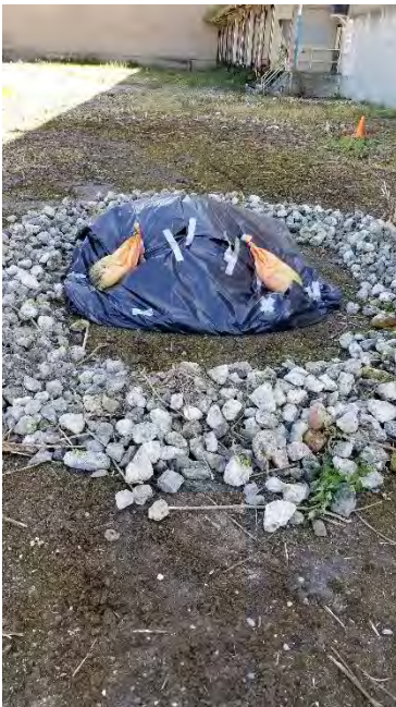
Photograph 4. Impacted soil removed from fuel oil pipe trench, stockpiled pending off-site disposal.
