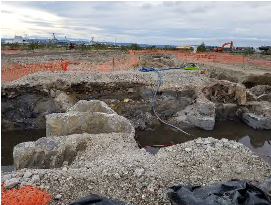
Photograph 11. Final limits of southern leg of BBH Area excavation, northern portion of west sidewall, view looking west.
