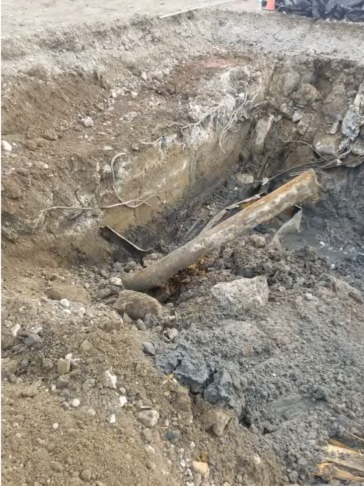
Photograph 9. Southern sidewall of main BBH Area excavation, showing concrete in upper 6 feet above sample S-67.
