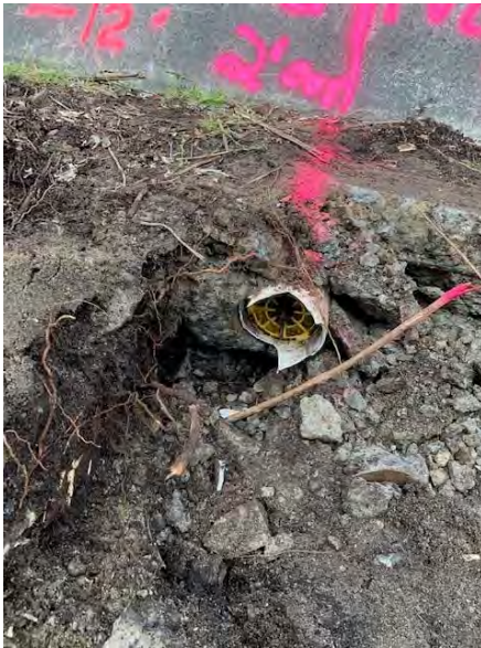
Photograph 1. Pipe L, with thermos plug installed, on west side of ecology block wall adjacent to bulkhead.
