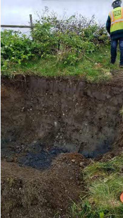
Photograph 3. Excavation for pipes Q3, Q4, and Q5, ~7 feet east of bulkhead, no pipes found.
