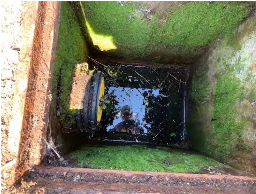
Photograph 2. Pipe H catch basin and pipe through bulkhead with thermos plug installed.
