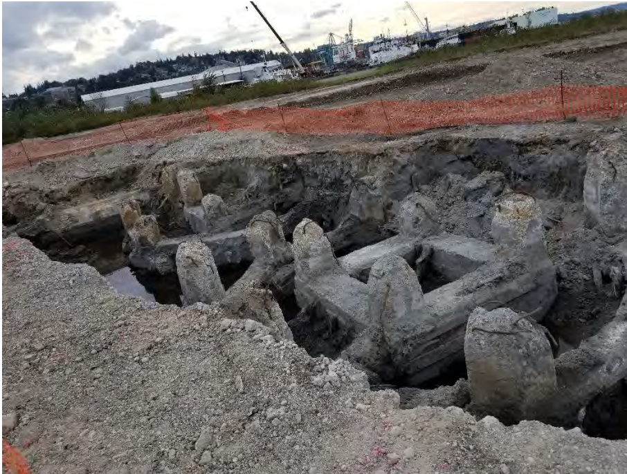
Photograph 10. Final limits of southern leg of BBH Area excavation, view looking southwest.
