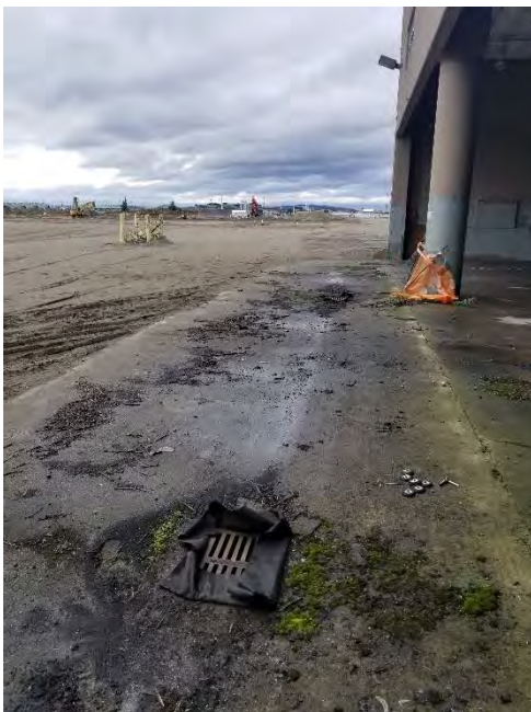
Photograph 2. Catch Basin B in foreground, Catch Basin C in background, looking north.
