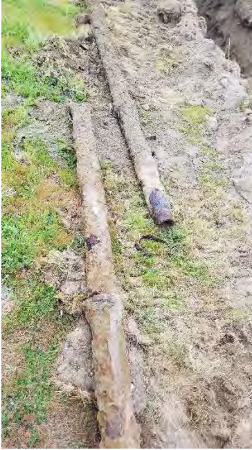
Photograph 3. Pipe G after being removed.
