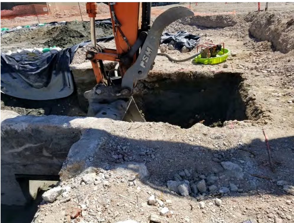
Photograph 8. Western overexcavation of west sidewall, on the south side of the concrete wall, view looking south.
