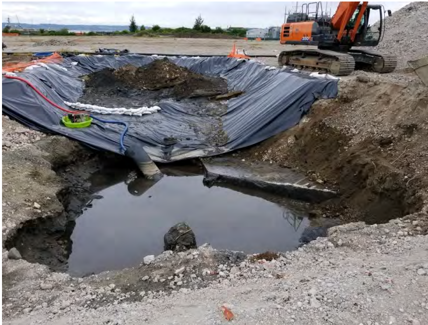
Photograph 2. Excavation after first overexcavation of north sidewall with dewatering turned off, view west. Soil on visqueen is staged awaiting loading for off-site disposal.
