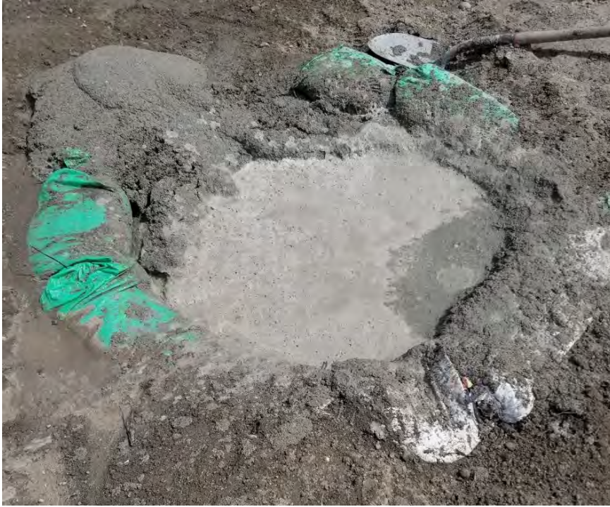
Photograph 13. Top of CDF plug at 75 feet inland. CDF plug is continuous from bulkhead to 75 feet.
