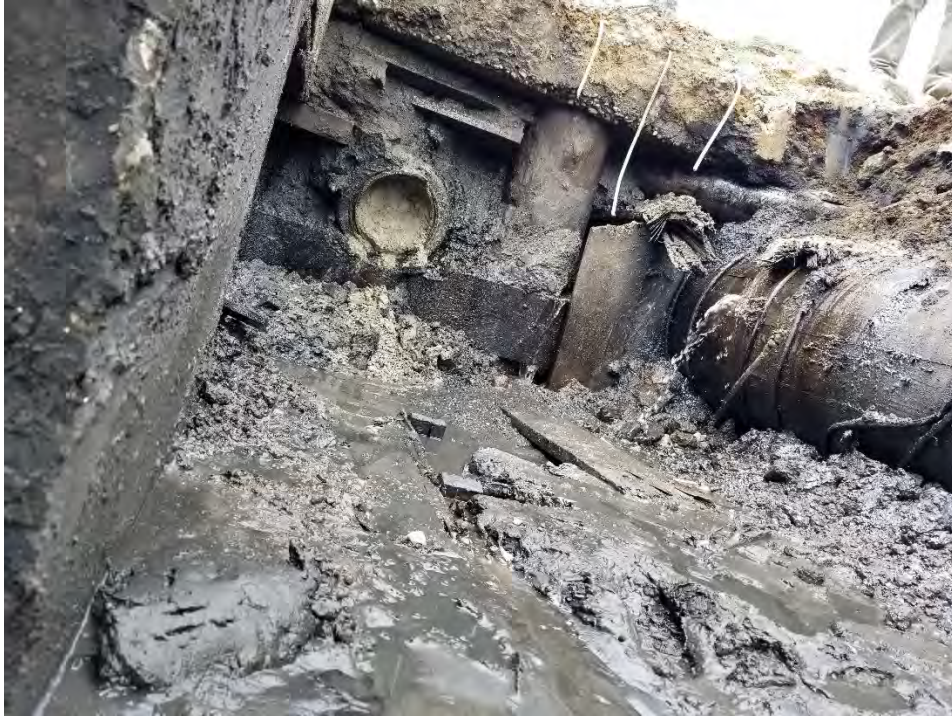
Photograph 3. Extensive structures and little soil on west sidewall north of concrete wall, view looking west.
