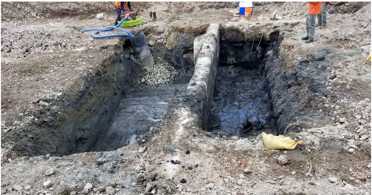
Photograph 2. Excavation showing mid-excavation concrete wall and wood stave pipe on north sidewall, view looking west.
