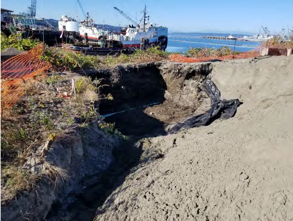
Photograph 10. Eastern corner of southern sidewall showing third overexcavation to wood stave Pipe C on 8/27/2020, looking southwest.
