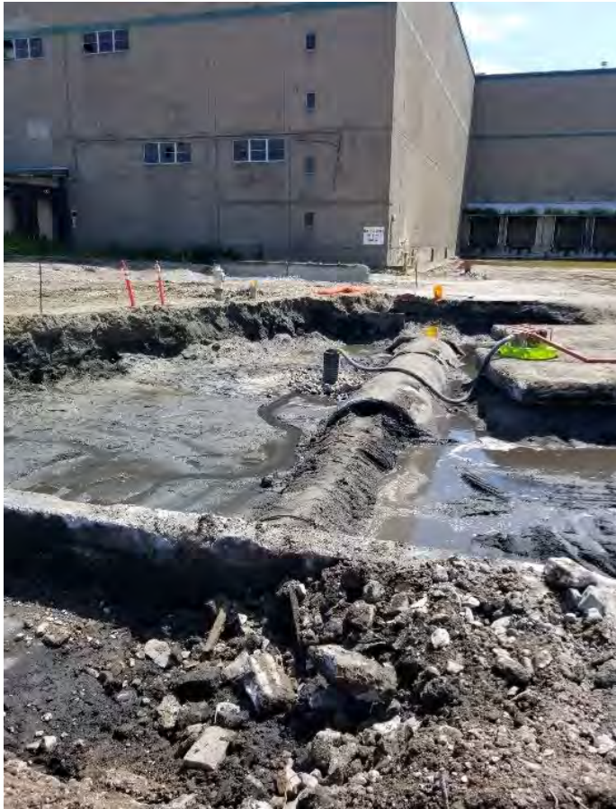
Photograph 3. Eastern side of south end of excavation, looking south. Concrete-encased wood stave pipe in center of photo, runs through/beneath east-west-trending concrete foundation structure.
