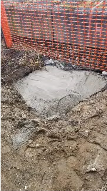
Photograph 3. Pipe H catch basin plugged with CDF.
