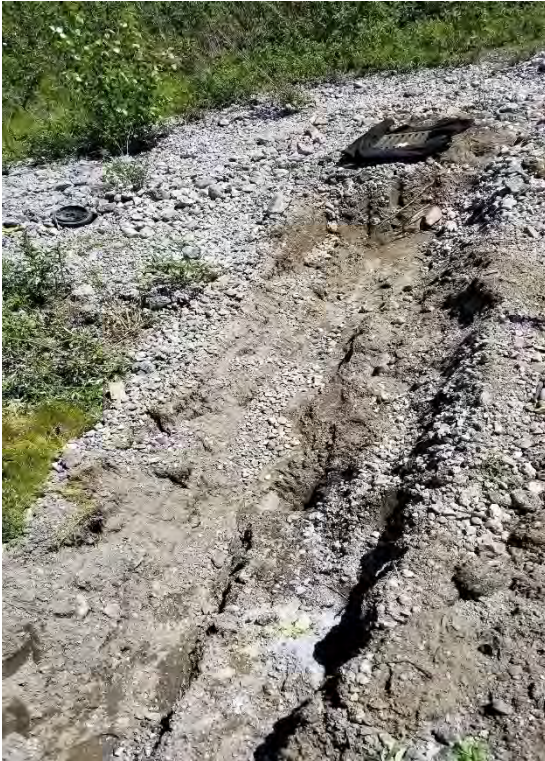
Photograph 5. B3 catch basin preexcavation. Thin veneer of CM adjacent to catch basin was removed and stockpiled.
