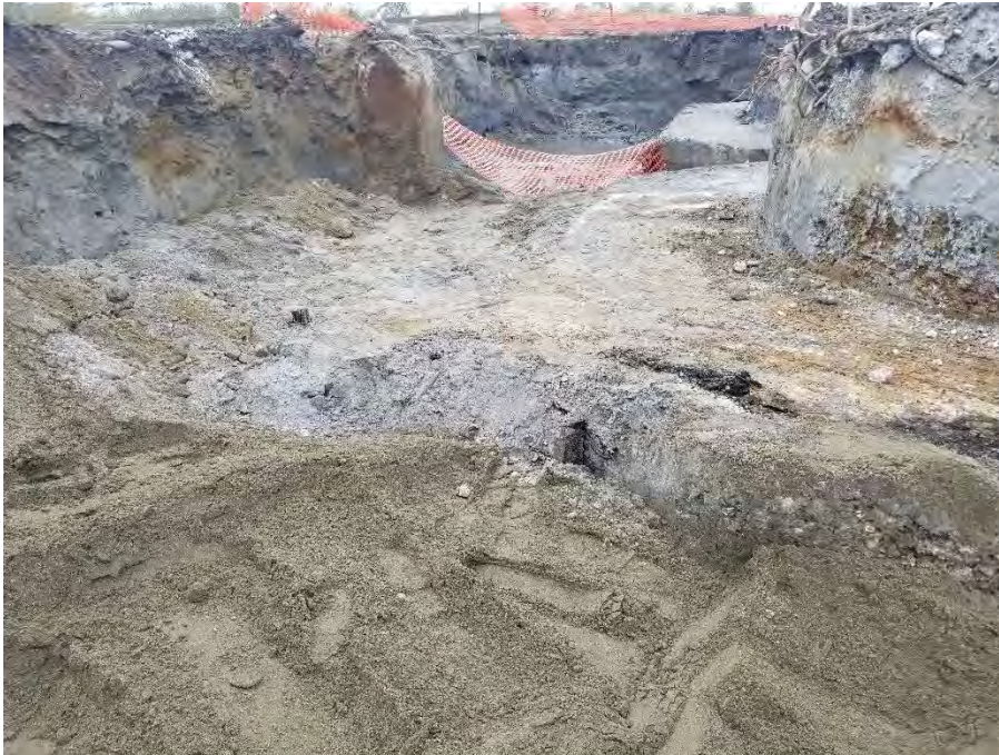
Photograph 5. Excavation extension between south leg of BBH Area (in foreground) and GFB12 Area (in background), view looking west, concrete structure comprising north sidewall evident in upper righthand corner of photo.
