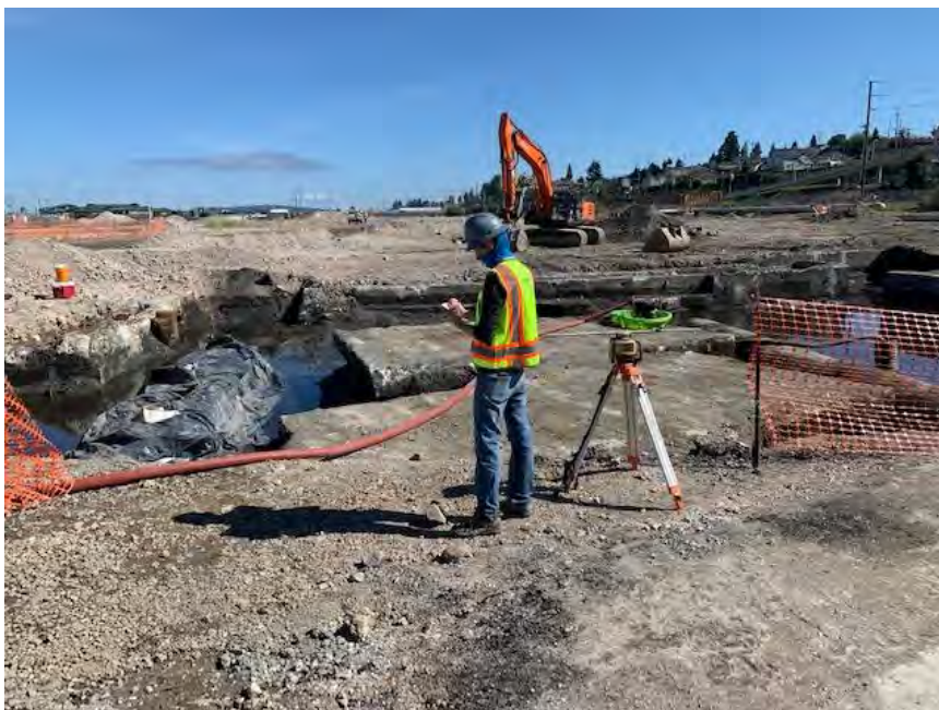
Photograph 8. Utilidor covered pending asbestos abatement (left side), dewatering in process, view north.
