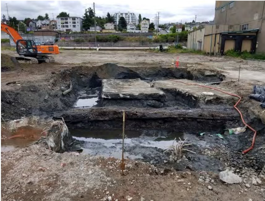
Photograph 1. South end of excavation, looking east. North-south-trending wooden utilidor on west side of concrete foundation elements.
