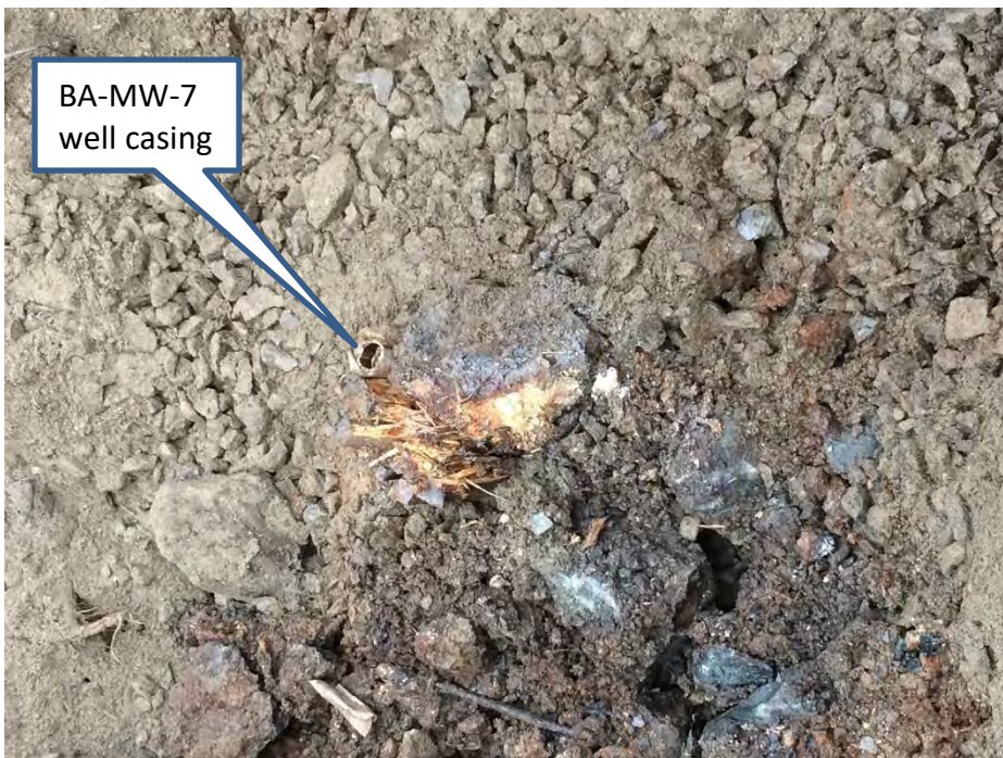
Photograph 4. Excavation bottom at ~ 9 feet, 10/12/2020. Note lower portion of BA-MW-7 well casing next to creosote-treated wood piling, quarry spalls across entire base.
