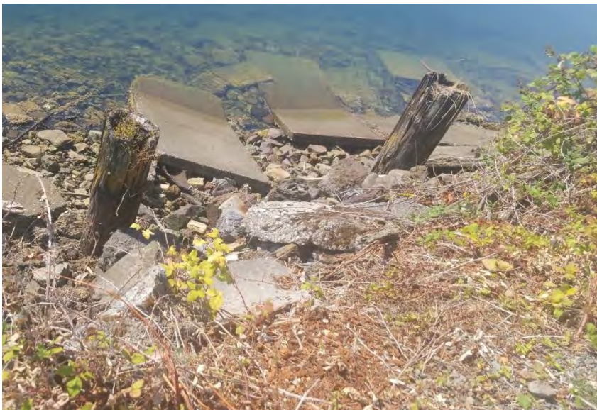
Photograph 13. Southern shoreline bank, including remnants of wooden bulkhead, after third overexcavation on 8/27/2020.
