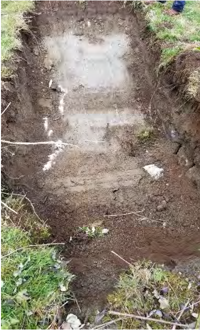
Photograph 1. Pipe N not present 7 feet east of bulkhead.
