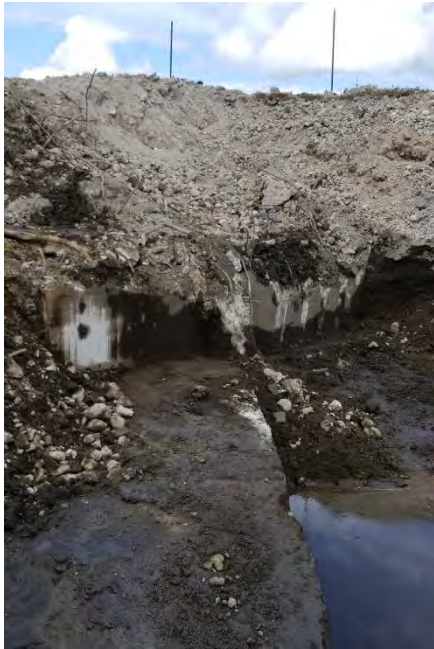
Photograph 3. East side of north sidewall of excavation after second overexcavation encounters large concrete structure.
