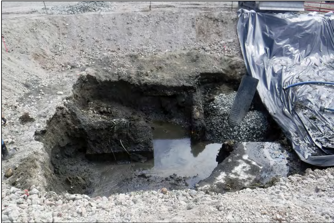
Figure 6. Photo of excavated Hydraulic Barker Area showing concrete and wood structural remains.
