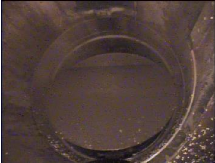
Photograph 9. Tide gate in Pipe F approx. 80 feet inland from bulkhead.
